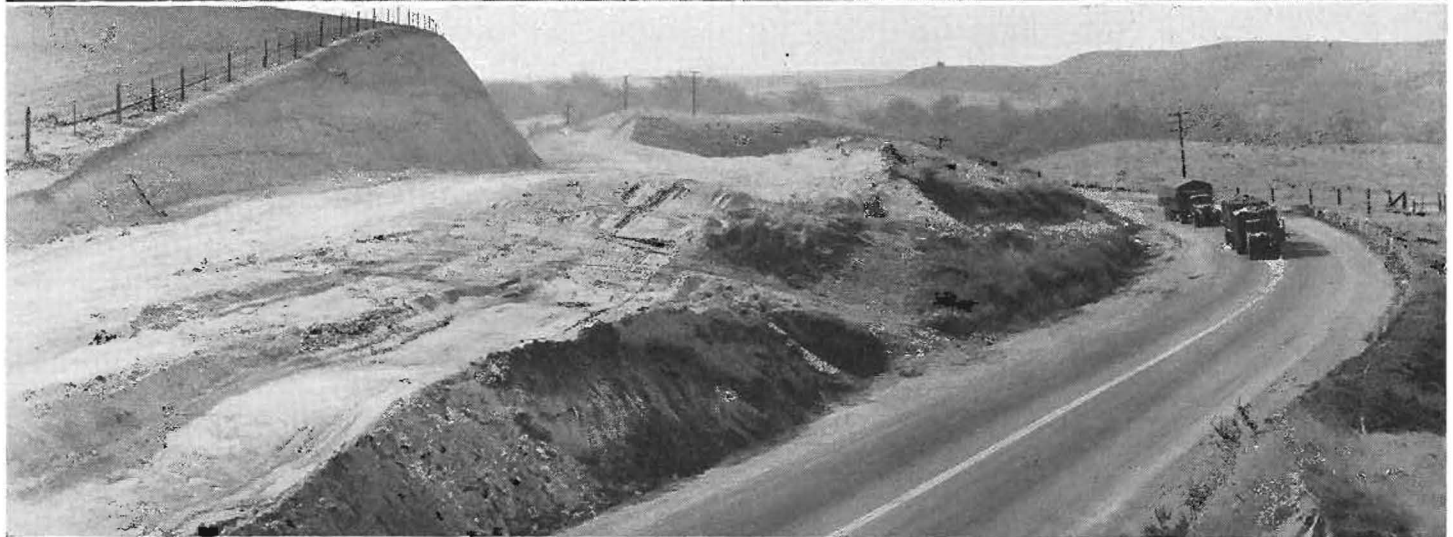
Construction scenes on Coast Highway through Malibu Ranch. Upper—Reconstruction at Encinal Canyon to eliminate reversing curves on old alignment. Center—Grading operations with modern heavy equipment to provide eighty-foot width of roadbed. Lower—Looking westerly from Walnut Canyon toward Zuma Creek, showing grading on new alignment.
