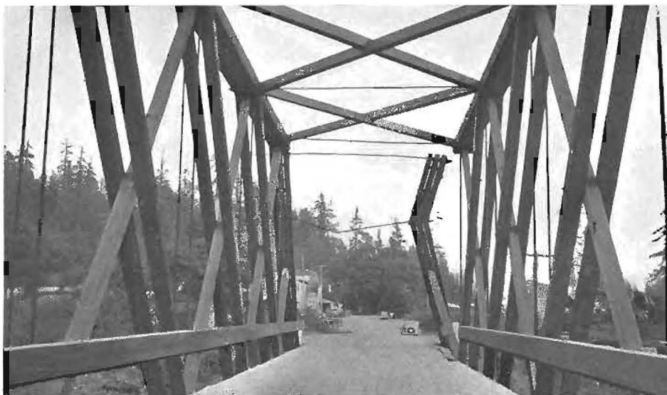
Yager Creek Bridge in Humboldt County. Note broken end post.
