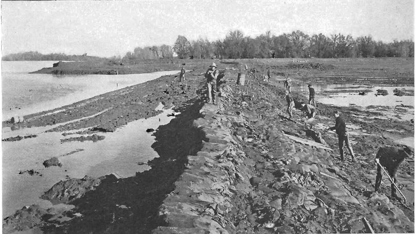
When the Sacramento River went on a rampage last December. Upper picture was taken on Phelan Ranch near Chico in Butte County and shows huge break in the Sacramento River levee and portion of hundreds of inundated acres. The lower photograph was taken at approximately the same spot after the levee closing operations had begun. The sacking job prevented overtopping of the newly built fill during later storms.
