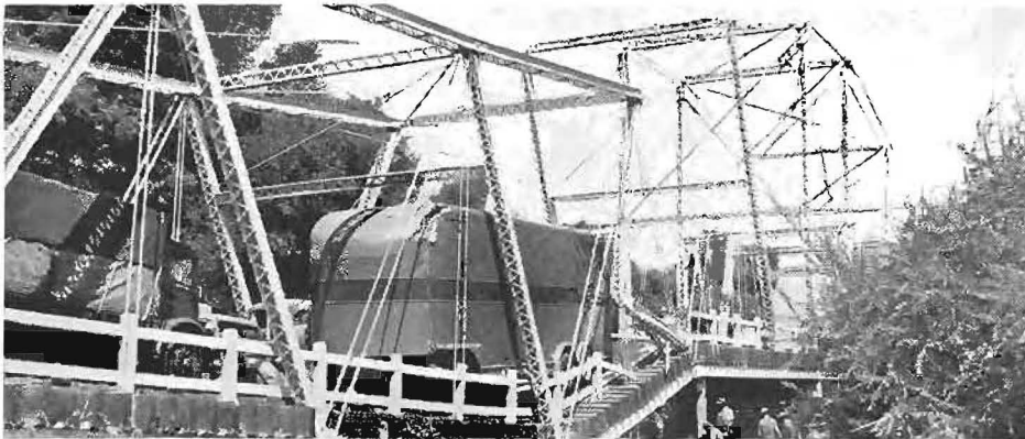
Center, overloaded truck causes collapse of San Joaquin River Bridge in Merced County.
