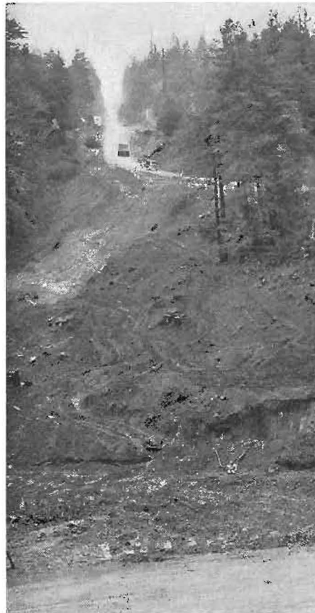
View across Mill Creek, Humboldt County, showing course of new road alignment.
