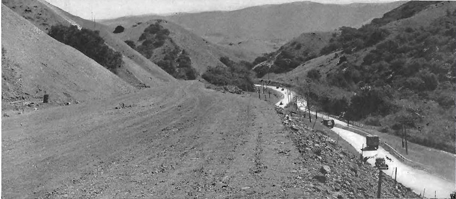
Looking south from Station 172. New Cuesta Grade construction ready for fine grading.
