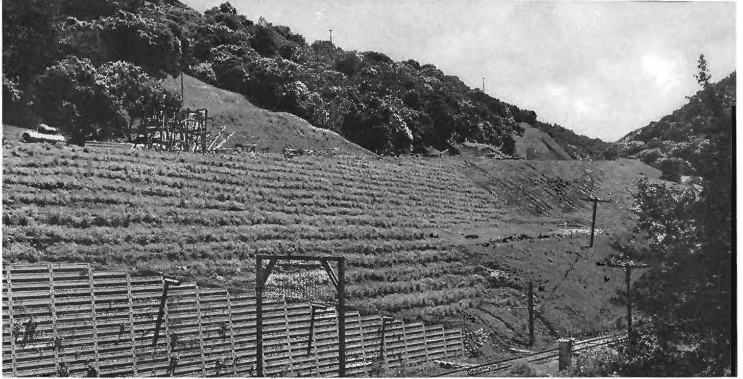
Looking south from existing Cuesta Grade. Metal crib and wattles adjacent to railroad just south of overhead.
