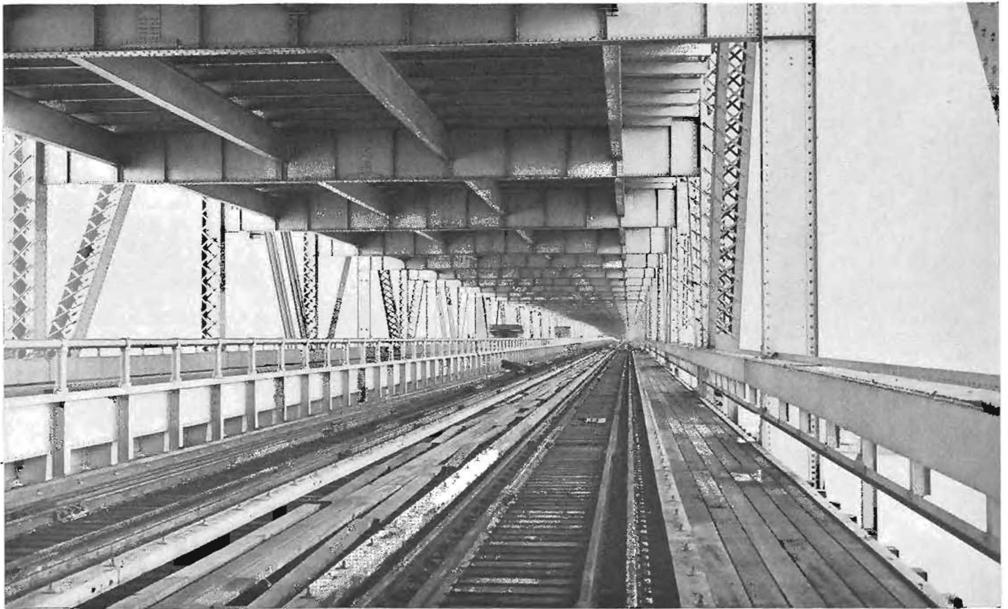
This view looking down the East Bay Crossing shows ties and tracks in place.
