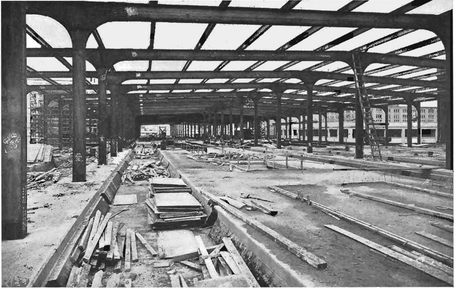
Trains will roll in the San Francisco Terminal over six tracks arranged in pairs. This view of the elevated track level also shows the roof steel just erected.
