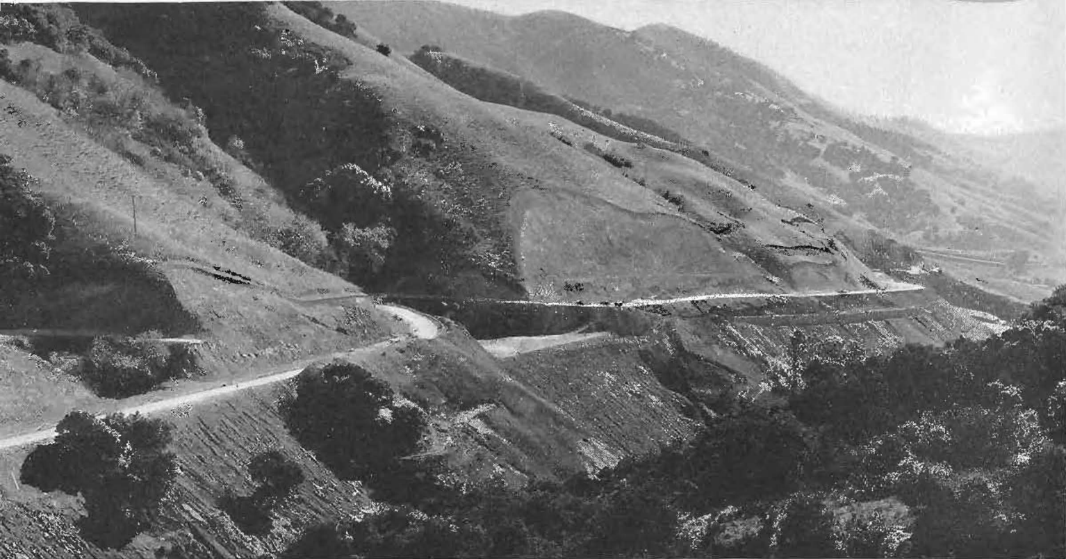
Here is an excellent view of one of many Cuesta grade curves now being eliminated.
