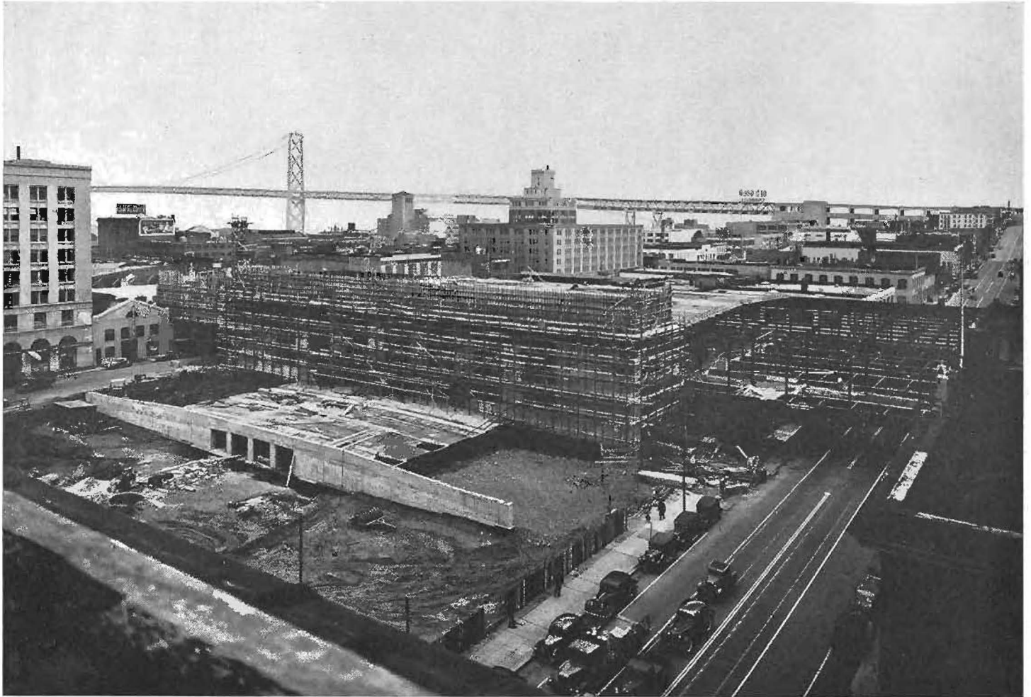
The San Francisco Terminal, facing Mission Street, showing the center unit well under construction. Street car ramp in the foreground. East and west units not visible.
