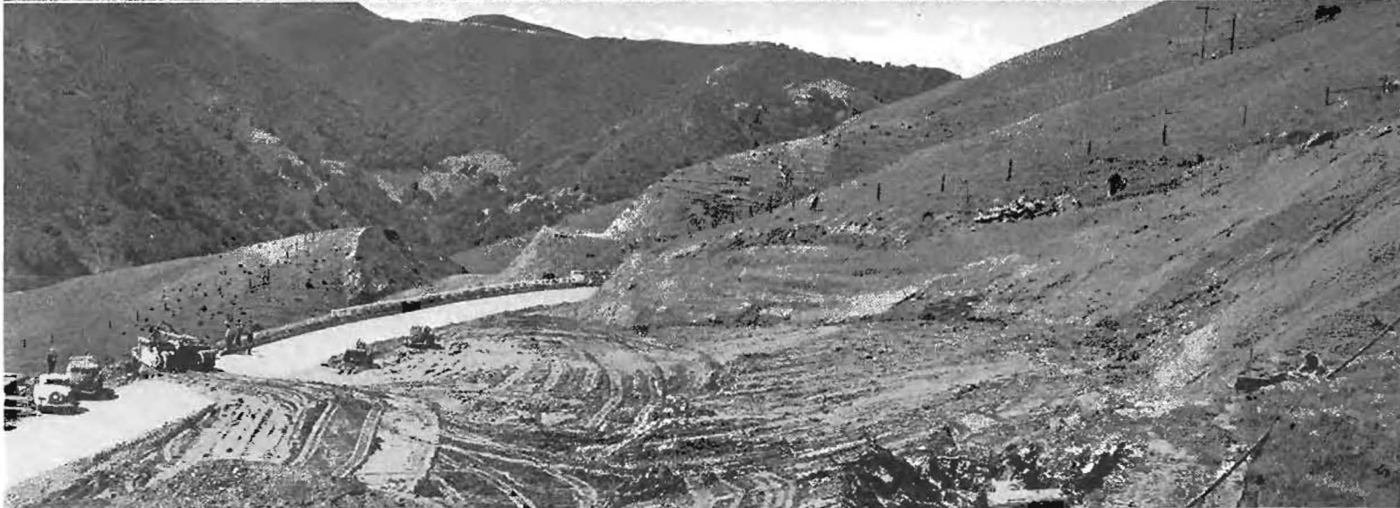
Construction scenes on Cuesta Grade. Upper—Looking south from Station 216. Note slide in upper left with roadbed cut below. Center—Heavy grading equipment in operation. Lower—Unloading top of slide at Station 210. Grade of finished road is 25 feet below existing road. This project presented Division of Highway engineers with many backfilling, cribbing and fill treatment problems.
