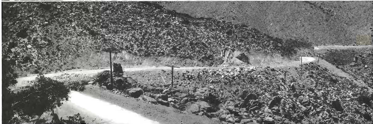
A novel ground-breaking ceremony was witnessed on the Mountain Springs grade relocation of U. S. 80 in Imperial County when Governor Merriam started the work by setting off a dynamite blast. In the official group, left to right, are: T. L. Richards, George Burnham, E. E. Cavanagh, Clarence Walker, H. R. Judah, Col. Ed. Fletcher, Governor Merriam, Frank G. Forward, L. G. Bradley and Edward I. Neron. The bottom picture shows a section of this narrow winding highway across the mountains between Imperial and San Diego Counties.
