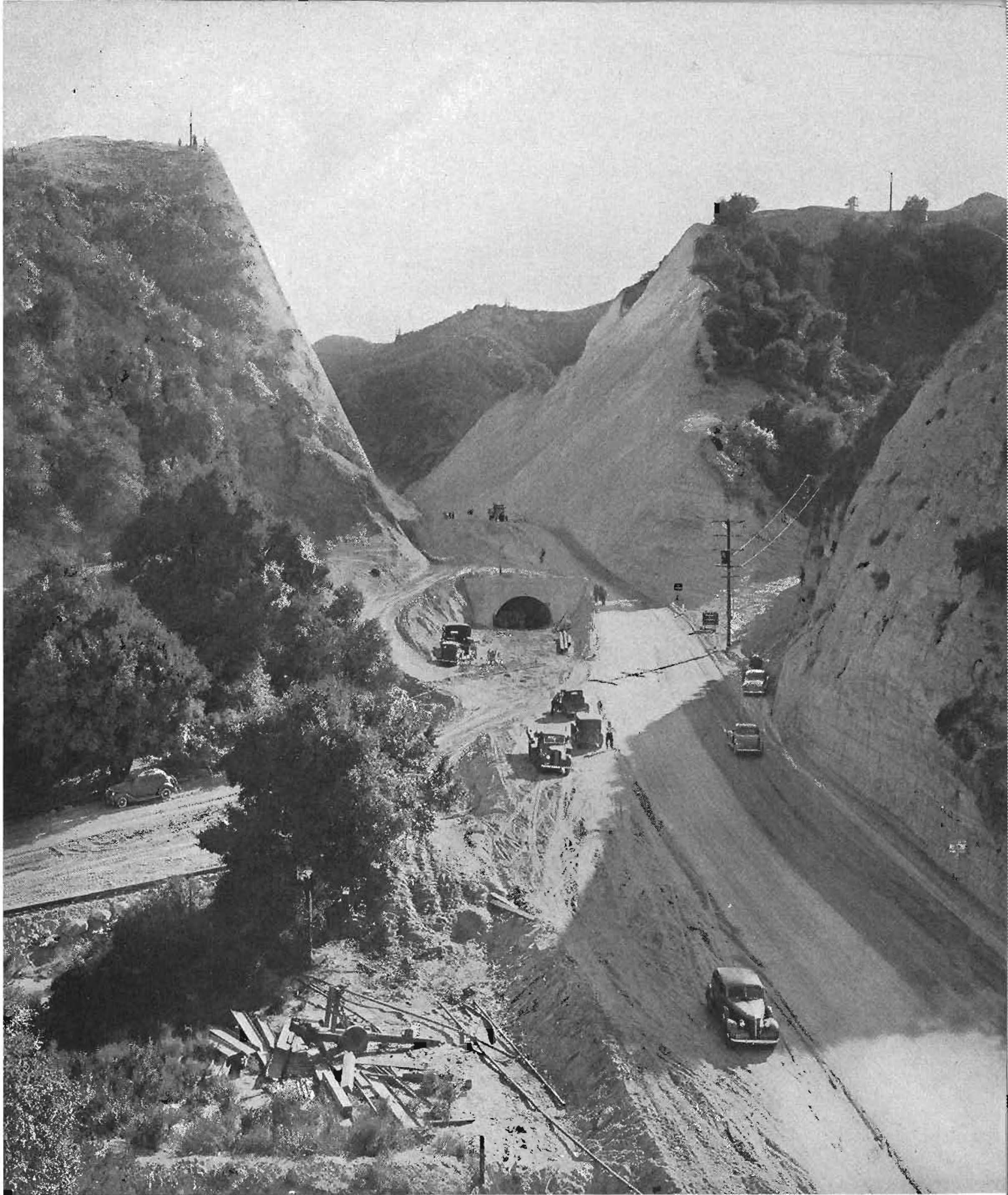
Newhall tunnel cut as it appeared with mountain slopes excavated permitting traffic to proceed beside and over the old bore.
