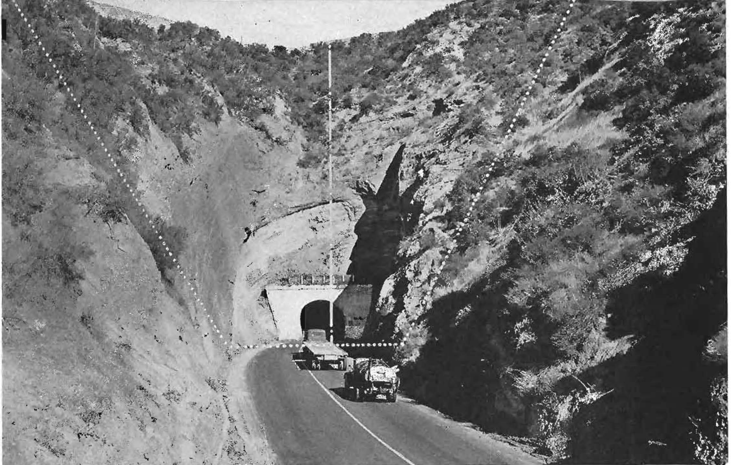
Narrow Newhall tunnel through Santa Susana Mountains is being transformed into open cut as indicated by dotted line.
