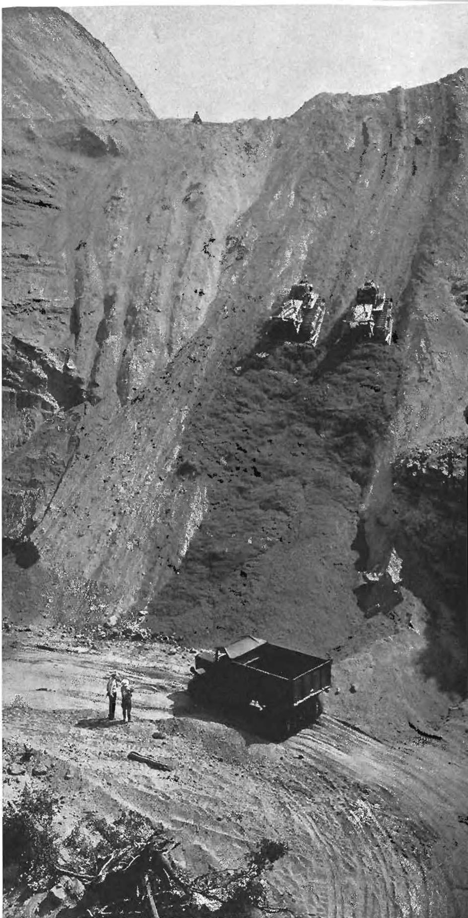
Newhall cut involved about 300,000 cubic yards of excavation. Tractors pushing dirt down for removal by shovel and truck.
