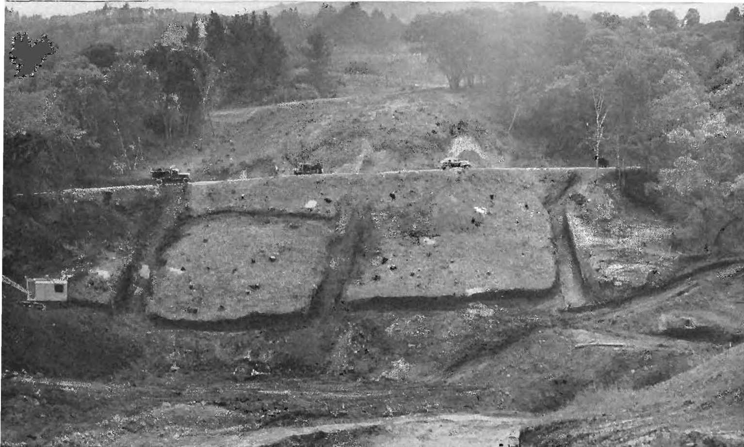
Extensive deep trenching for rock filling in drainage system made necessary to insure stability of big fill on realignment in Santa Cruz Mountains.
