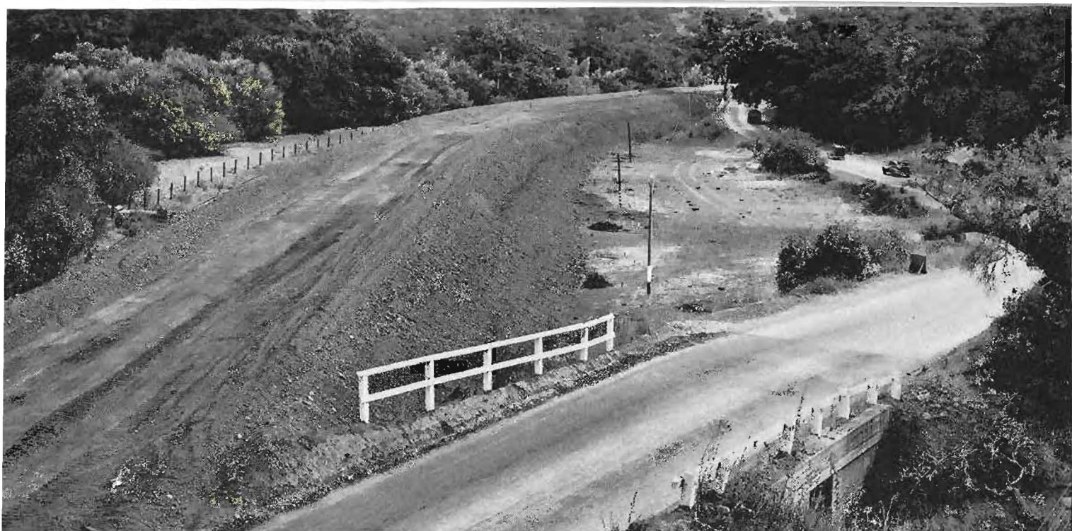
New highway sector in Nojoqui Valley with gradual grade and easier curves cuts out many sharp turns and shortens distance.
