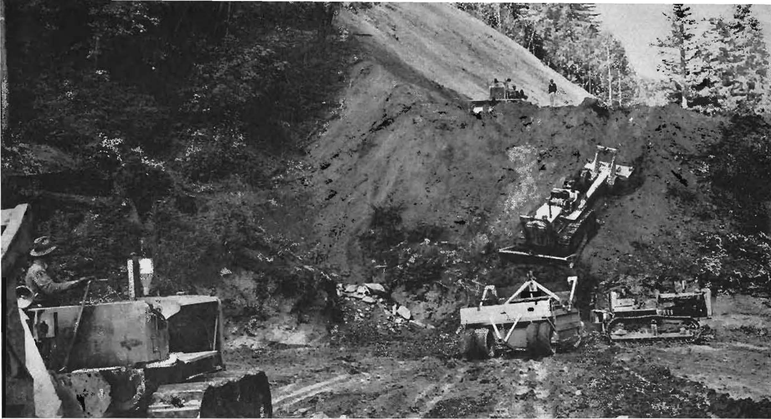
Heavy grading work under way on Los Gatos-Santa Cruz realignment. Approximately 2,300,000 cubic yards of dirt will be moved.
