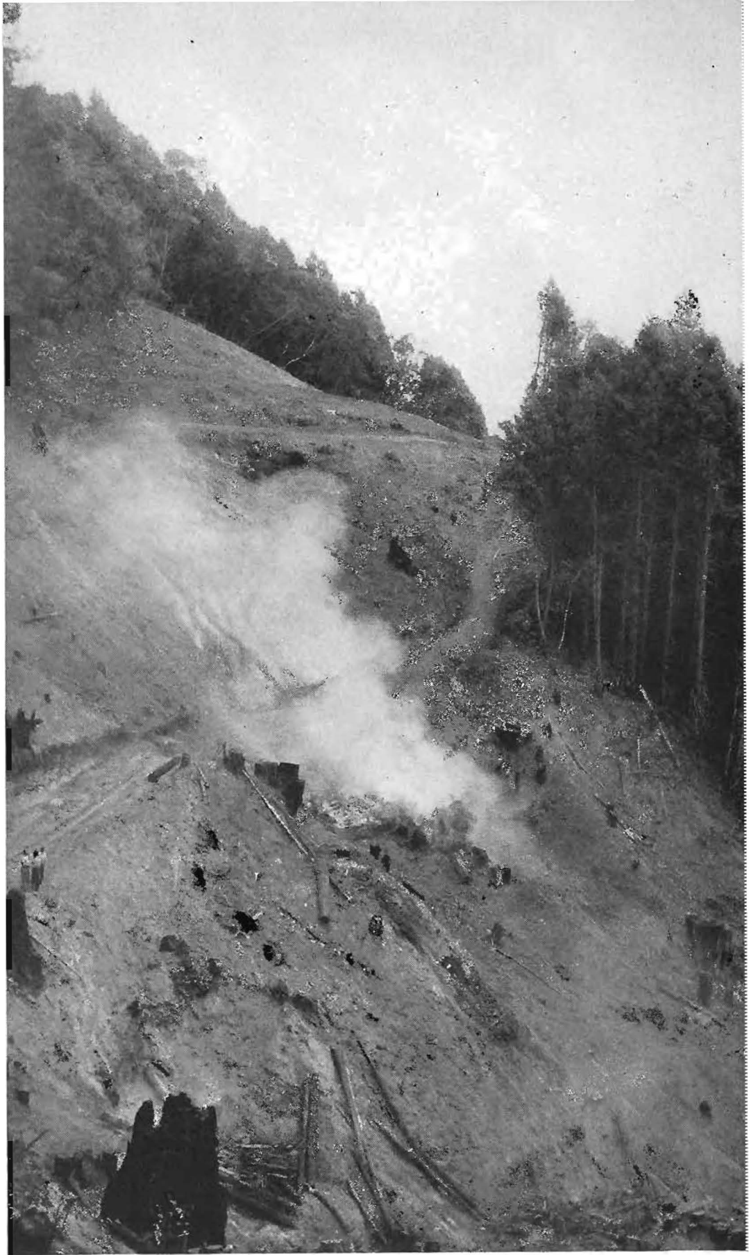
Mountainous area and geologic conditions of Los Gatos-Santa Cruz realignment present many fill and drainage problems. Picture shows clearing operations for large fill across deep ravine on new route which crosses line of existing highway seen near top of photograph.
