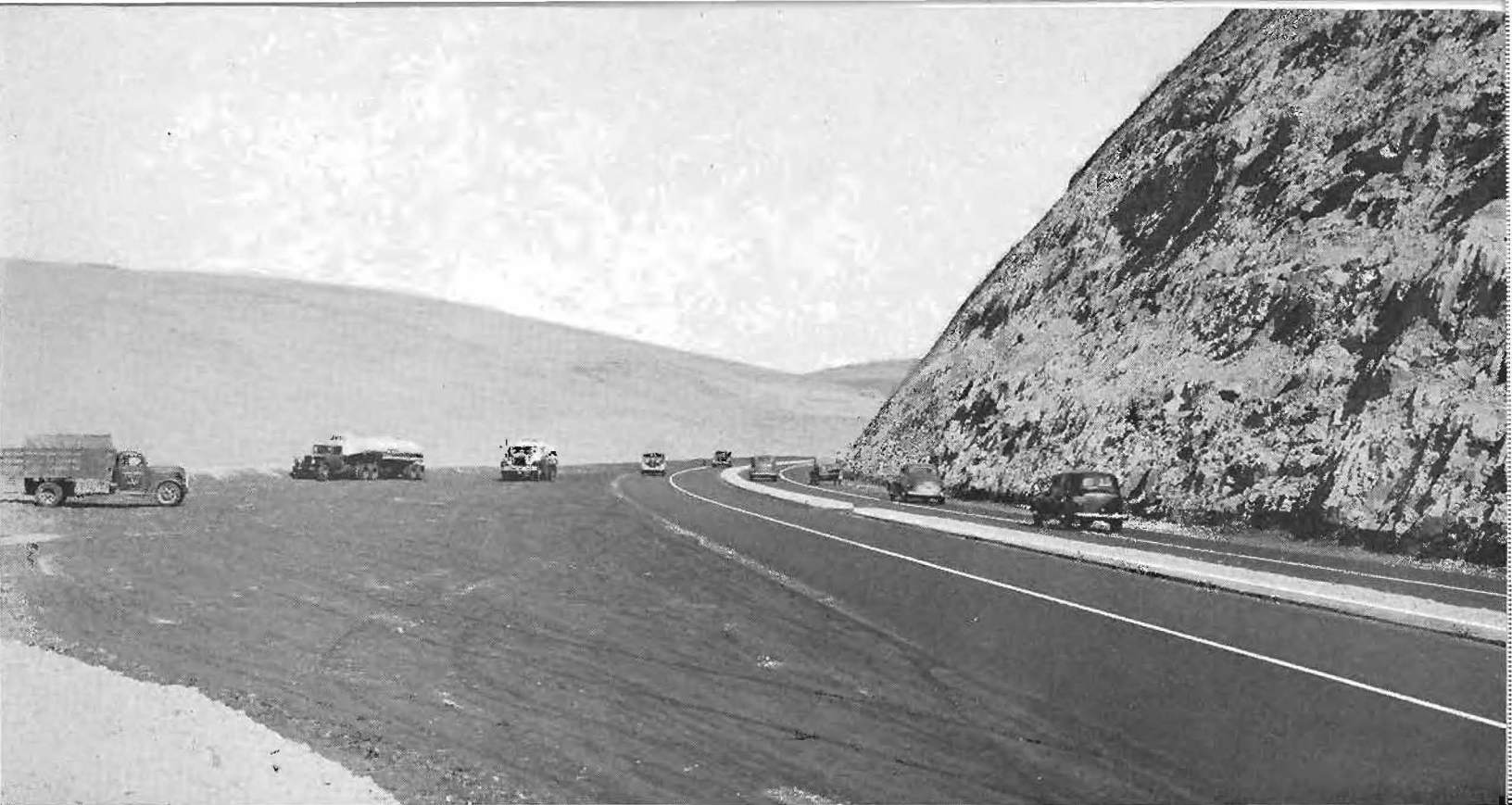
Wide parking areas are provided on the realigned Altamont Pass Highway. Heavy rock cut on right is nearly 100 feet high.
