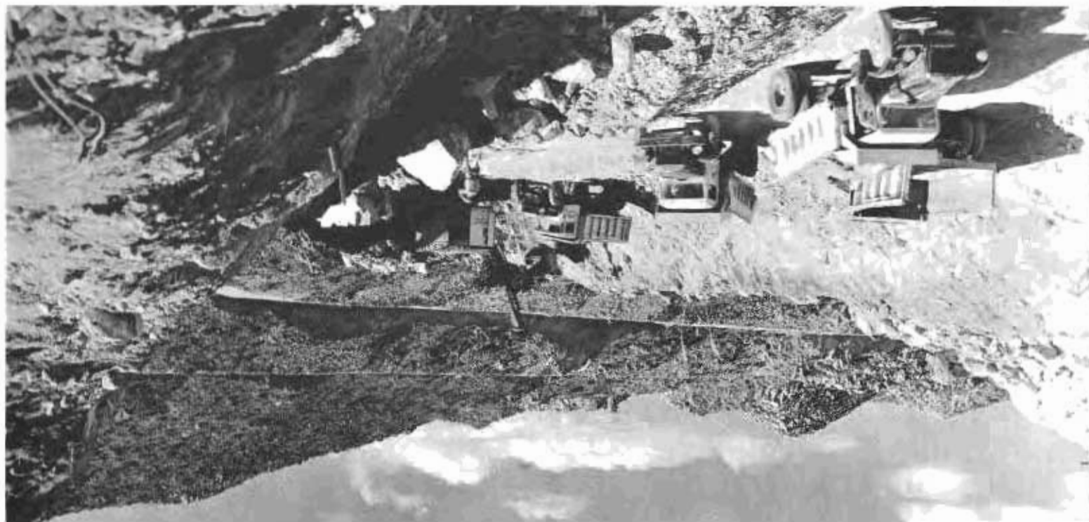
Shovels and heavy trucks working on excavation of new Mountain Springs grade. Old grade and look-out tower seen in background.
