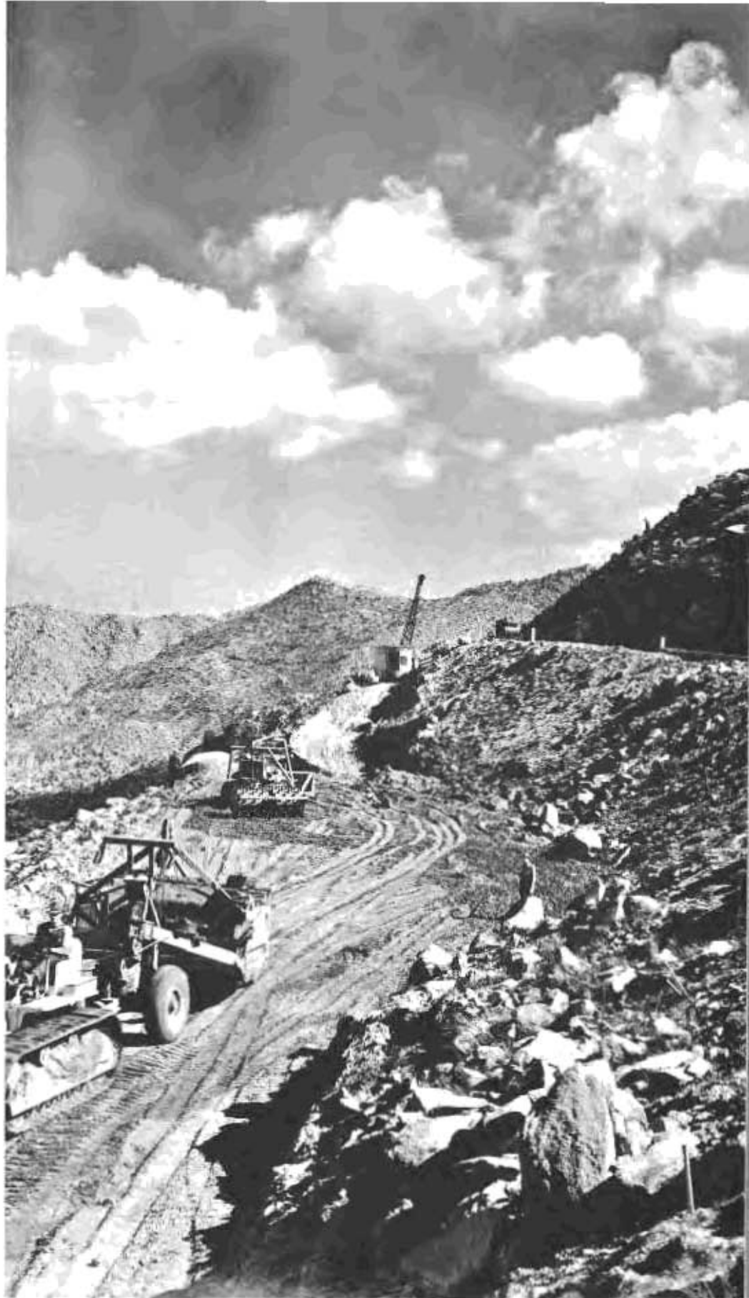
Construction scene on Mountain Springs grade relocation involving excavation of approximately 100,000 cubic yards per mile, mostly granite rock. 13,000,000 gallons of water will be required in consolidating this rock into embankment sections.
