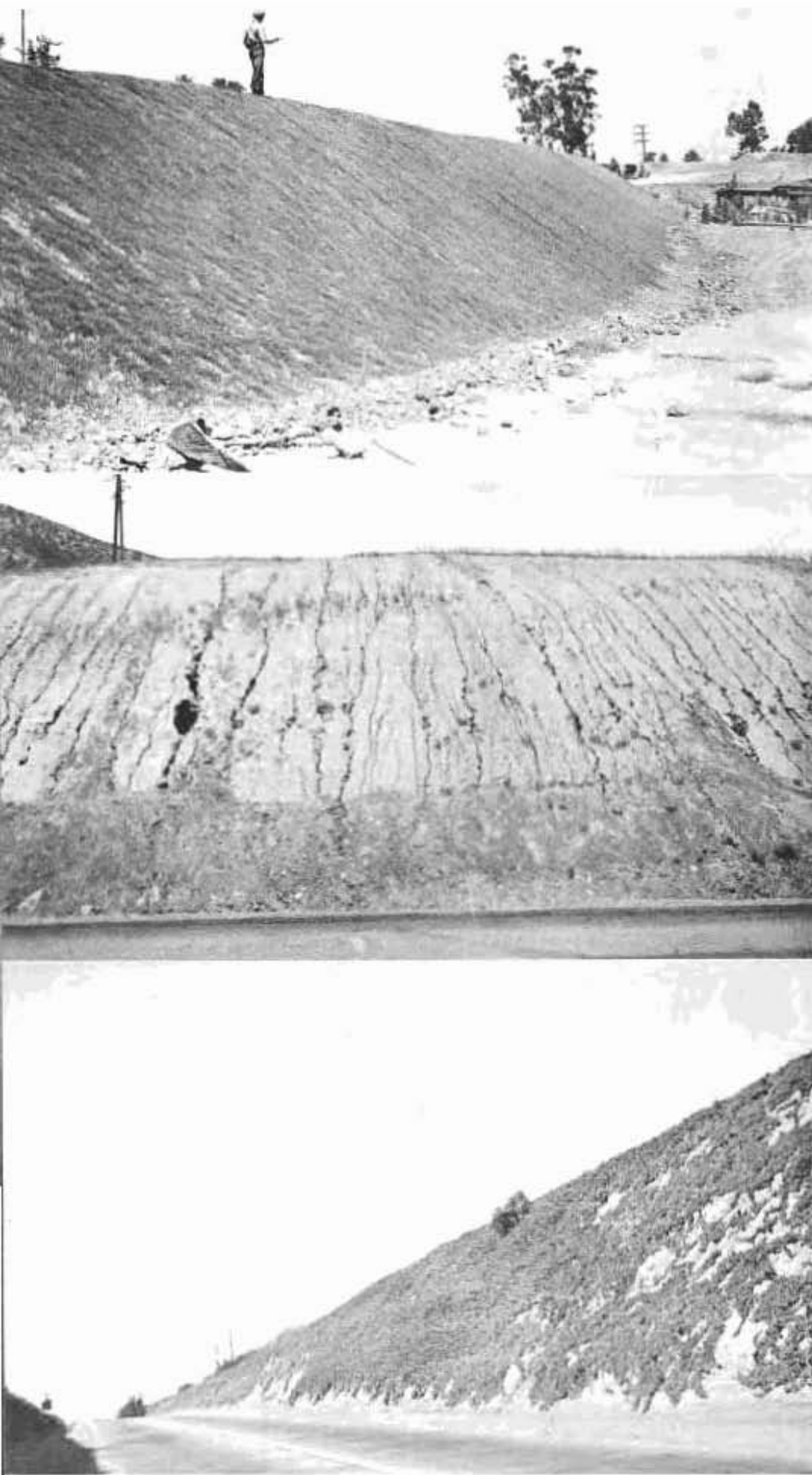
New cut slopes on the Arroyo Seco Parkway in Los Angeles are grass seeded immediately to get a coverage protection against erosion by early rains. Center—One rain, the first of the season produced this extensive bank erosion. Bottom—Ice plant is protecting this previously badly eroded slope in Solomon canyon.
