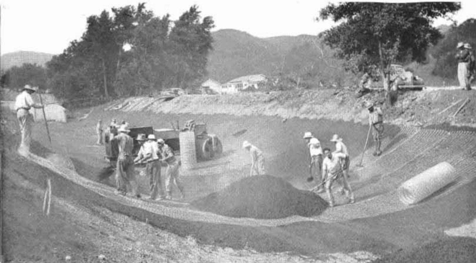
Placing reinforced concrete channel lining on Santa Clara River near Saugus in Los Angeles County.
