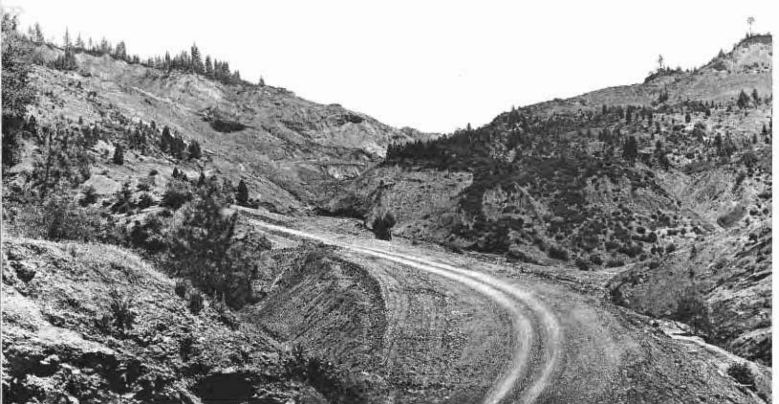
Partially graded highway approaching hydraulic cut through Oregon Mountain from west. The cut is 2000 feet wide, 2500 feet long, 210 feet deep at top.
