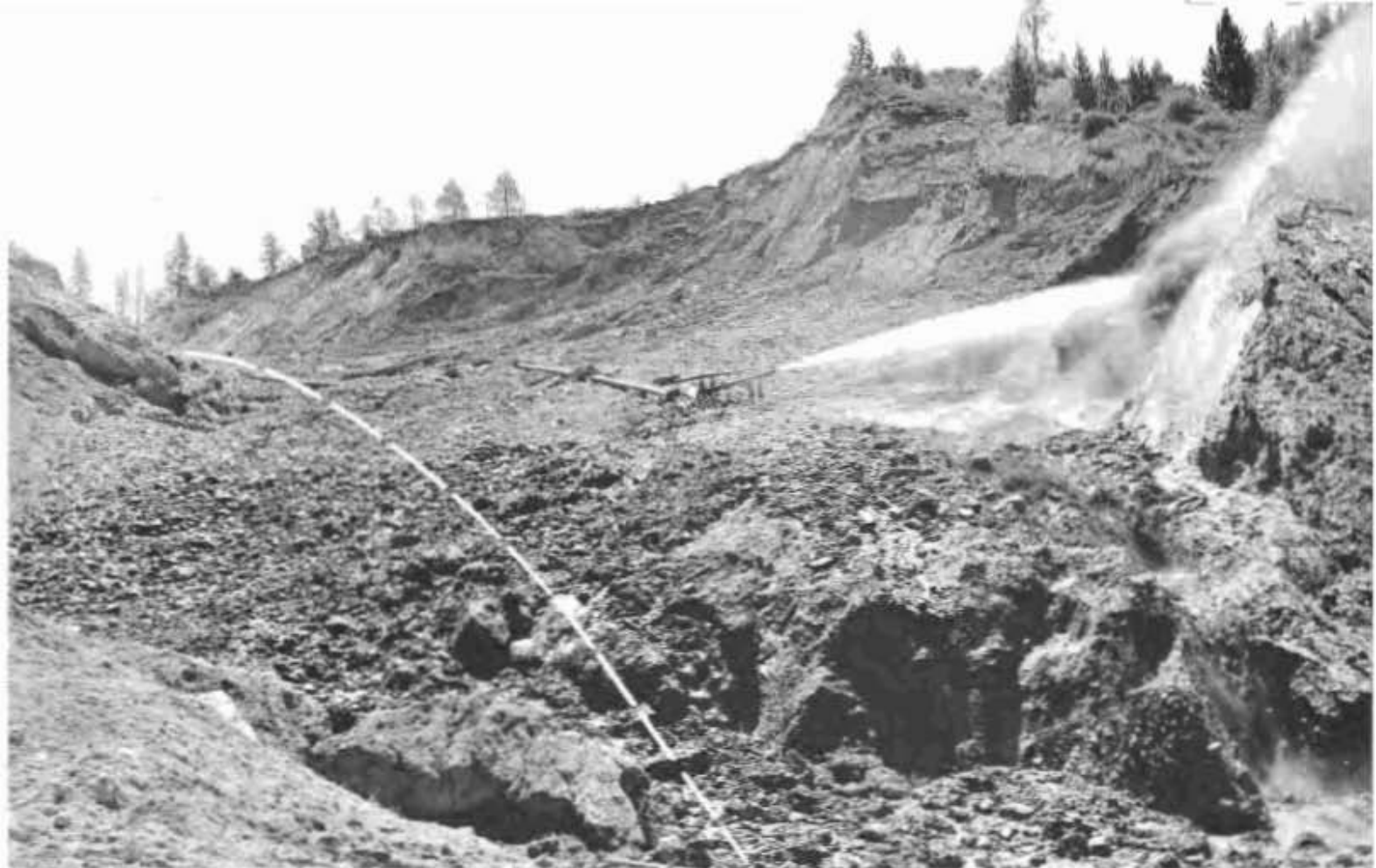
View of hydraulic giant working on highway excavation in Oregon Gulch. White dash line shows highway grade through cut at summit.
