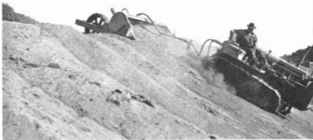
Blanketing a sandy slope with top soil spread from above with tractor equipment.
