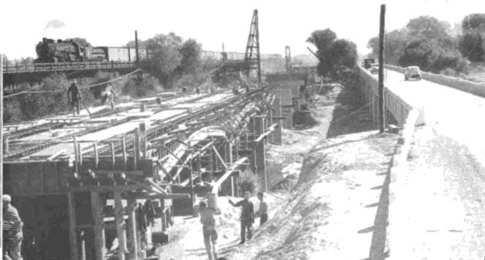
Constructing reinforced concrete bridge across Kings River near Kingsburg, Fresno County, to carry northbound traffic of proposed 4-lane divided section of U. S. 99.
