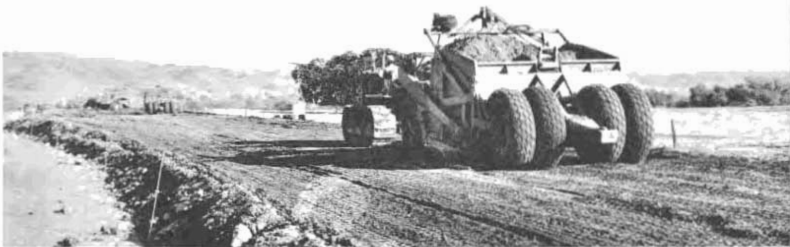
Construction scenes on realignment of U. S. 101 near Bradley, Monterey County, showing tractor and 28 cubic yard scrapers at work. Center—Narrow old bridge across Salinas River to be replaced and section of existing 15-foot concrete pavement laid in 1910.
