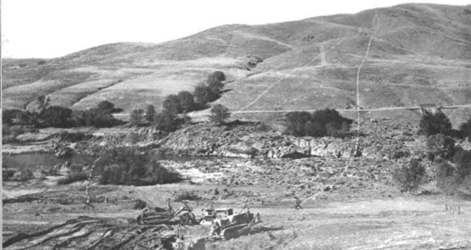
View of Friant Dam site looking across San Joaquin River toward right abutment. White lines indicate excavation area for dam foundations.
