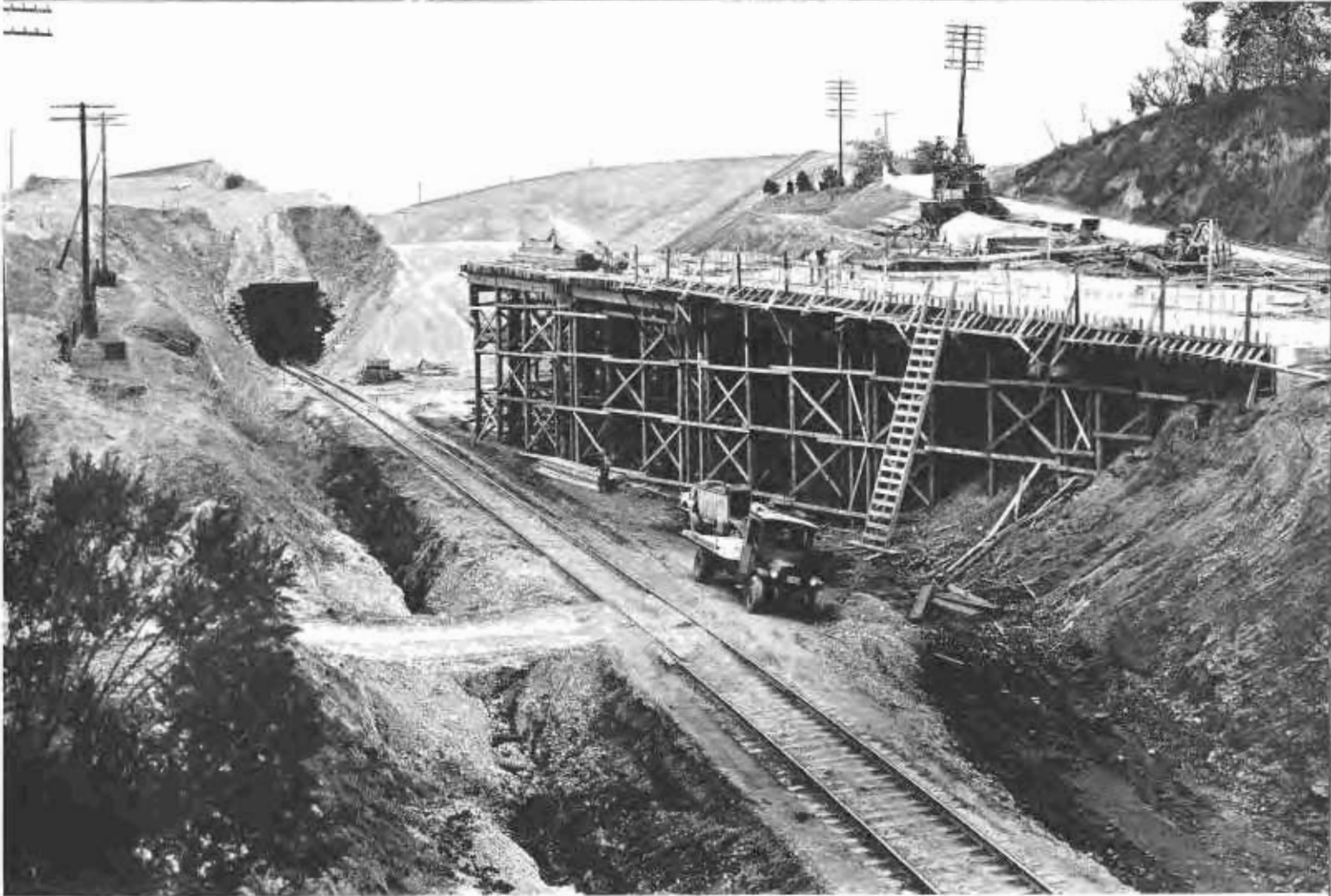
Two views of extensive operations involved in realignment near Pinole of a link of U. S. 40 carrying heavy traffic between San Francisco and Sacramento, owing to the abandonment of a tunnel by the Santa Fe Railroad and relocation of route in an open cut. The existing highway crosses over the top of the tunnel. Its realignment on a straighter line will cross the railroad cut on a bridge. Upper photo shows highway detour and bridge operations without halting train or motor traffic. Below—Bridge construction near tunnel. New tracks will swing under this section of bridge permitting other half to be built.
