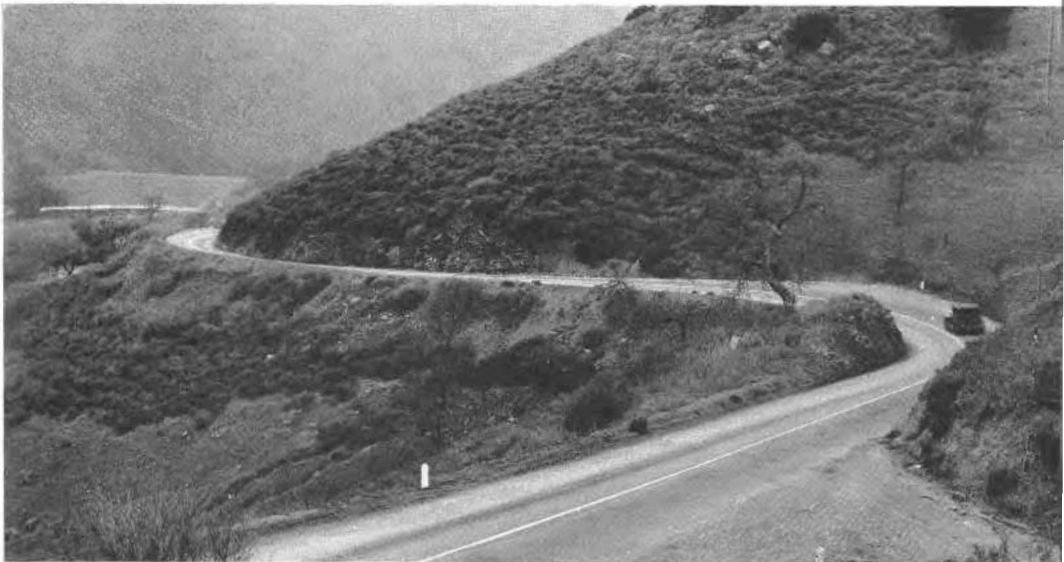
Several of the thirty-one sharp curves on Pacheco Pass mountain highway being eliminated by realignment project.
