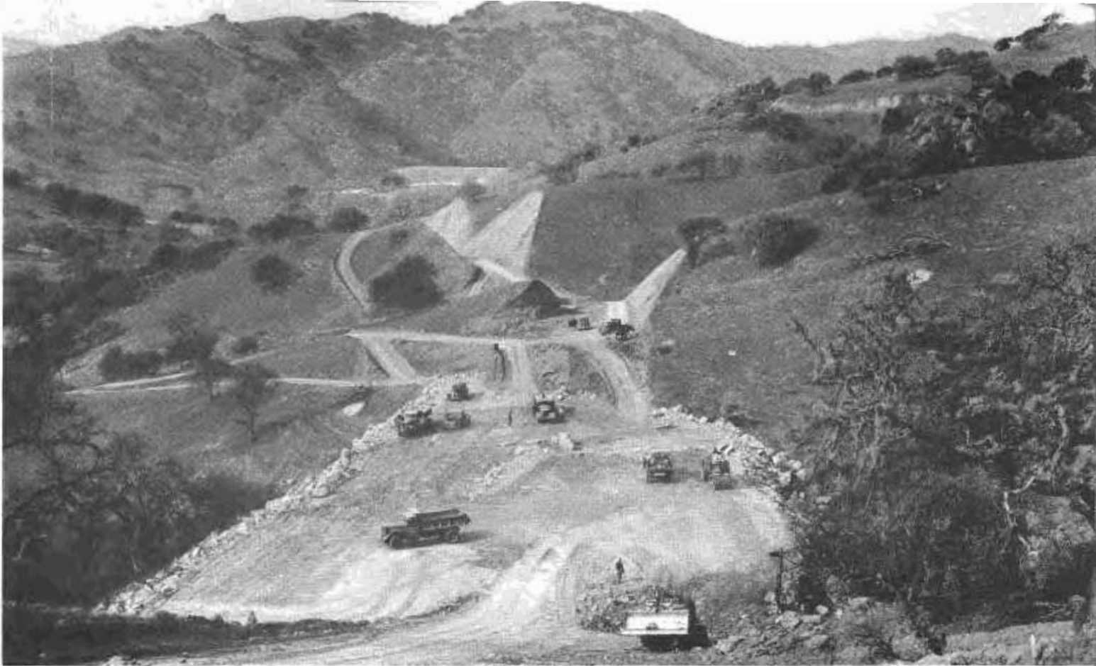
View of construction operations on section of Pacheco Pass realignment showing cuts and fills eliminating curves on upper level.
