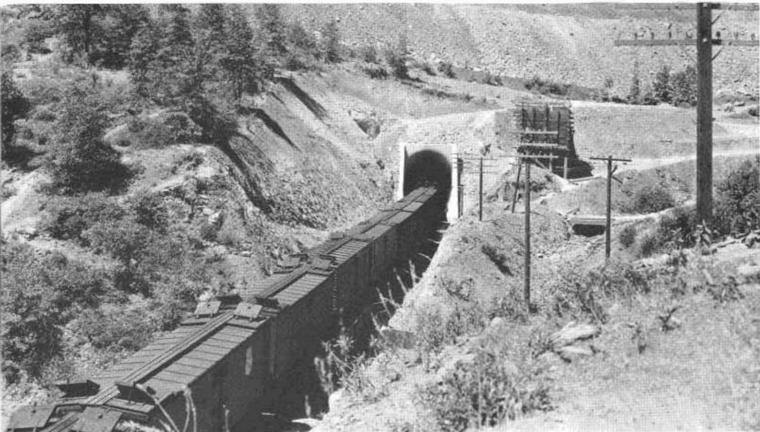
By-pass tunnel through west abutment of Shasta Dam, recently placed in operation as temporary route for trains to permit construction to proceed on the dam without interference to traffic.
