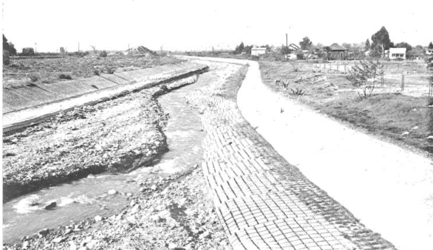
Toe of gunite facing protected by conformance of articulated concrete block apron to scour on Pacoima Creek, Los Angeles County.
