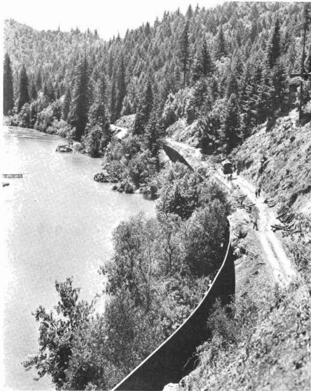
This view of construction on the Northwood Park-Guerneville Highway, looking towards Monte Rio, shows steel piles and treated timber bulkheads.
