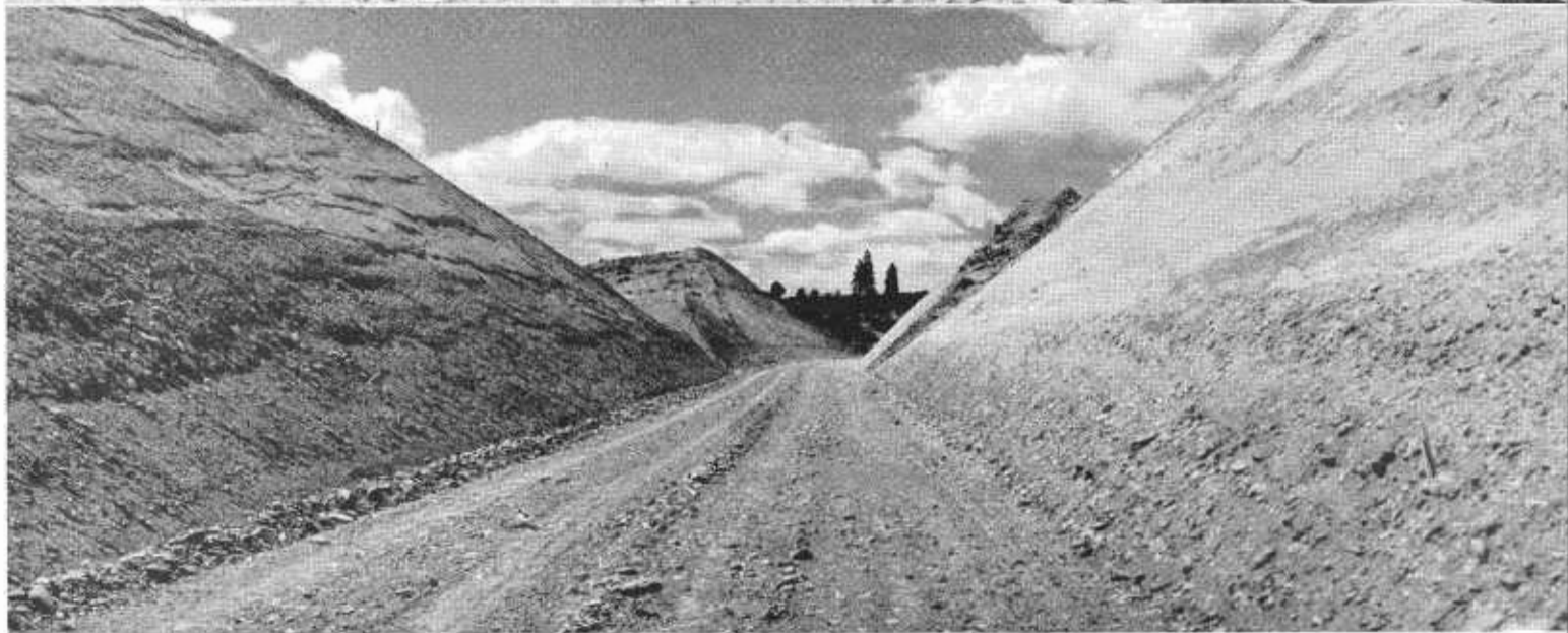
Construction progress on Southern Pacific Railroad relocation, Redding to Delta. Upper—4346-foot railroad bridge crossing Sacramento River near Redding. Center—One of twelve tunnels under construction. Lower—Completed section of grading north of Redding.
