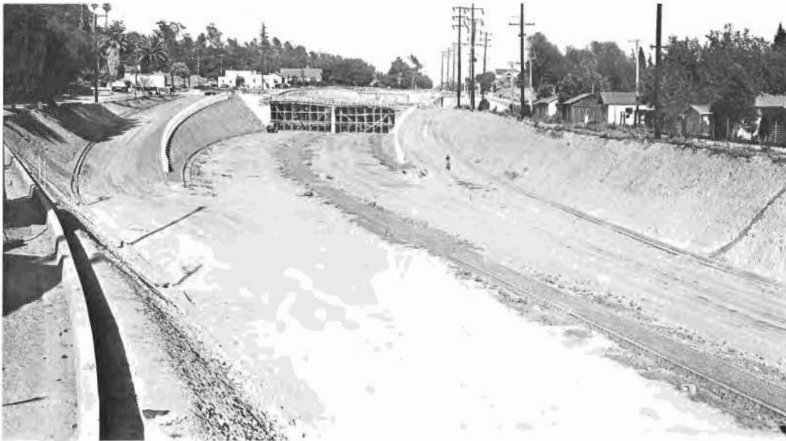
Bridge across Arroyo Seco Parkway on Orange Grove Avenue, Pasadena, is shown under construction flanked by off and on ramps.
