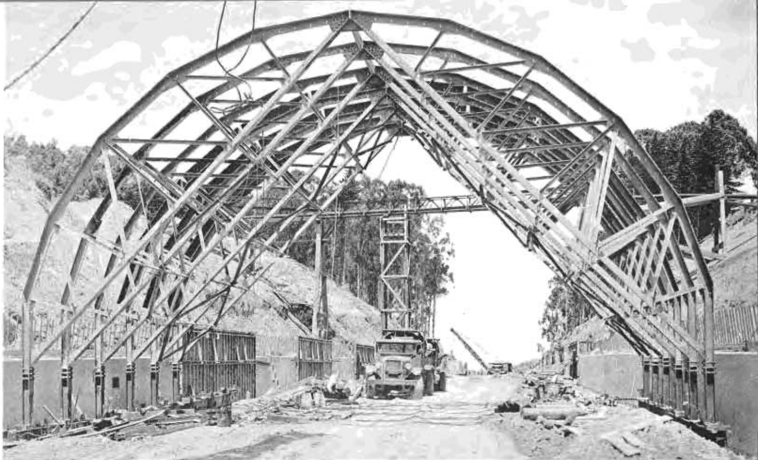
Erecting steel form jumbo preparatory to pouring arch for tunnel under Presidio golf course and Washington Boulevard.
