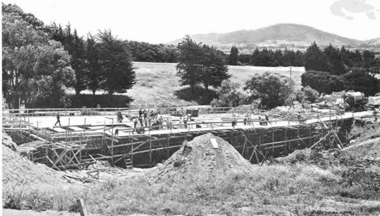
Pouring last section of the deck of Viaduct "A" which carries the approach highway over West Pacific arterial in the Presidio.
