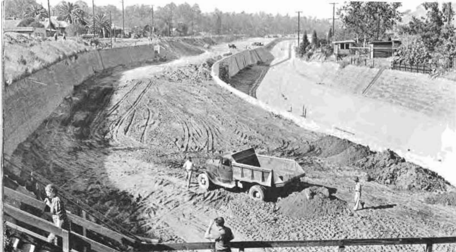
Constructing and compacting fill for Arroyo Seco Parkway which closely parallels the concrete lined arroyo channel throughout this section.
