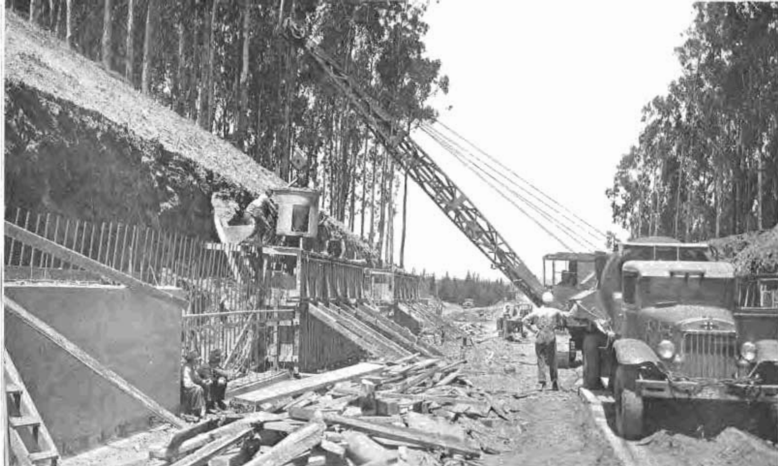
Pouring tunnel sidewall blocks. The tunnel, 1300 feet long, is being constructed by open cut and backfill method.
