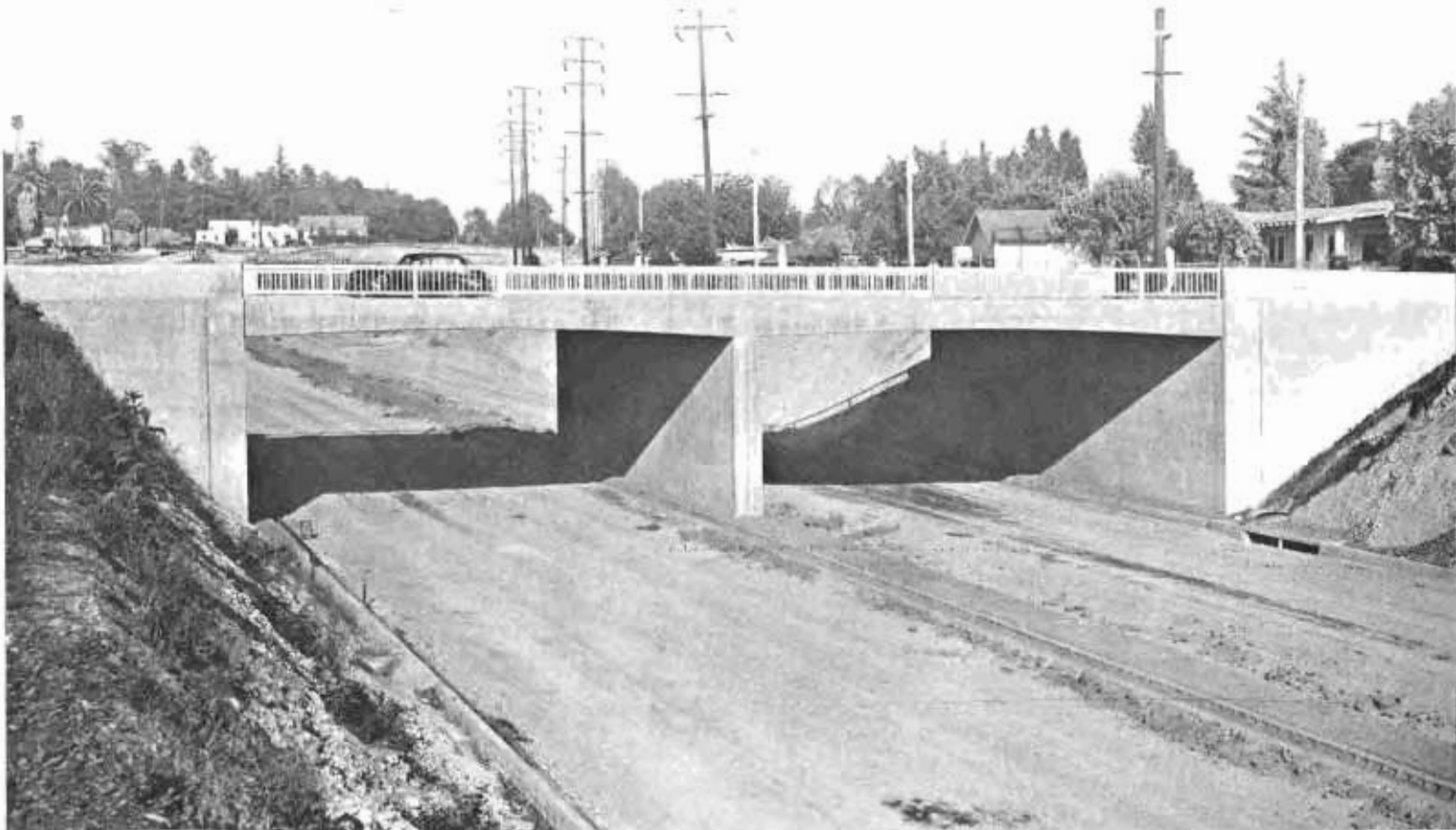
Newly completed bridge on the Arroyo Seco Parkway at Grand Avenue. Sixteen street and railroad bridges will cross the parkway.
