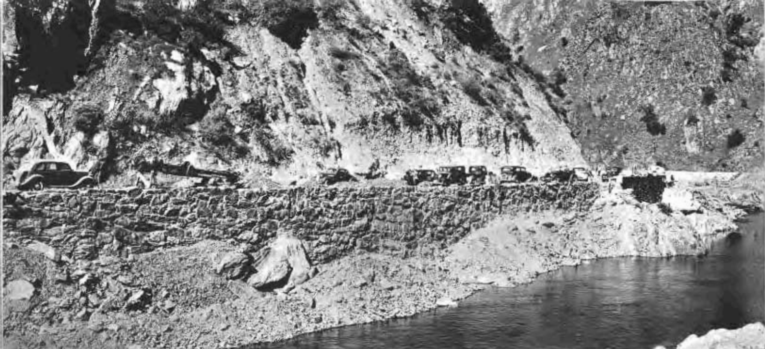
Section of rock wall flood protection being built on Yosemite Highway—Rock sizes from \frac{1}{2} cubic foot and larger.
