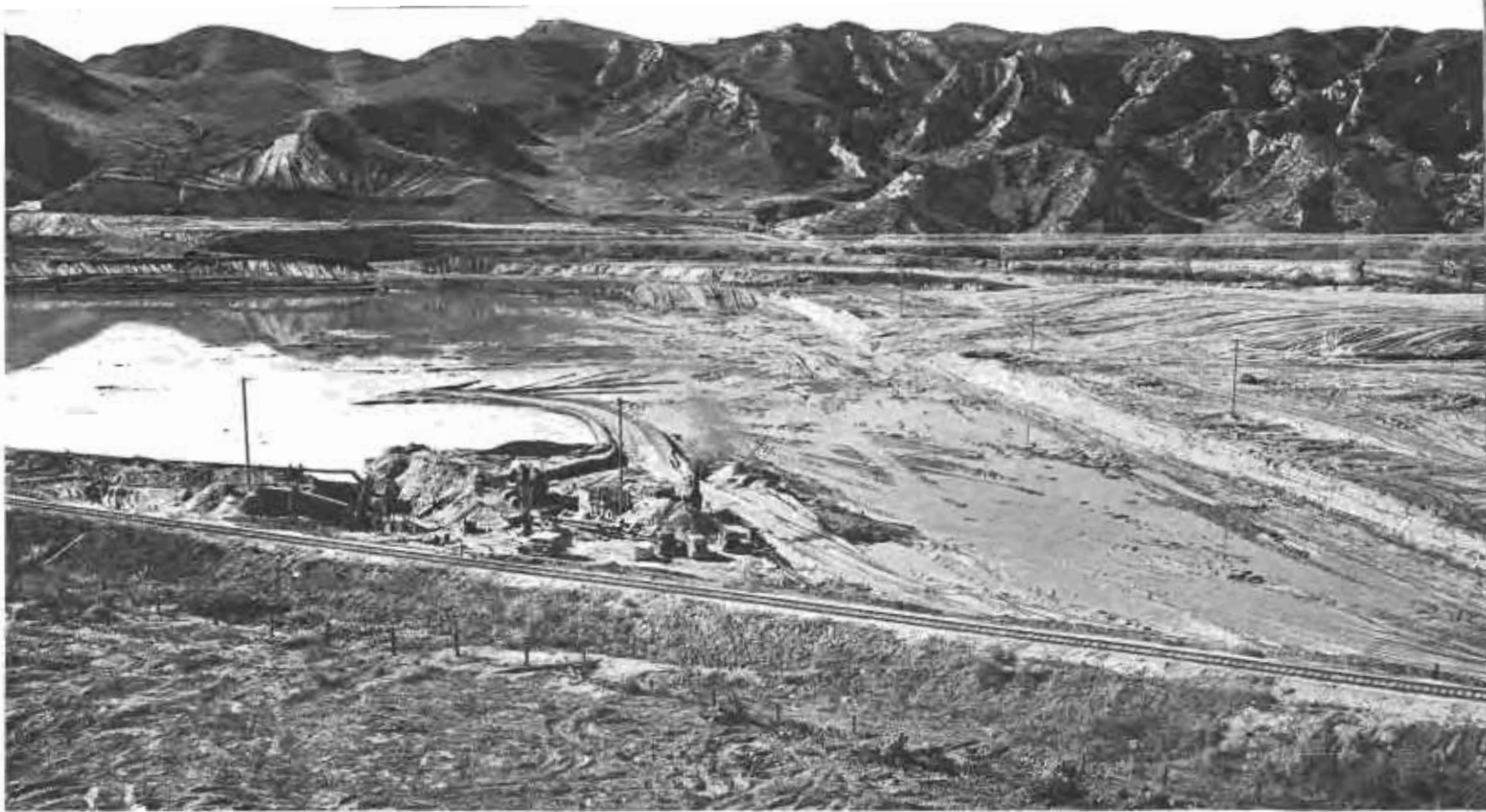
View of excavation operations under way at Prado Dam site on Santa Ana River compelling relocation of the State highway and the railroad tracks seen in foreground of picture.
