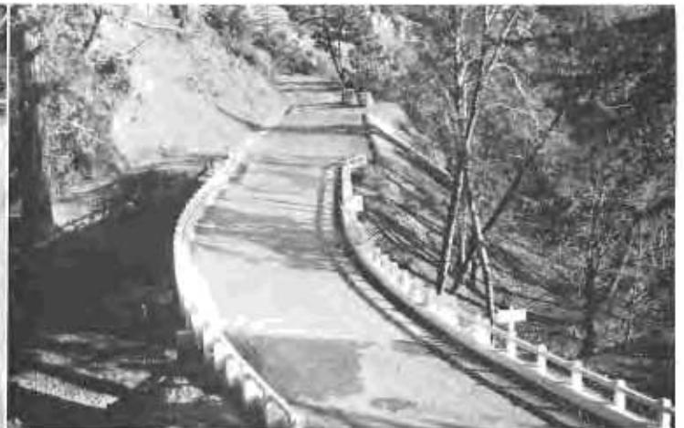
6—View of completed deck showing pleasing effect of new alignment and ample width of roadway.
