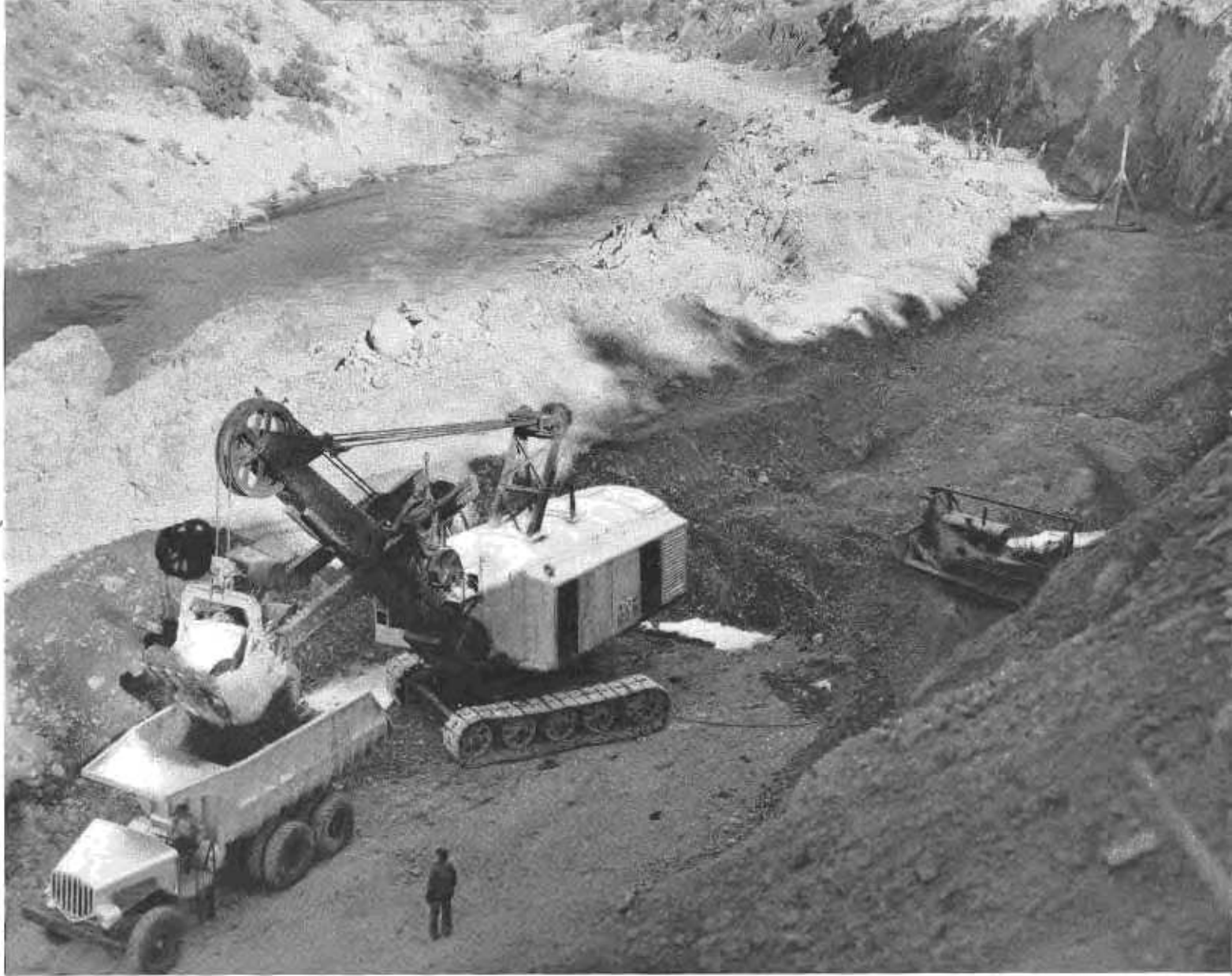
Excavating diversion channel at Shasta Dam site for Sacramento River, upper left. Shovel with 5-yard scoop filling 25-yard truck.
