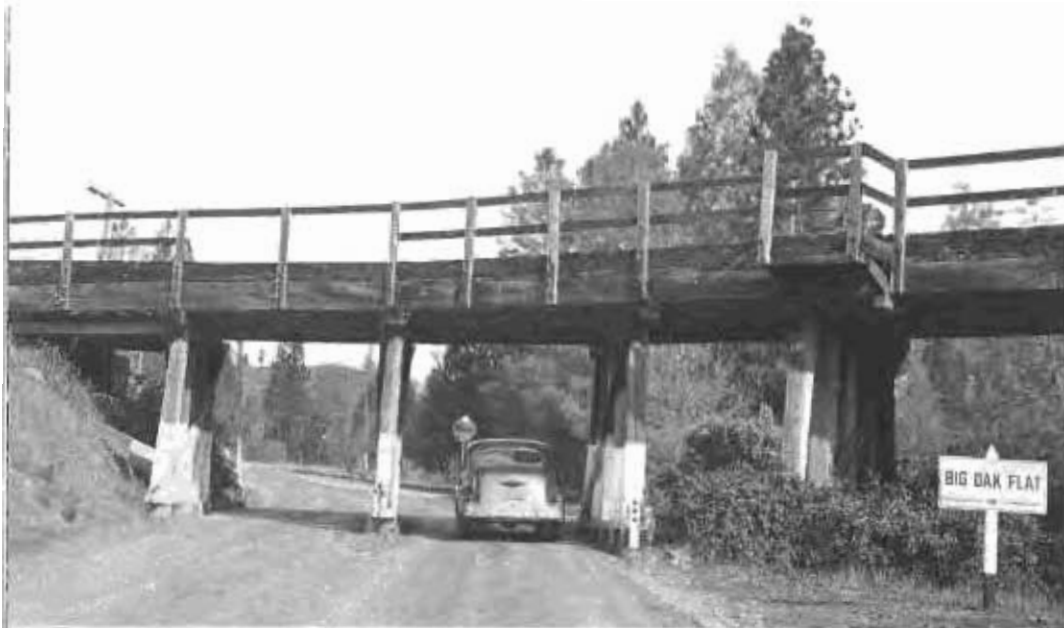
Top—Underpass below tracks of Hetchy Hetchy Railroad at Big Oak Flat, Tuolumne County, which is below legal clearance. Center—One-way road west of Coulterville in Mariposa County. Bottom—New Hope Landing bridge in San Joaquin County presents traffic hazards.
