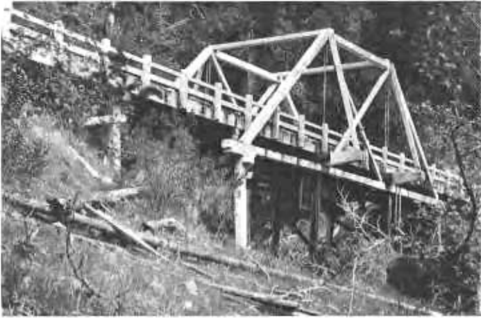
1—Old wooden Queen Post truss bridge which was replaced by modern deck structure.
