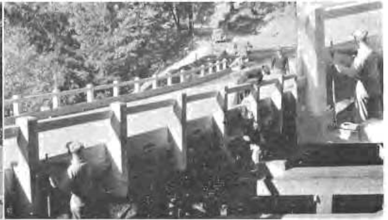
4—View of skidding operation in progress, showing jack operators and signal man. Insert shows jack installation.
