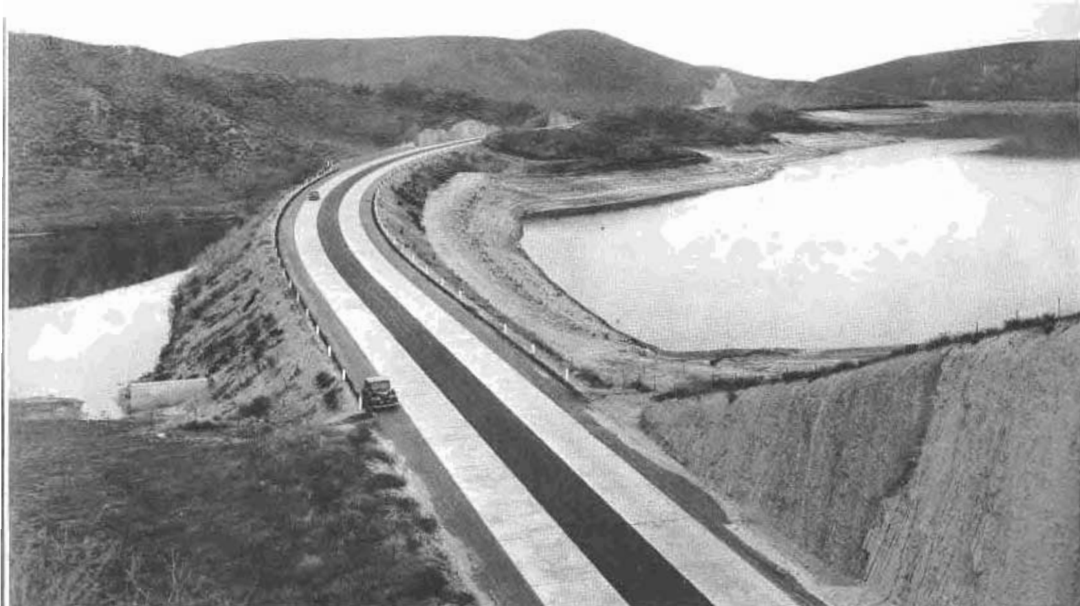
Section of recently completed Sepulveda Boulevard unit where it passes the lower San Fernando reservoir of the L. A. water system.
