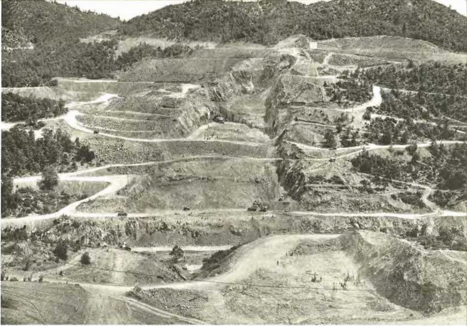
Progress of excavation at Shasta Dam site is shown in this picture of work on the east side of river. Photo by U. S. Bureau of Reclamation
