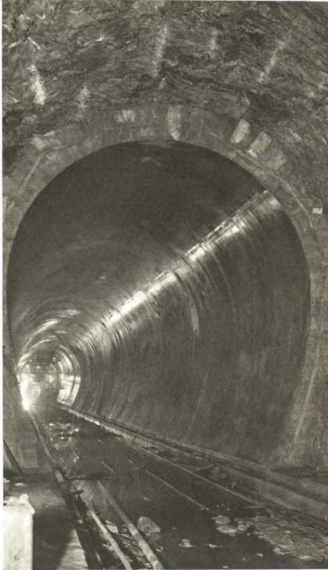
Photo by U. S. Bureau of Reclamation Through this by-pass tunnel, main line railroad traffic now crossing site of Shasta Dam will be routed early this Summer.
