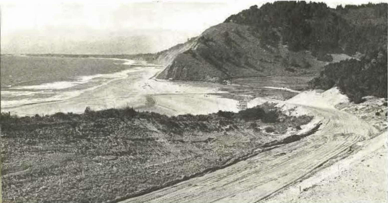
Relocation under construction on Ocean Shore highway north of Santa Cruz extending to Waddell Creek seen in middle ground.
