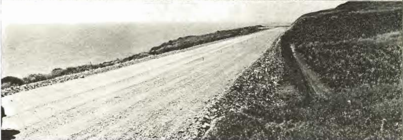
At top—Section of old narrow, winding highway on Coast north of Santa Cruz now being reconstructed. Project is 8.2 miles long, eliminating 133 curves and saving 2.1 miles in distance. Center—equipment at work widening grade. At bottom—Stretch of new roadbed along ocean bluffs showing straight, level alignment.
