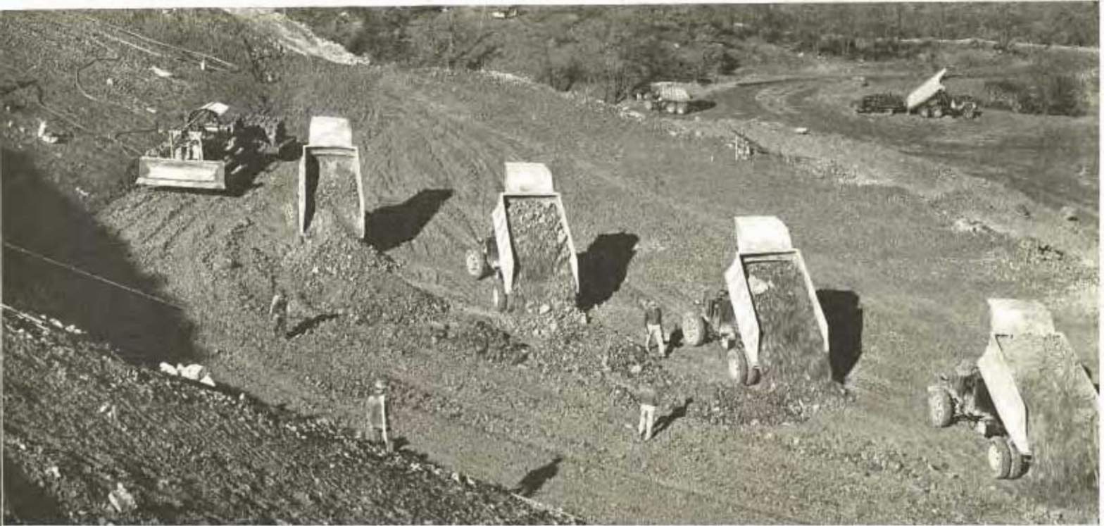
Placing excavated material in intermediate zone of upstream embankment section of Shasta Dam. Note bulldozer and sheepfoot roller at left.
