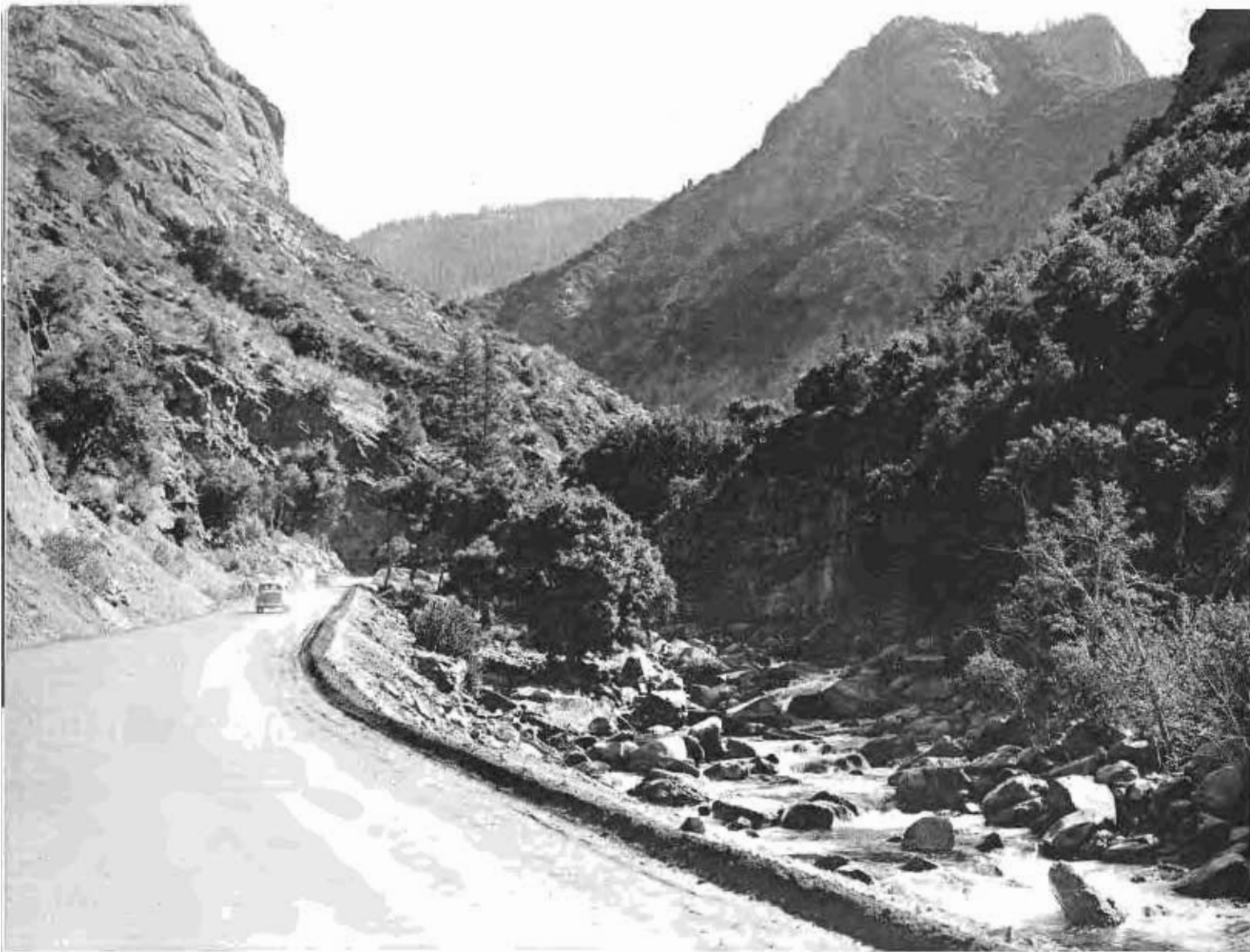
Section of new highway in Kings River Canyon between Grizzly and Boulder Creek showing glimpse of rugged south wall of canyon.
