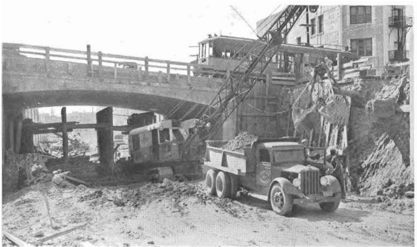
Heavy equipment constructing underpass for Figueroa Street while traffic proceeds on Temple Street in Los Angeles.
