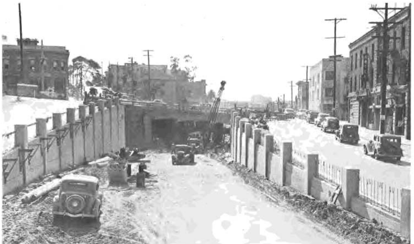
Permanent ramps built before excavation began permit Figueroa Street traffic to proceed during construction of underpass.
