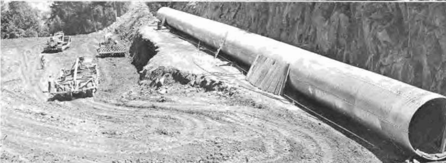
Construction scenes on highway relocation in Shasta County, showing grading operation, a completed section and building fill over large culvert.
