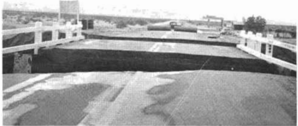
Approaches to bridge washed away by desert torrents on U. S. 60.
