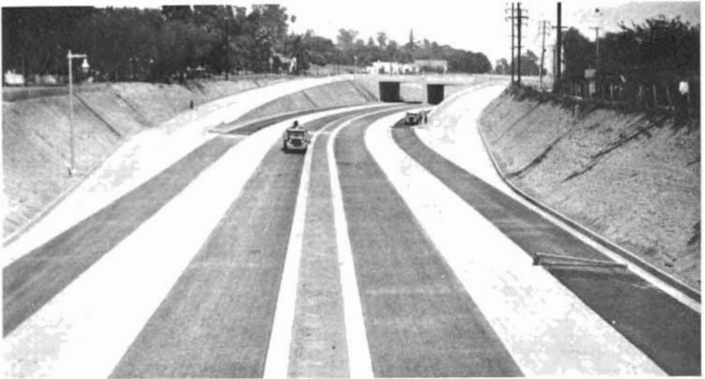
Sunken section of Arroyo Seco Parkway a 6-lane freeway with parallel service roads and no grade intersections as authorized by legislature, now under construction between Los Angeles and Pasadena.
