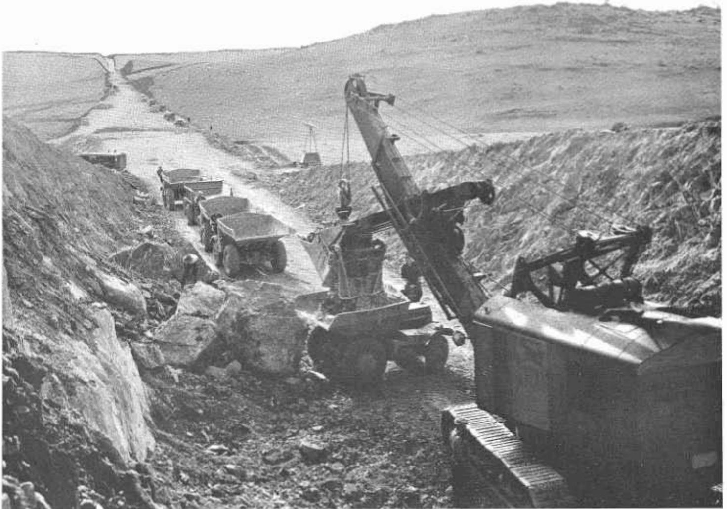
This is another view of construction on U. S. 50 between Folsom and Clarksville in El Dorado County.
