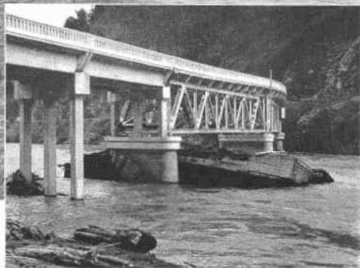
This view shows wrecked dredger washed against bridge piers.
