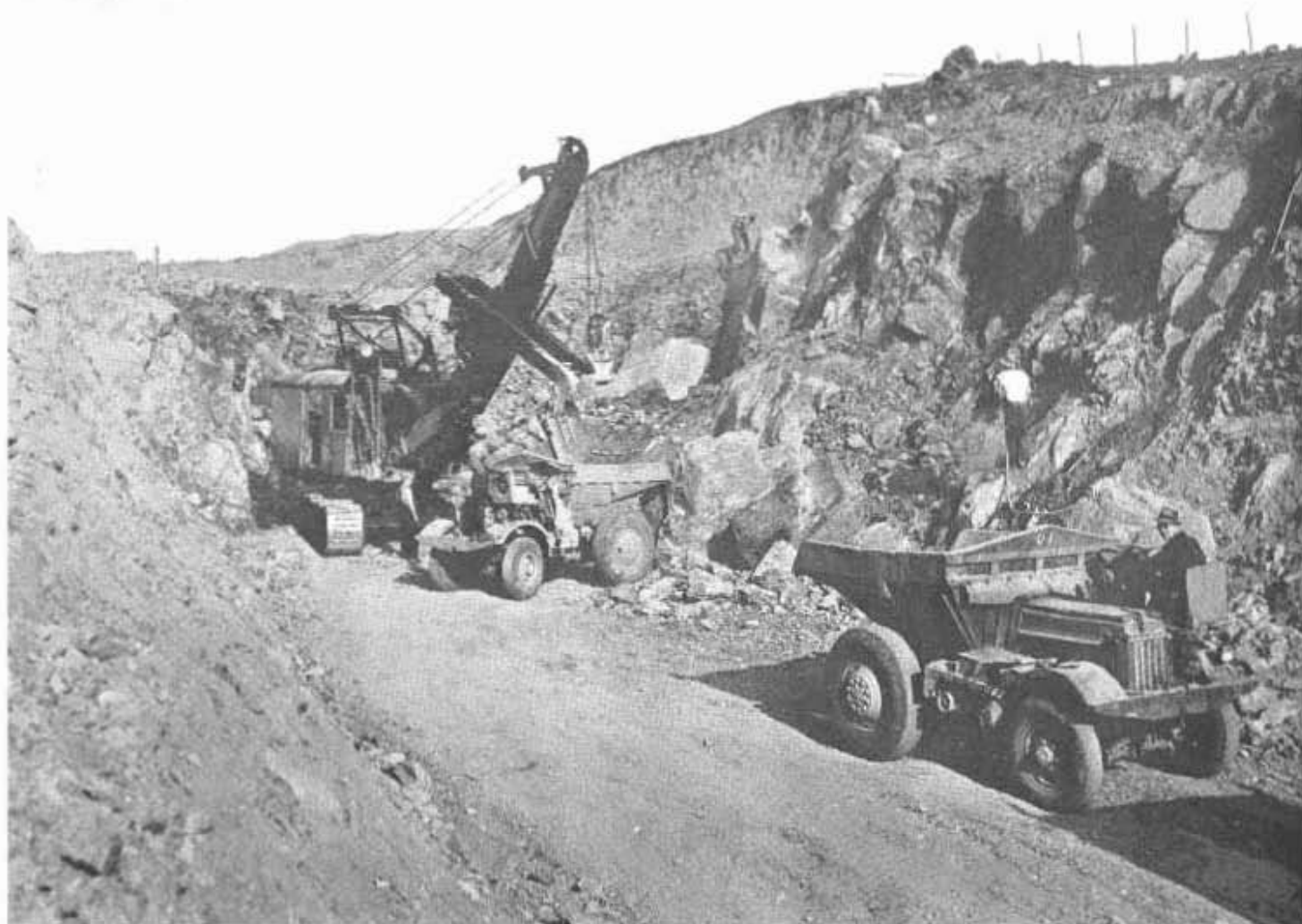
Shovel engaged in heavy excavation work in rock cut on realignment east of Folsom.
