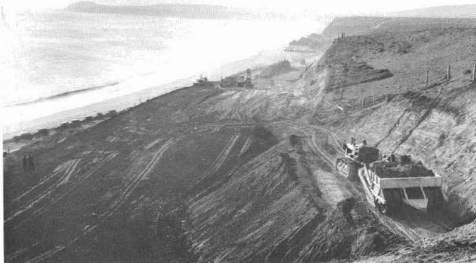
View of construction activities at summit cut between Latigo and Escondido Canyon.
