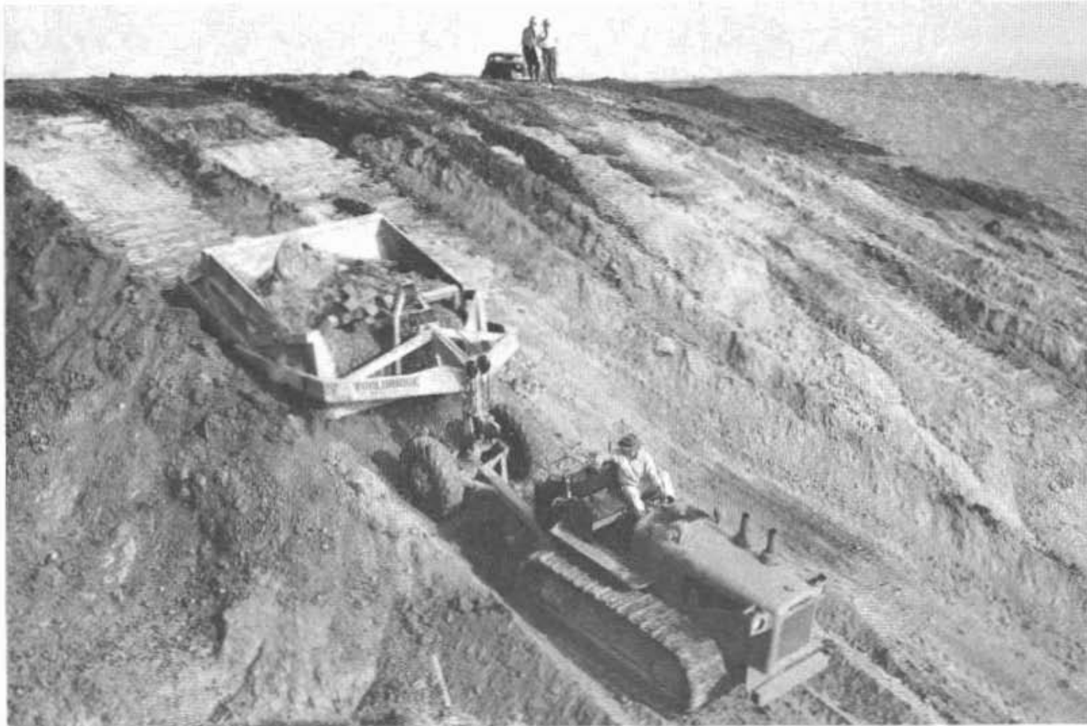
New type six-cylinder Diesel tractor pulling 15-cubic yard scraper on Roosevelt Highway construction.
