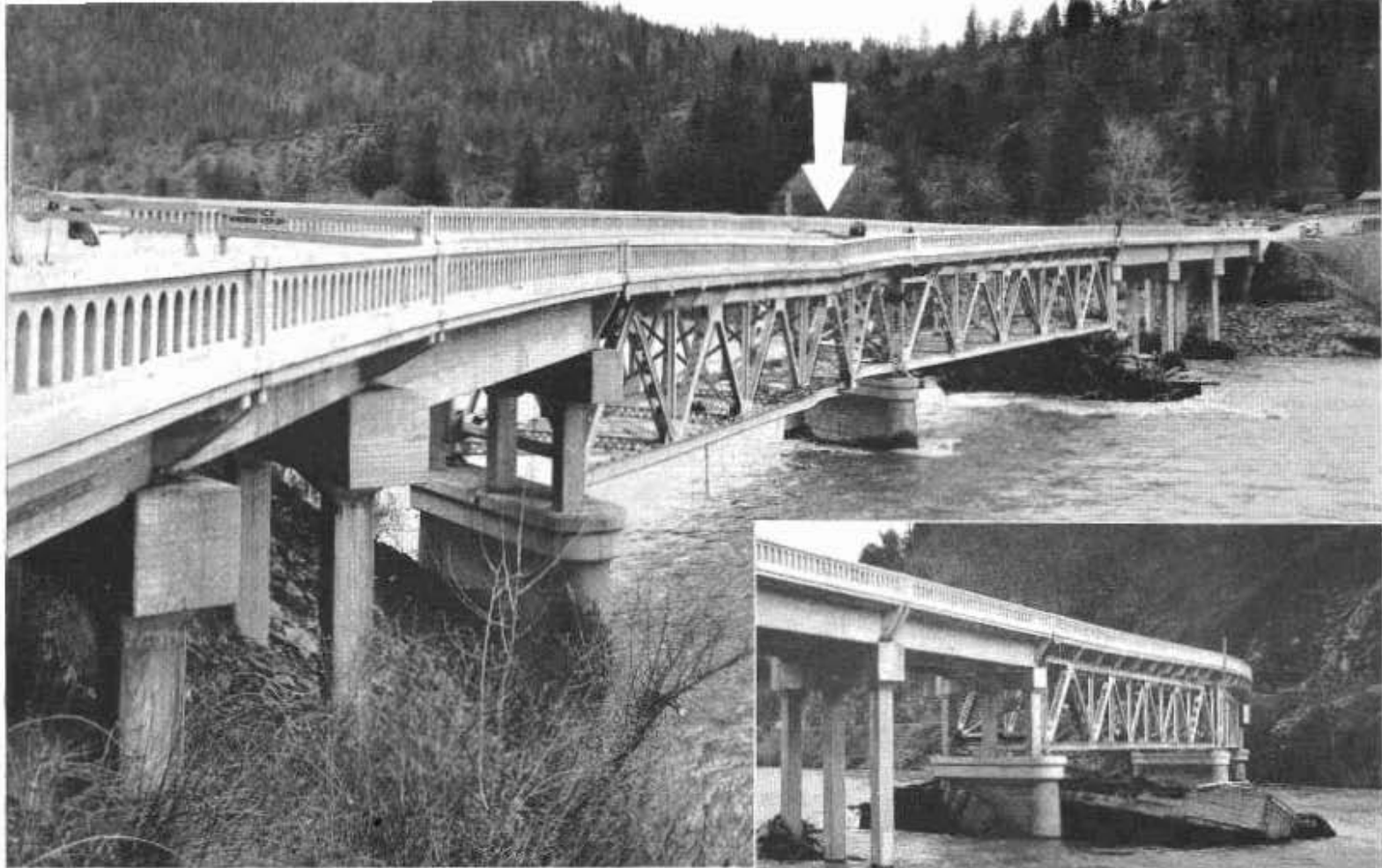
Flood-Damaged Highway Bridge across Trinity River near Douglas City. Arrow points to weakened section.
