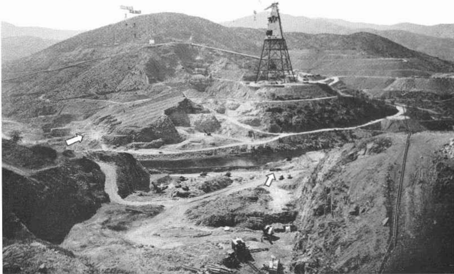
Shasta Dam site ready for pouring. First bucket of concrete was lowered from head tower cable to spot marked by white arrow in center foreground. Arrow at left center points to power house site and flume excavations.
