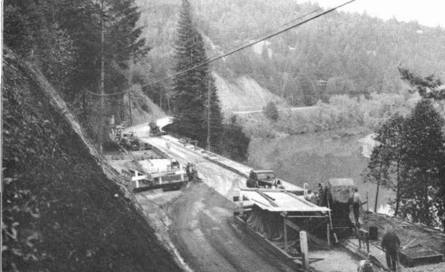
Constructing sidehill viaduct carrying State highway across slide area along Russian River
