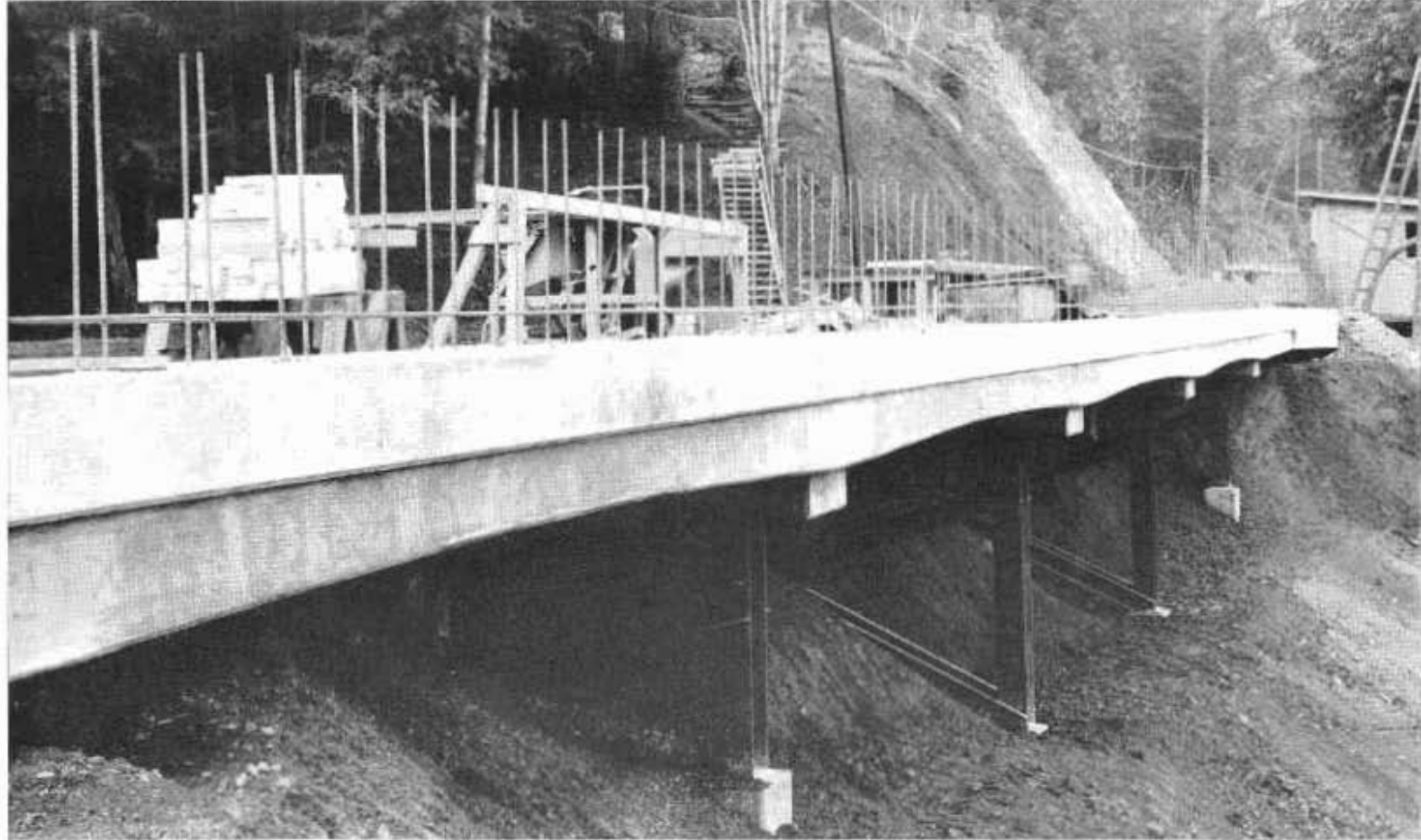
Two sidehill viaducts being constructed along the Russian River near Guerneville in Sonoma County provide 26-foot roadways of reinforced concrete. Continuous slab spans 20 feet in length are built on open steel pile bents. Four-foot pedestrian sidewalks with concrete rails are provided on the river side
