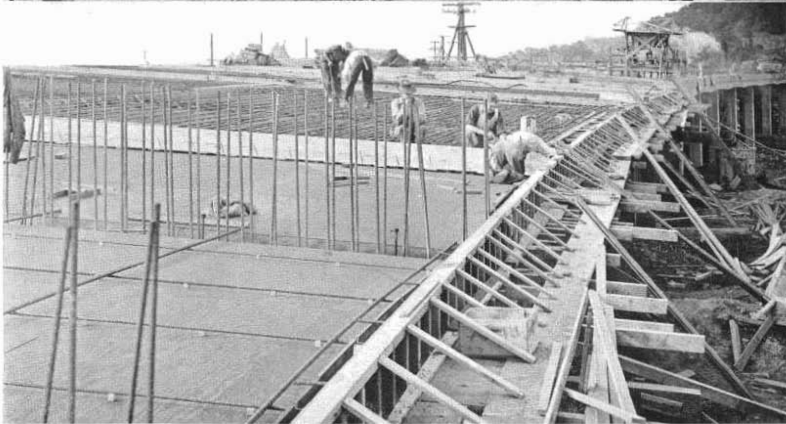
Upper picture shows 4-lane highway viaduct under construction through San Rafael at junction with existing highway to San Francisco. Lower shows deck forms and reinforcing steel details
