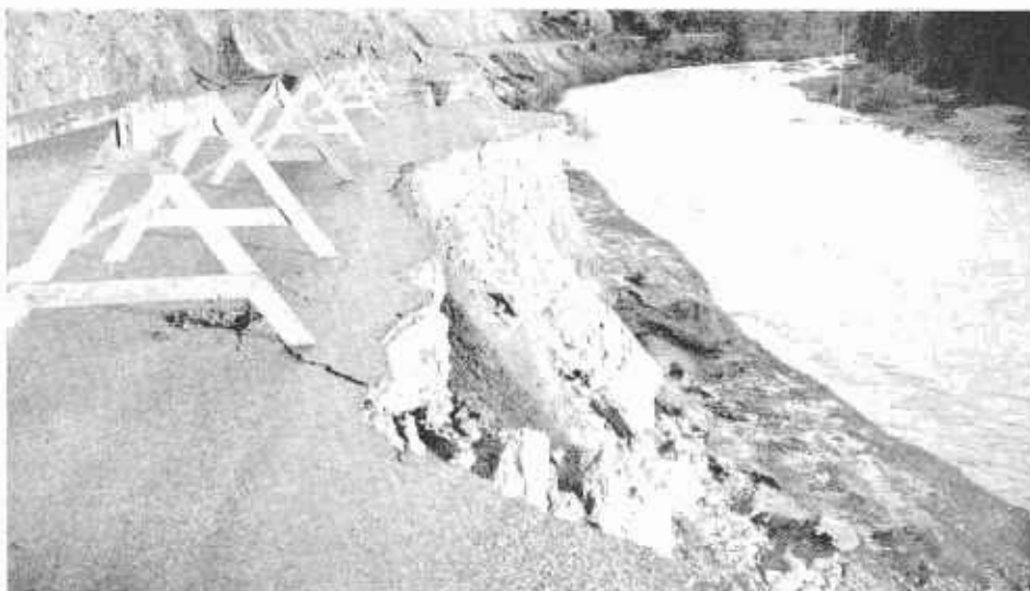
Flood damage on Redding-Alturas Highway, Shasta County in 1937 storm.
