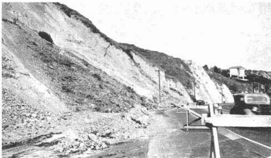
Large slide on Coast Route, north of Santa Monica, Los Angeles County.
