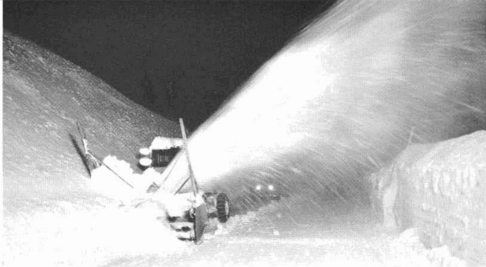
Auger blower rotary plows at work during night on Donner Summit highway (U. S. 40) clearing and keeping it open for traffic.
