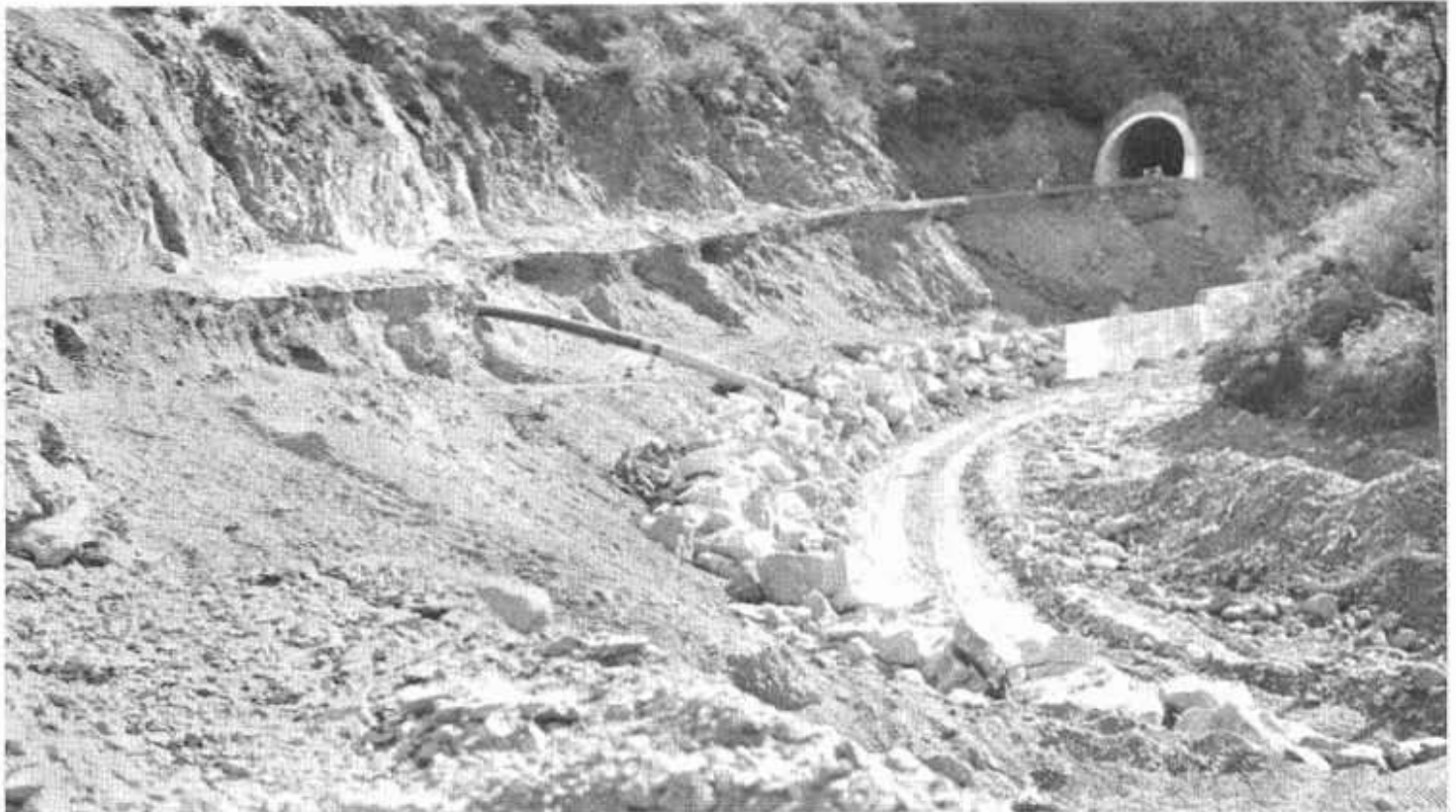
Washout north of Ojai on the Ventura-Maricopa Highway in Ventura County during the storm of 1938.
