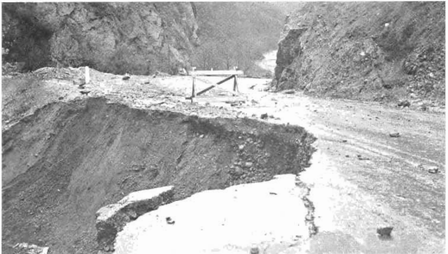
Typical Slip-out During Heavy Storm on Topango Canyon Route Near Santa Monica in Los Angeles County.
