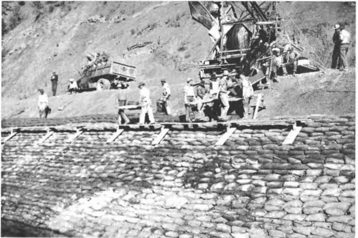
Scene showing bags being filled at concrete mixing machine and carried by crews for placement on Cache Creek embankment.
