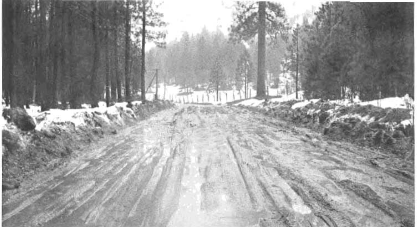
Winter Failure of Light Surface North of Quincy, Feather River Route, from Storm and Traffic Conditions.
