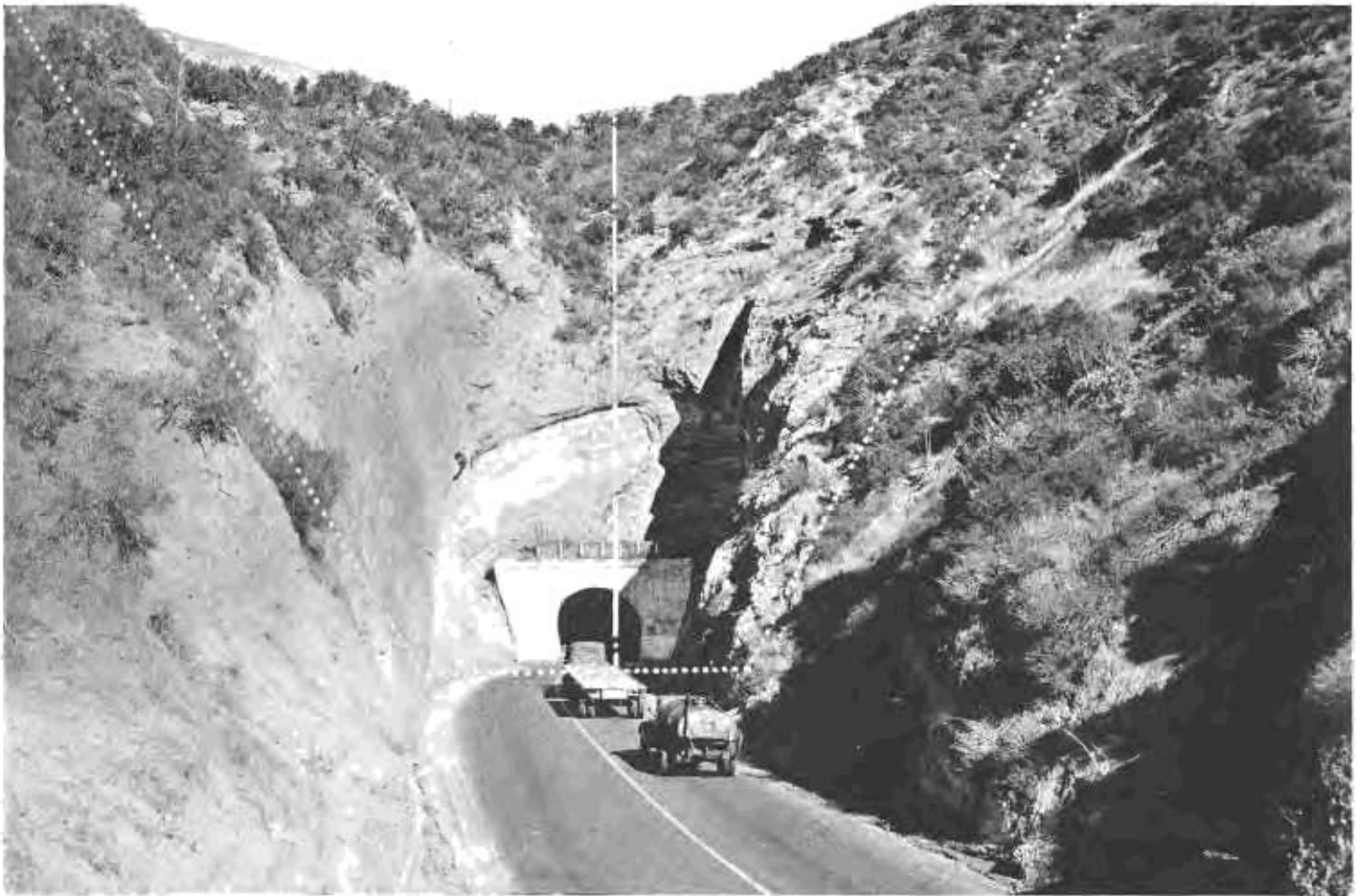
Narrow Newhall Tunnel bottleneck on State Highway 23 as it appeared before excavating of cut slopes as indicated by dotted lines.
