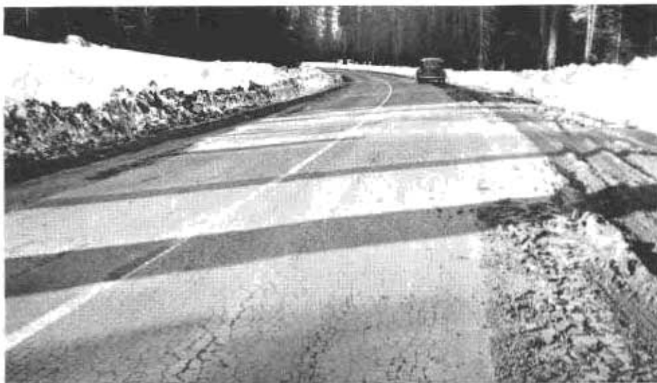
Failure of Red Bluff-Susanville Route Due to Inadequate Base.
