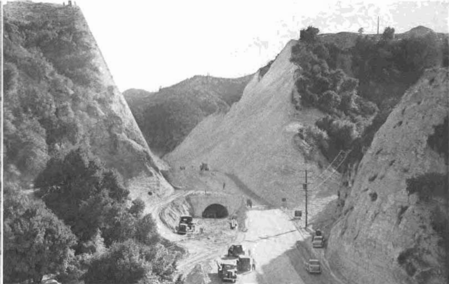
Santa Susana Mountain ridge in process of being cut through to transform Newhall Tunnel into an open cut highway.
