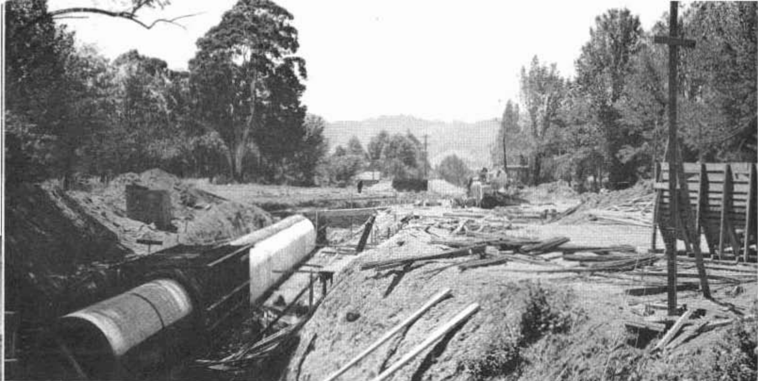
Construction of reinforced concrete arch culvert to carry waters of Irwin Creek under four streets beneath viaduct through San Rafael.
