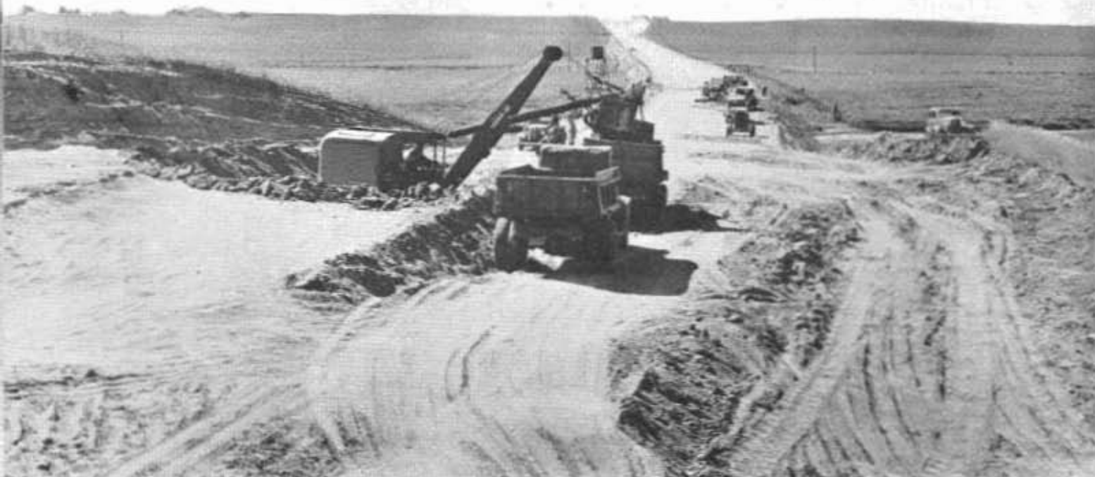
Equipment at work on "Ducor Cut-off," a portion of the Orange Belt highway in Tulare County near Porterville.
