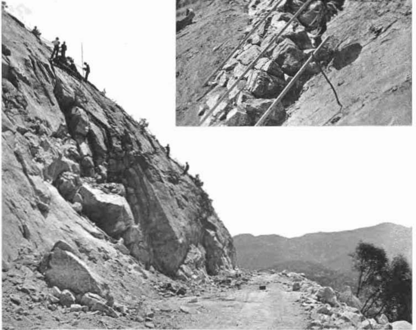
At top, Construction of rock retaining wall on PWA link of Grant Park approach road. Bottom, Drilling for removal of cliff.
