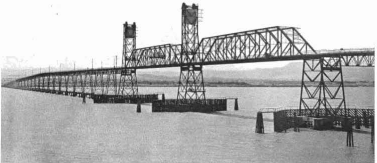
Privately owned Antioch Toll Bridge across the San Joaquin River on State Highway Route 11 near Antioch, Contra Costa County.
