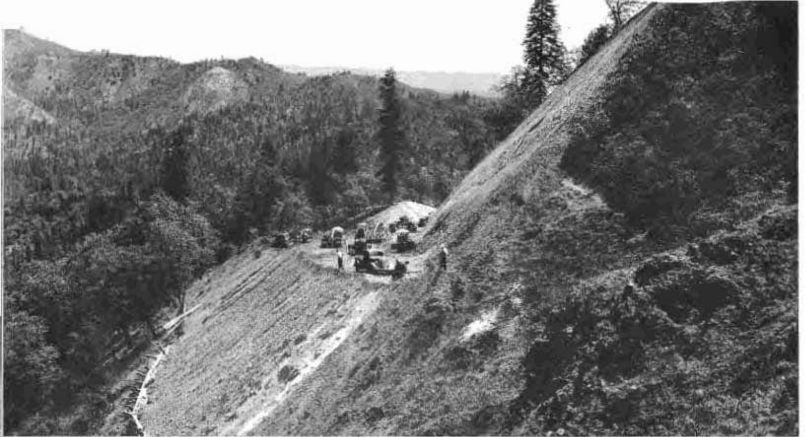
State Highway relocation on U. S. 101 between Bass Hill and O'Brien Summit involves record grading in Northern California.
