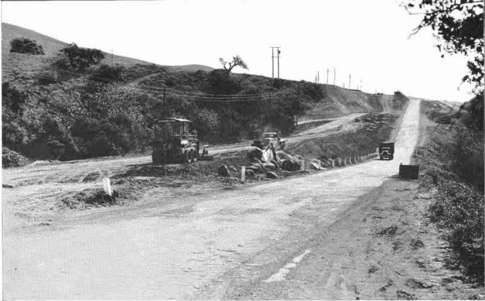
View of new grade under construction east of El Capitan Creek while traffic uses the existing highway.
