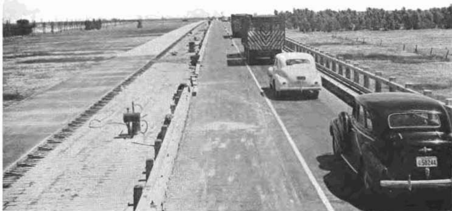
Paving Yolo Causeway with reinforced concrete. Traffic is kept moving in two of the four lanes while work is under way on the other two except for intervals while concrete is setting when one-way traffic control is in effect.
