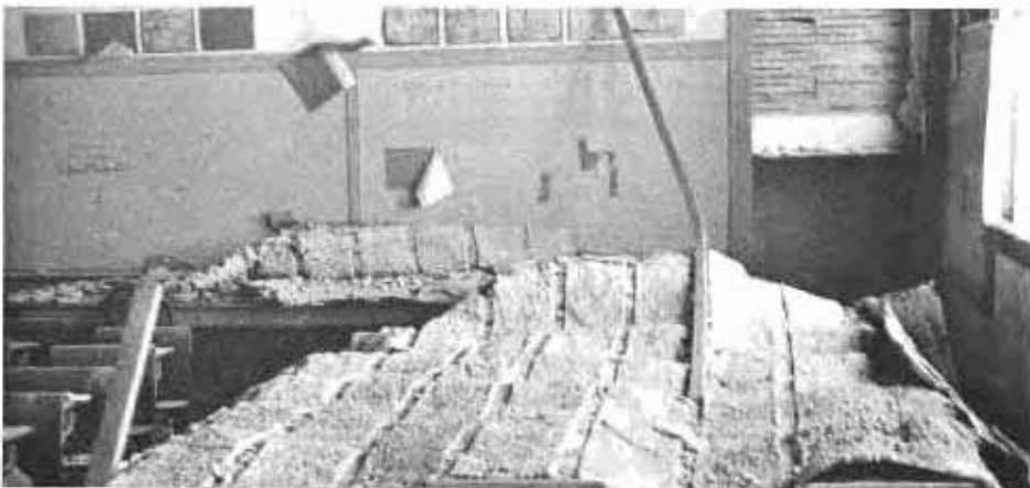
Ceiling dropped to floor in one old school.
