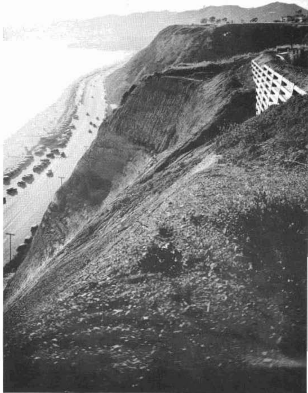
This photograph shows a completed section of slide prevention work near Santa Monica where retaining wall prevents slides from blocking State Highway seen at base of unstable cliff. Highway traffic was endangered by these Palisades.
