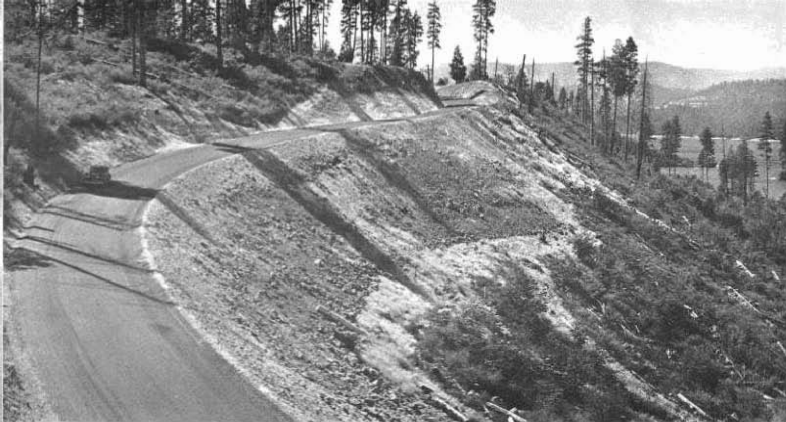
Typical stretch of recently realigned highway between Lake Britton and Burney Falls on Sierra Way.
