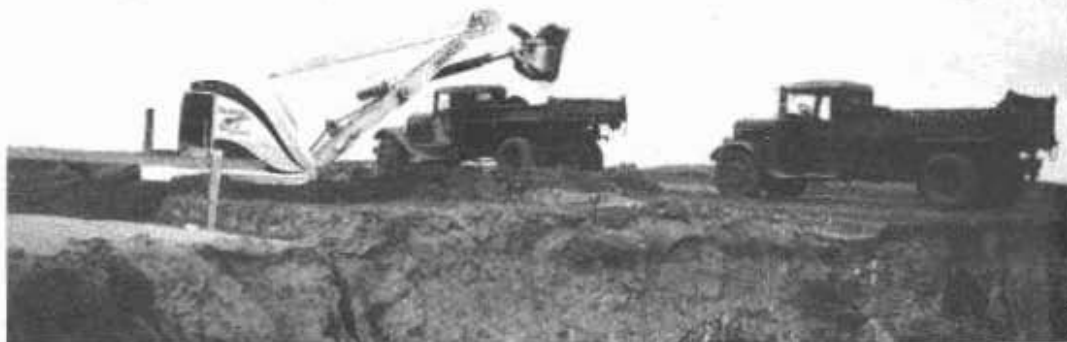
Top—Crew finishing cut slope on Kern County's section of cut-off. Center—Graded roadway nearly completed. Bottom—Shovel purchased by Kern County for project.
