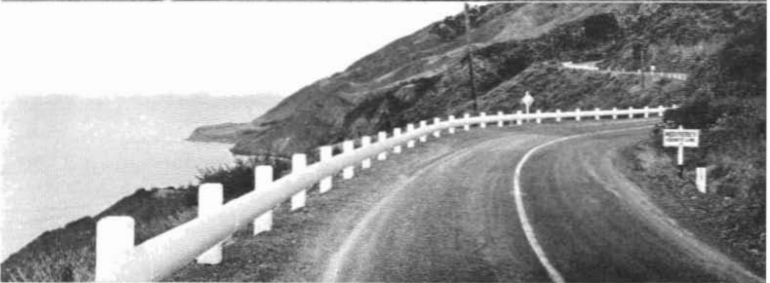
Views on Monterey Coast Highway between San Luis Obispo County line and Big Sur showing installations of steel guard rail
