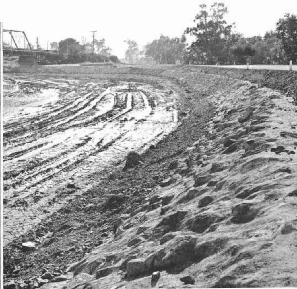
Detail of the boulder facing set in Portland cement for slope protection
