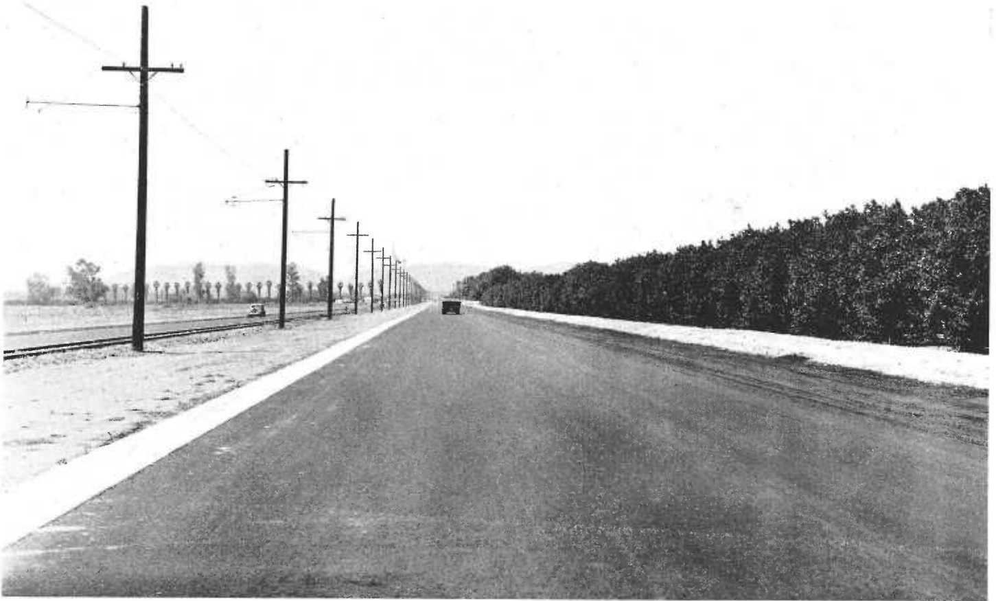
Reconstructed section of Sepulveda Boulevard showing railroad right of way used as division strip with new pavement for north bound traffic
