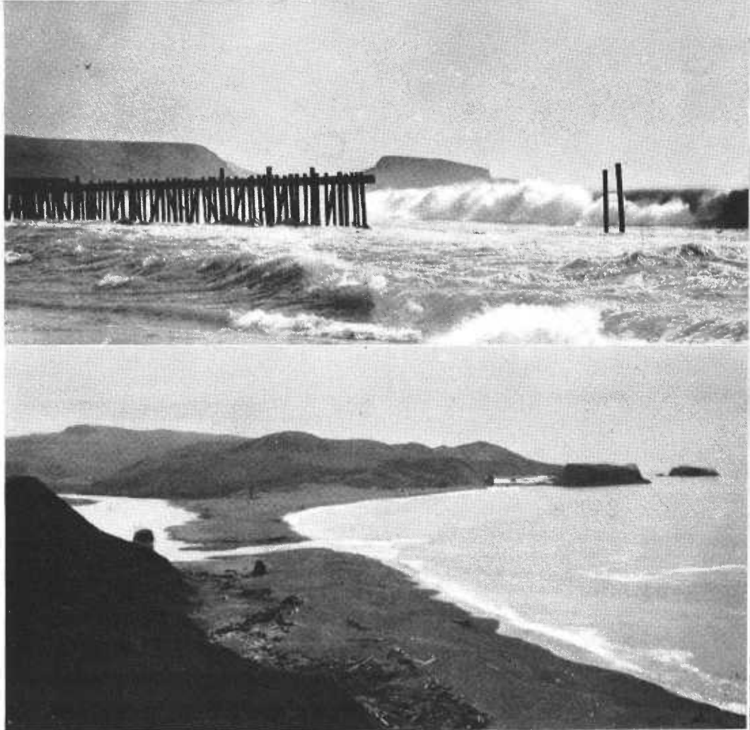
At top, part of old jetty remaining at mouth of Russian River. Center—Waves destroying construction trestle. Bottom—River mouth almost closed by sand
