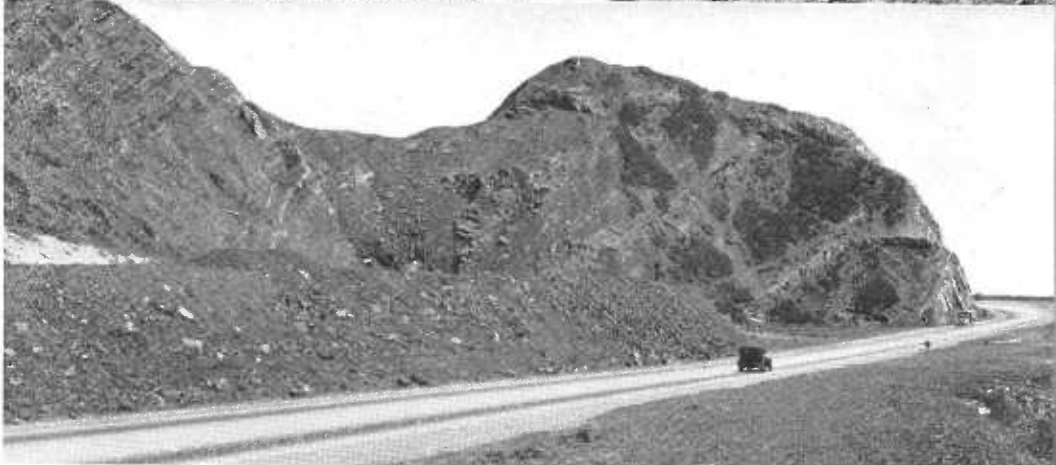
Blasting and excavation scenes at cut through Point Mugu and old road around ocean end of mountain
