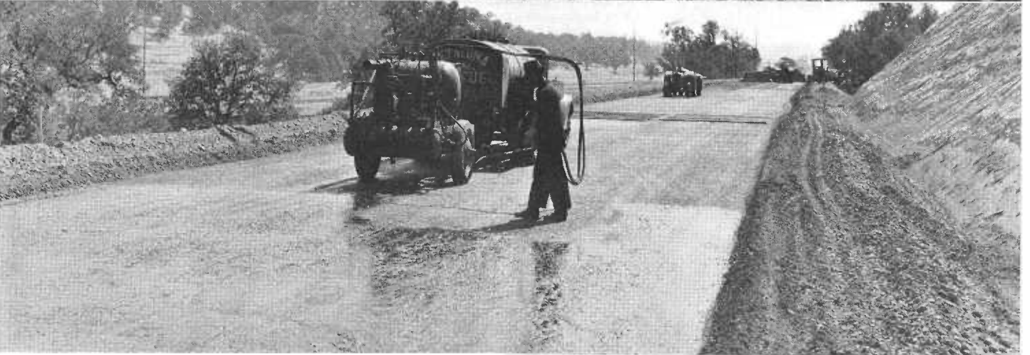
Top and center—Views of dumping and rolling cement stabilized base material on prepared subgrade of relocation north of Red Bluff Bottom—Operation of applying curing seal of asphaltic emulsion on prepared subbase.
