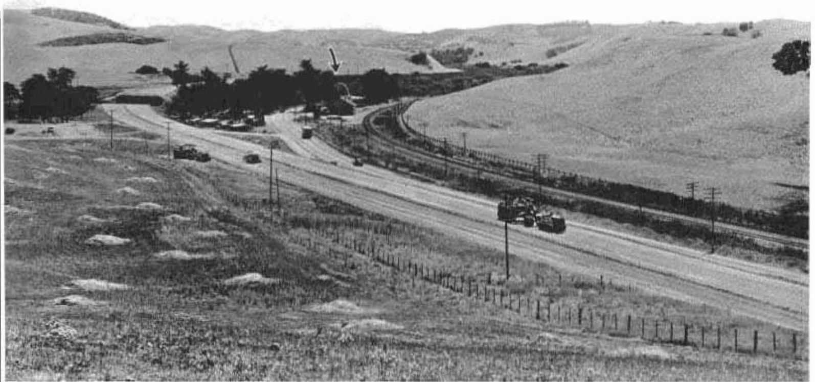
Realignment under construction at Pajaro River Crossing of U. S. 101. Arrow points to old one-way bridge on existing road
