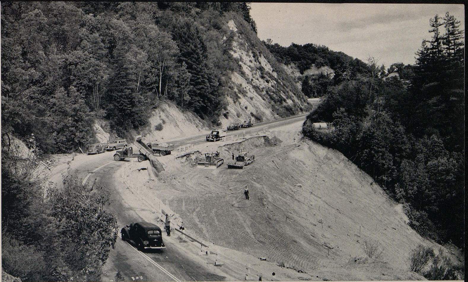
View of last stages of 30,000 cubic yard fill restoration at slipout on Los Gatos-Santa Cruz Highway.
