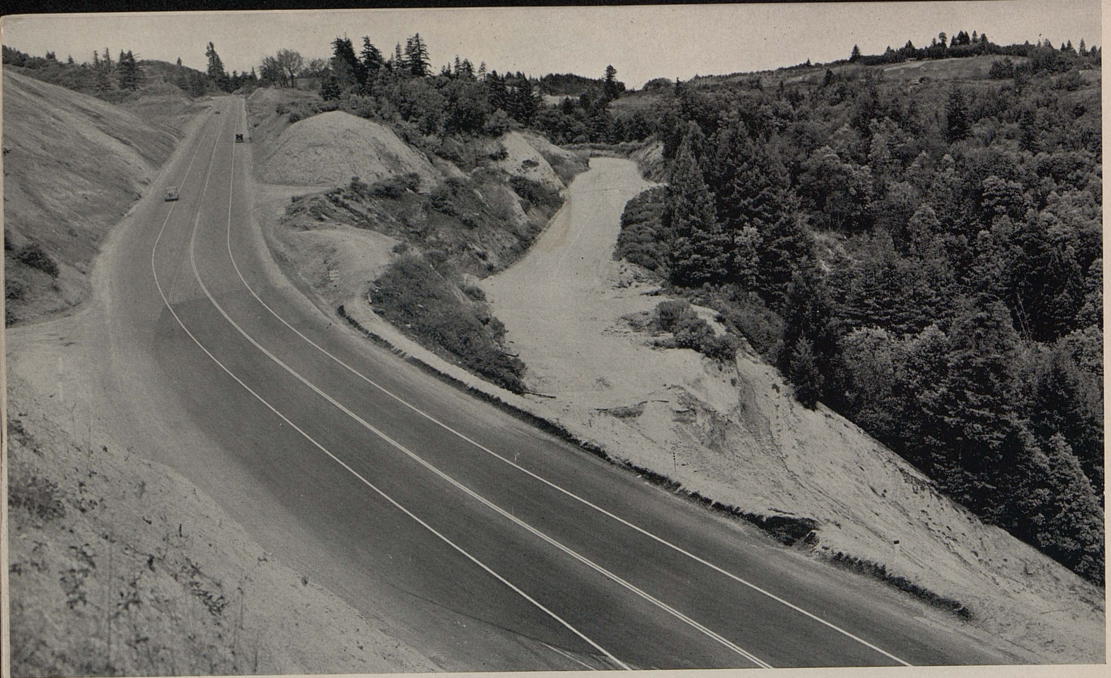
Completed repair of slipout at junction of old and new highways 12 miles north of Santa Cruz. Dark pavement marks area of slipout.
