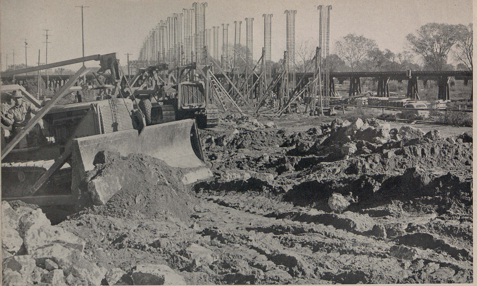
Equipment tearing up old pavement and grading for south approach to new North Sacramento Viaduct structure.
