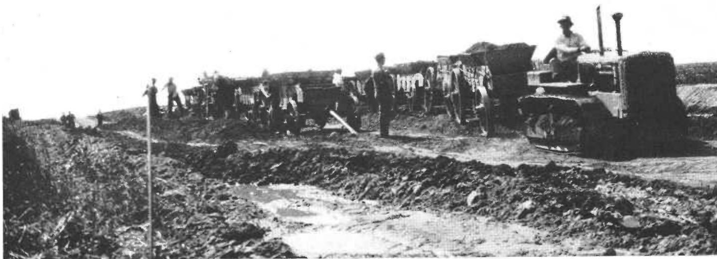
Complying with W.P.A. regulations dirt was moved by wagon trains filled by hand labor and hauled by tractor
