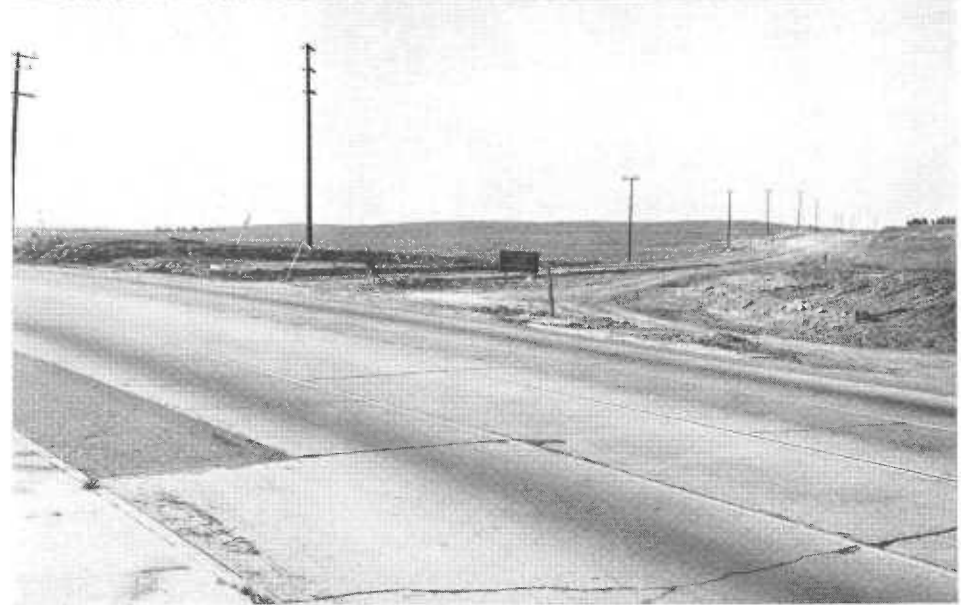
Construction Scenes on Santa Ana-Corona del Mar Highway Link. Top—Culvert Construction near Santa Ana. Center—Graded route at Corona del Mar end. Bottom—Junction point with Coast Highway
