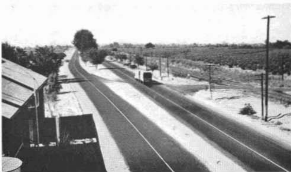
New divided road construction saves and utilizes on division strip trees that bordered roadside of old highway
