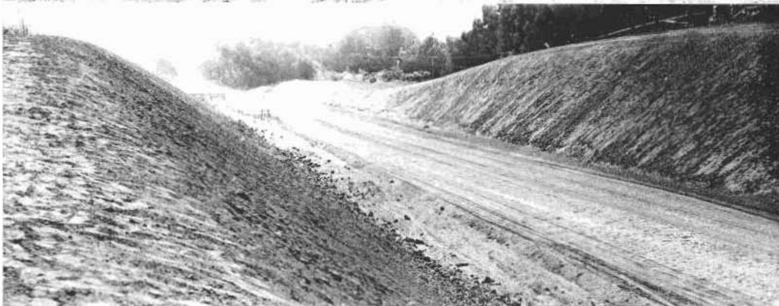
Top—Rough graded section of realignment of Coast Highway west of Santa Barbara. Center—Cut slopes being rounded preparatory to application of top soil. Bottom—Top soil applied and left rough to permit natural vegetation to gain a foothold
