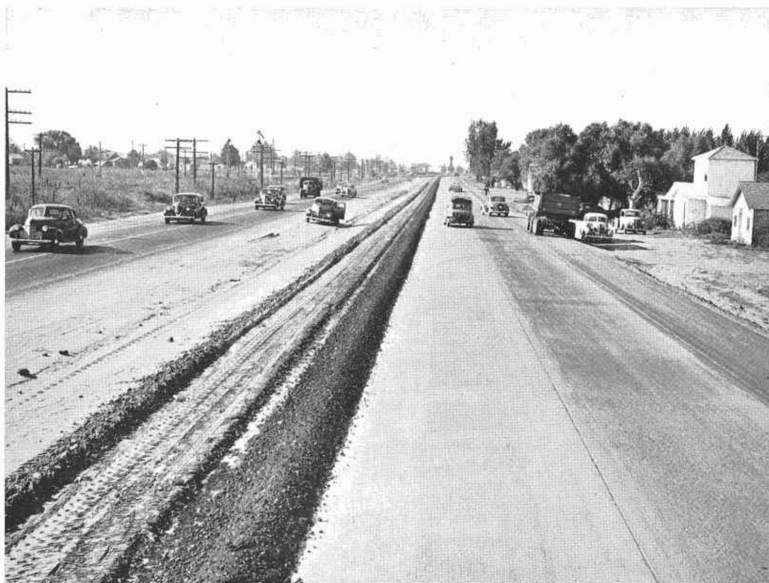
Divided highway unit of U. S. 99 nearing completion south of Modesto with traffic using outside lanes
