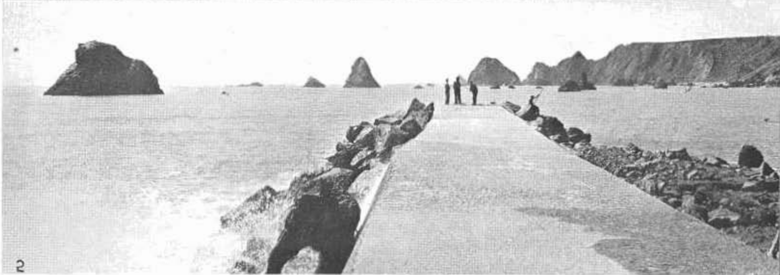
Views of rock and concrete jetty at Jenner that is keeping open Russian River channel to ocean
