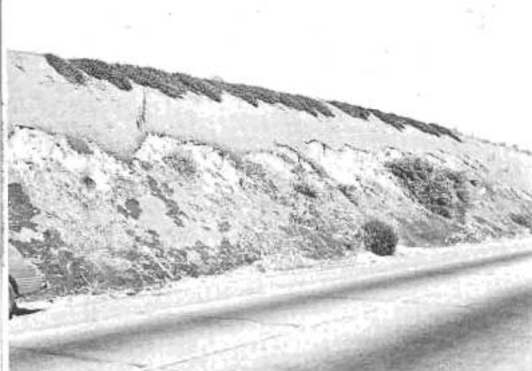
Erosion control by artificial means such as oiling is always subject to failure and demands constant repair
