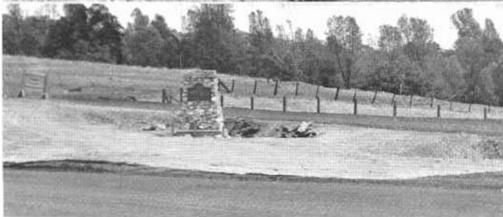
Top—Section of realigned highway into Jamestown. Center—Mother Lode vein exposed by highway cut. Bottom—Gold discovery monument near highway
