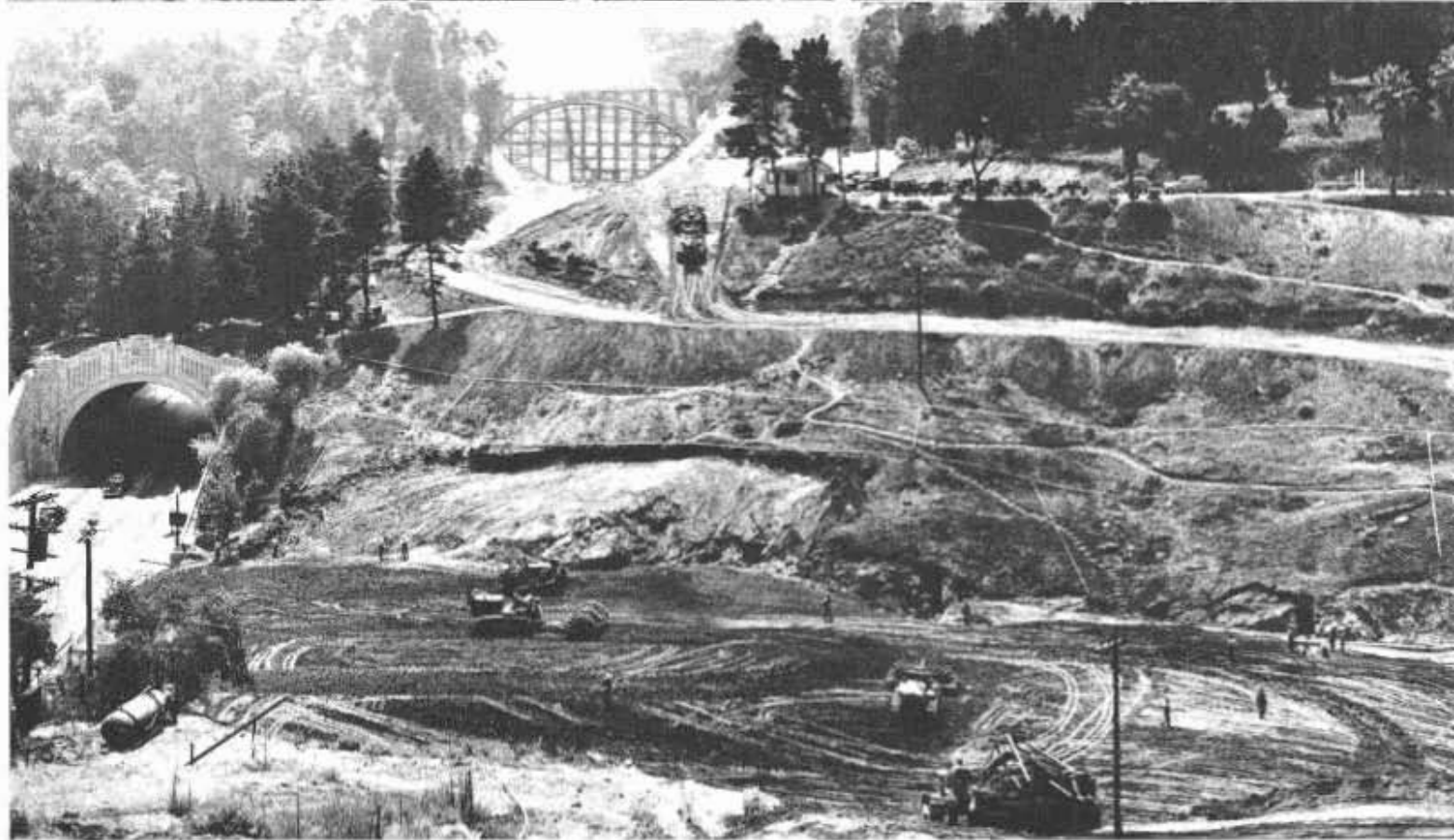
Top view shows existing Figueroa Street tunnel on right and construction at Solano Street grade separation with Park Lane bridge in background. At bottom—Extensive grading at site of Bishops Road grade separation and construction of dam that will also serve as highway embankment. Excess excavation material is used for dam which permits extension of city-owned reservoir
