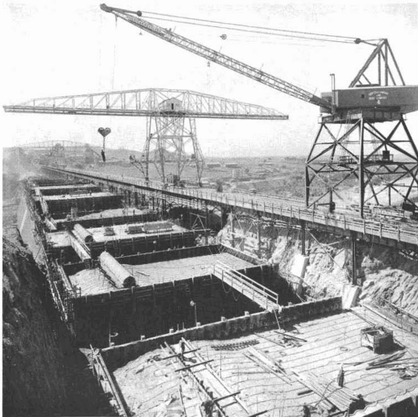
This view of Friant Dam shows the progress of concrete pouring made to date by the trestle and crane system
