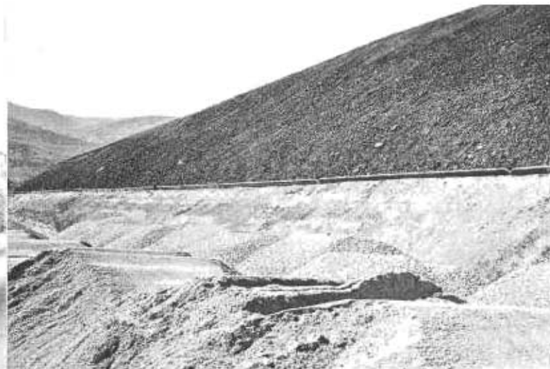
Finished 1½:1 slope too smooth to retain lumpy adobe top soil. Header-board above plant mix ditch line to hold cover soil
