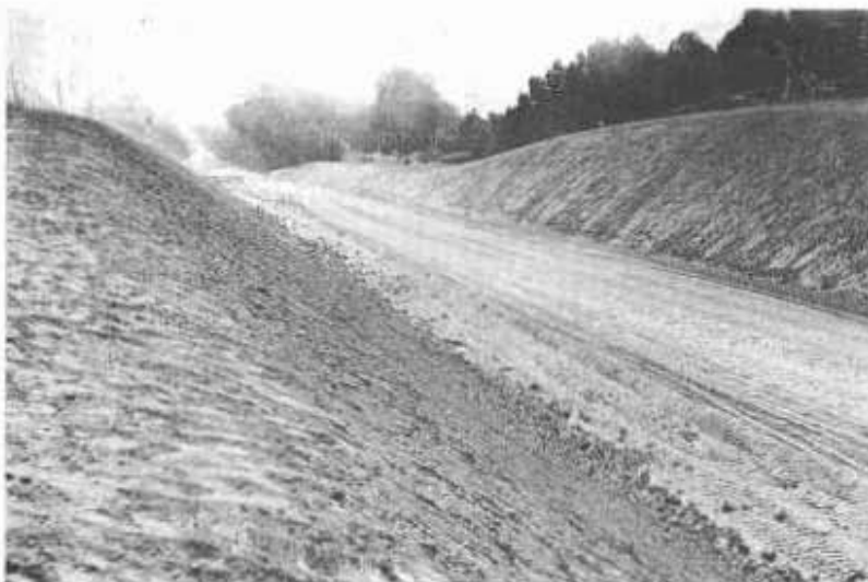
Cut slopes, 1½:1 that were blanketed with 6 inches of top soil as part of contract
