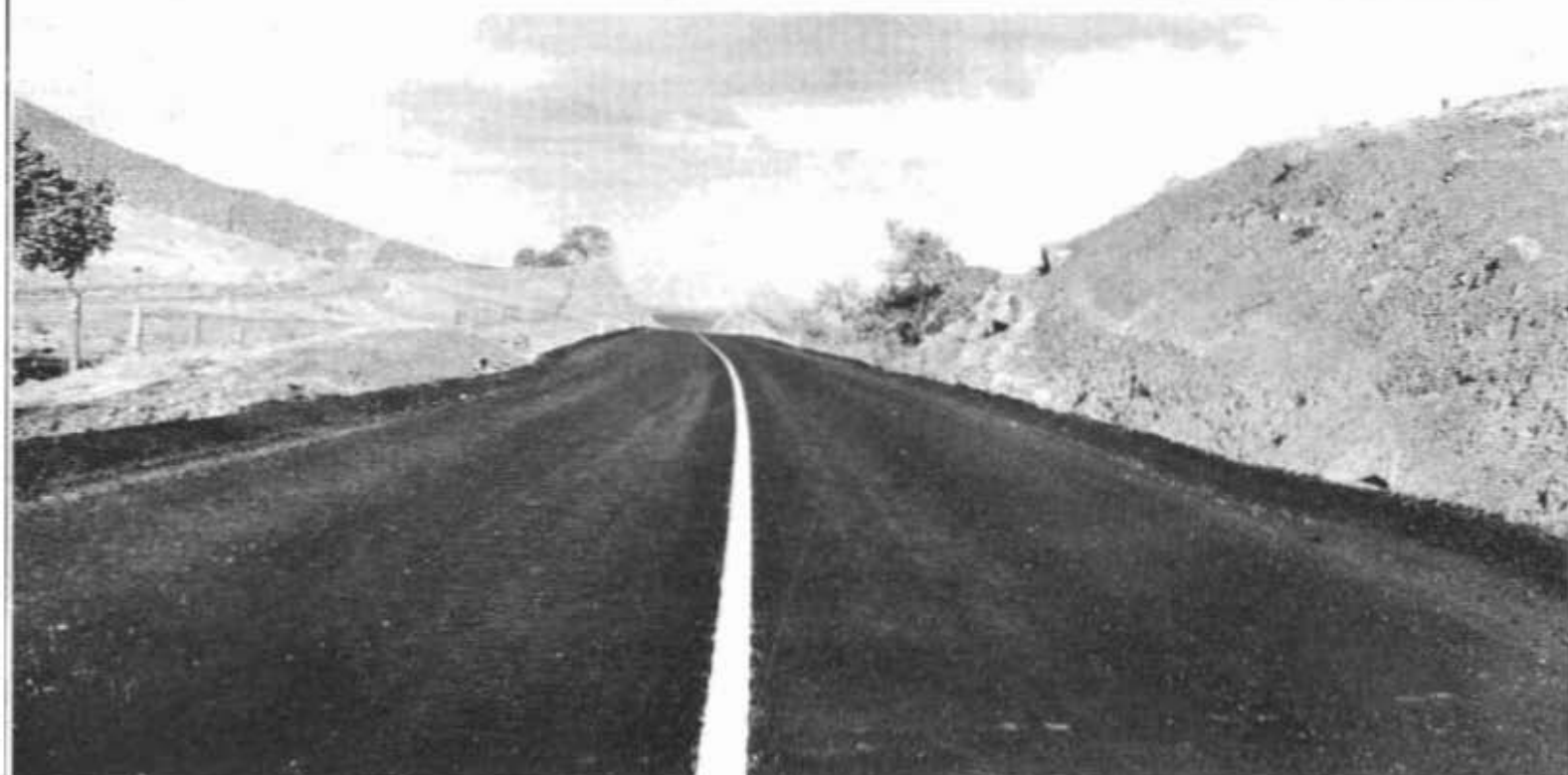
Section of new, wide two-lane highway with bituminous mix surfacing recently completed on Cholame lateral through Cottonwood Pass
