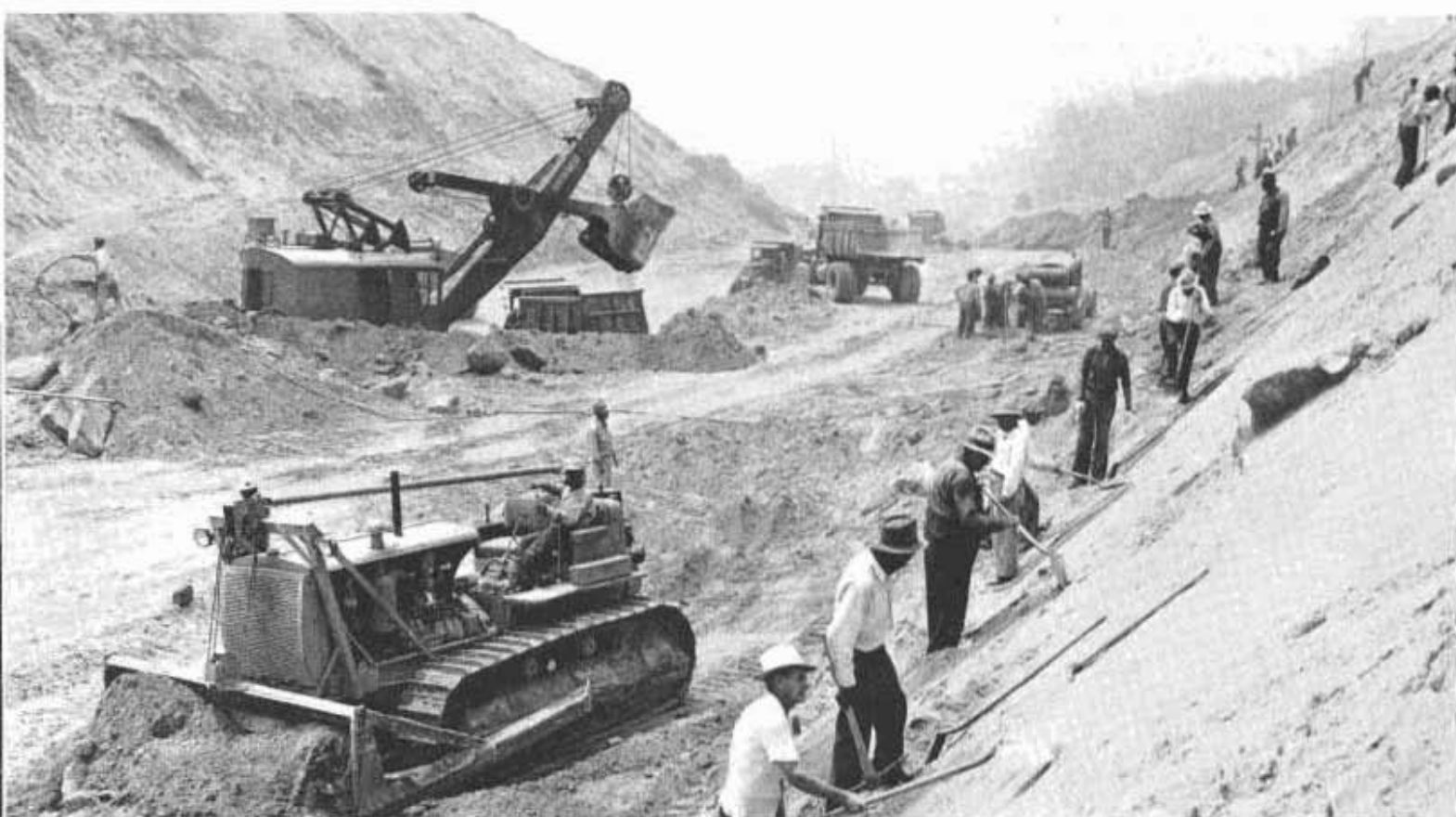
Big power shovels, tractors, bulldozers, trucks and some of 2,000 men engaged in building Arroyo Seco extension through Elysian Park
