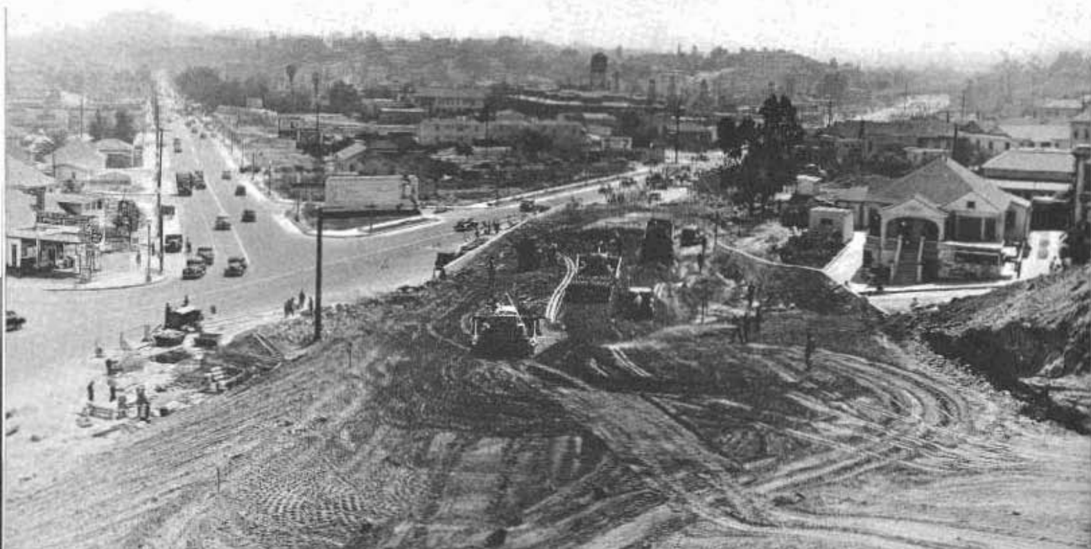
Extensive grading work and site of two overhead grade separation structures at intersection of Castelar and Figueroa Streets
