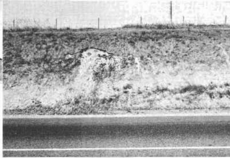
Gravel slope on which erosion was prevented by top soil cover damaged by pedestrians climbing up and down
