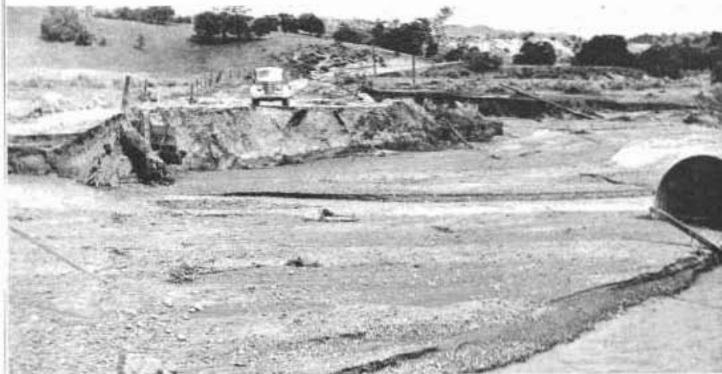
Realignment by-passes this washout of culvert and bridge
