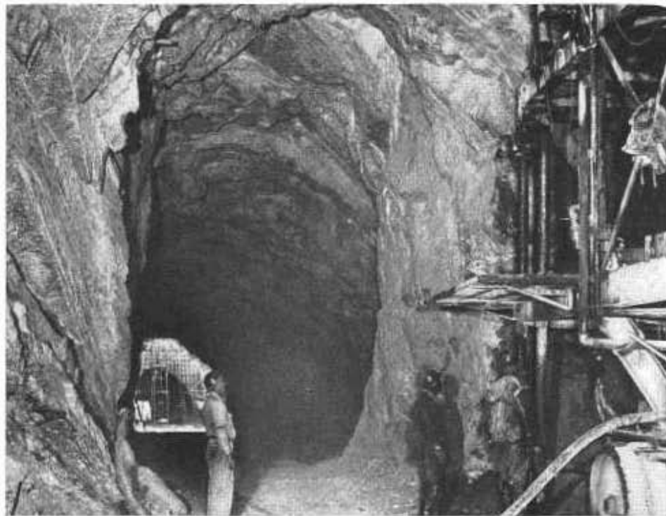
Equipment widening tunnel No. 1 bore. No. 2 bore entrance is seen in background
