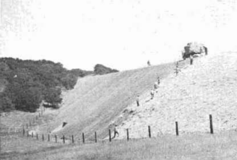
Fill slope treatment. Half of seed is sowed before straw is applied
