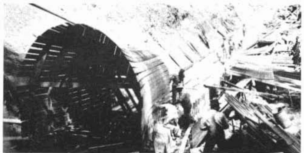
FIG. 20. Forms for throated entrance to concrete arch culvert. Note gradual flattening of grade towards outlet
