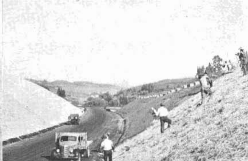
A closer view of strawing operation. Rate of application is 3 tons per acre
