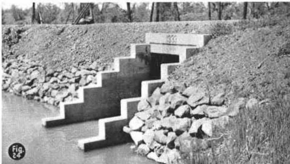
FIG. 24. Stepped "U" Type Endwall. Most inefficient type—not recommended except for cattlepass where drainage is a minor factor
