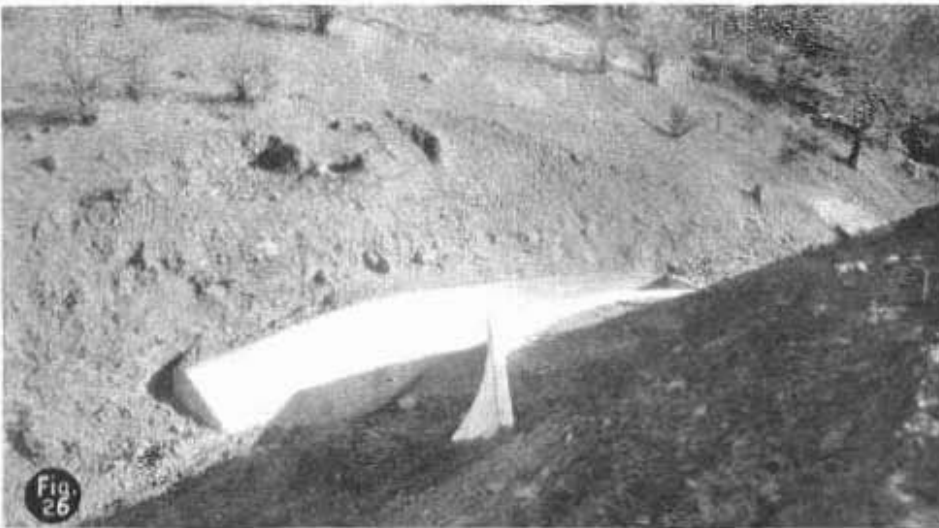
FIG. 26. Open lined training channel to concrete box culvert accelerating stream flow requiring minimum culvert section. Note warped wings
