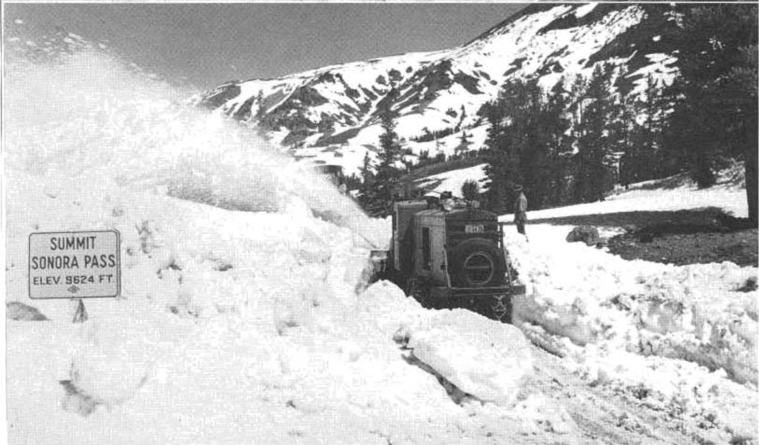
Snow was packed so hard on Sonora Pass Highway that it had to be dynamited before plows could work. Upper—Blowing Pack. Lower—Plow makes headway
