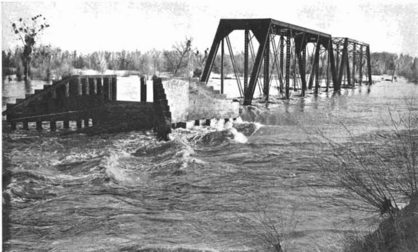
Portion of railroad bridge span damaged by February break of Feather River levee in Reclamation District 803
