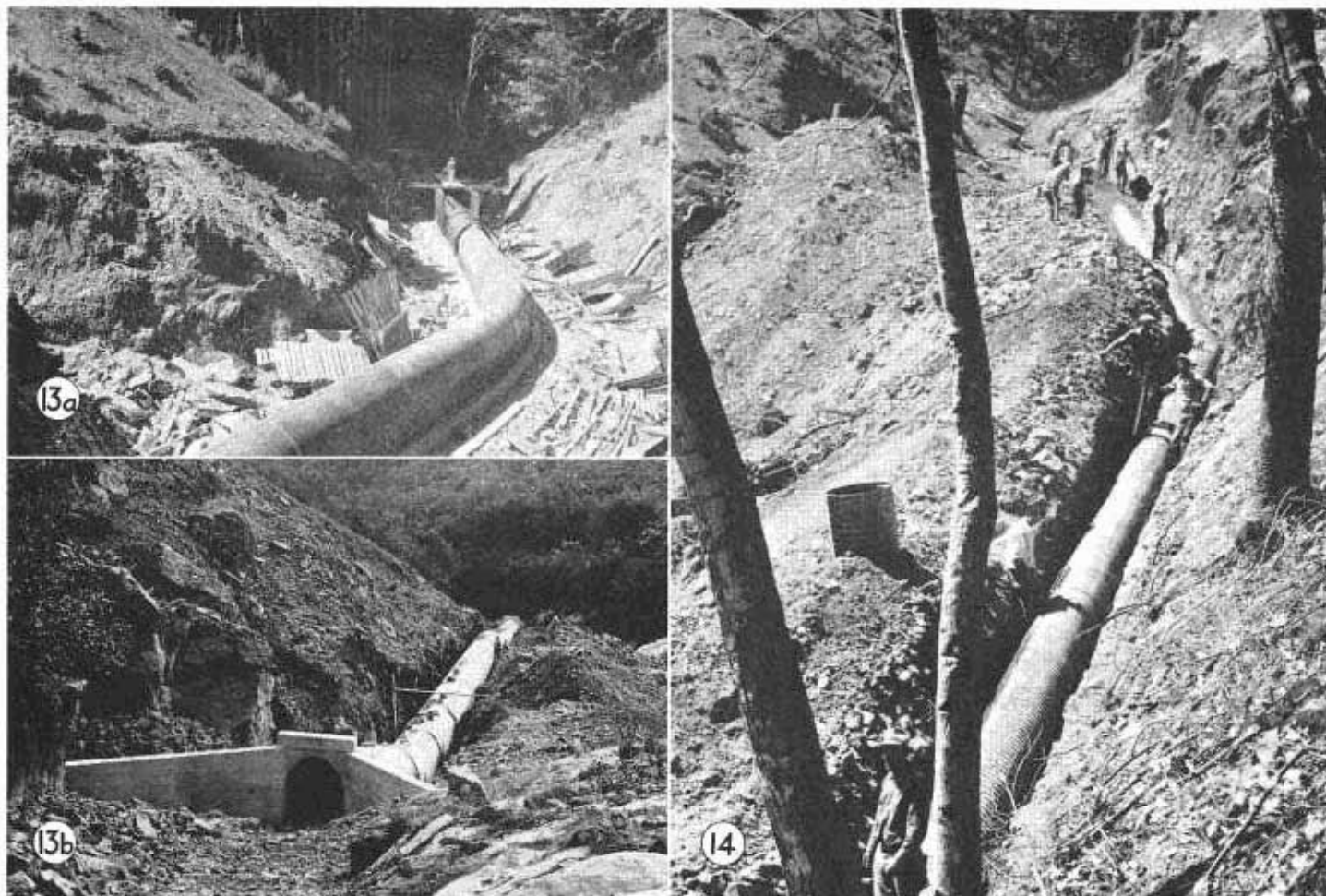
Figure 13a. Bottom Location—reinforced concrete arch on curved alignment and uniform gradient in bottom of ravine. Figure 13b. Bottom Location—reinforced concrete arch on straight alignment and broken gradient. Figure 14. Modified Bottom Location—corrugated metal pipe, with entrance in bottom of ravine and alignment following grade tour in sidehill trench, to an outlet well above and to one side of natural channel.
