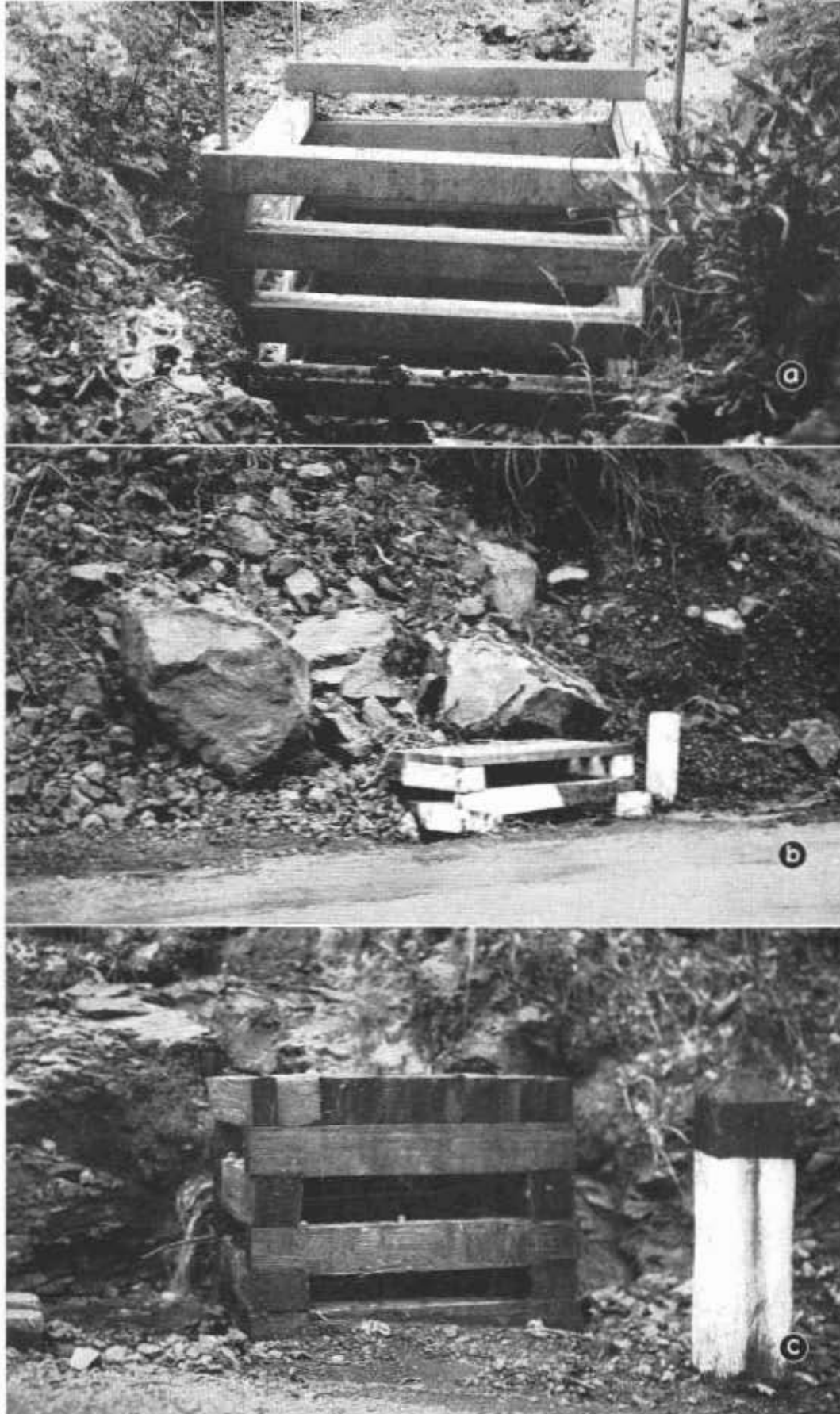
FIGURE 10. (a) Debris crib of reinforced concrete, with provision for extension placed over culvert entrance in small debris basin and commonly known as a "bear trap." (b) Timber debris crib installed over culvert entrance in roadway gutter. Note how debris has been prevented from blocking culvert entrance. (c) Debris crib of hewn timber, with a solid cover, placed over culvert entrance in roadway gutter
