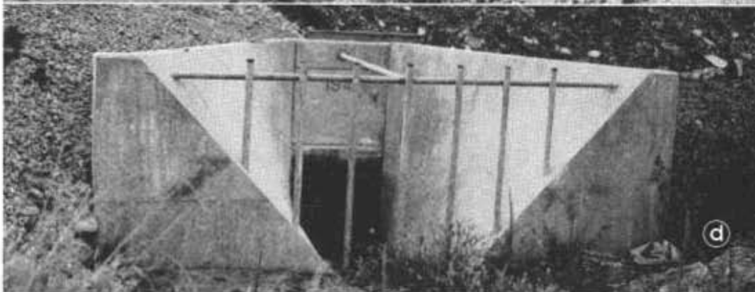
FIGURE 9. (a) Steel rail debris rack installed at end of wing walls to large reinforced concrete arch culvert. (b) Steel rail debris rack at end of wing walls to reinforced concrete arch culvert. (c) Steel rail debris rack placed in channel well above a culvert entrance. (d) Pipe debris rack at end of wing walls to reinforced concrete culvert. Note warped wing walls and curved-lip entrance
