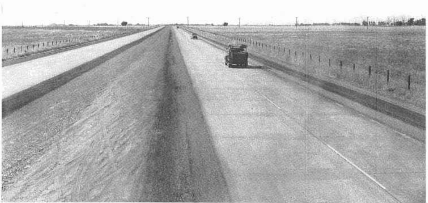
View of typical section of 4-lane divided highway on partially completed Davis-Dixon cut-off recently opened to traffic
