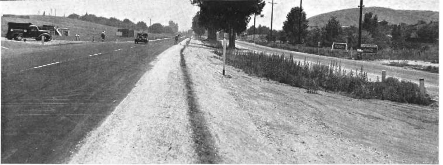
Four-lane divided highway East of Redlands. New construction for dual West bound traffic lanes on left. Existing highway on right
