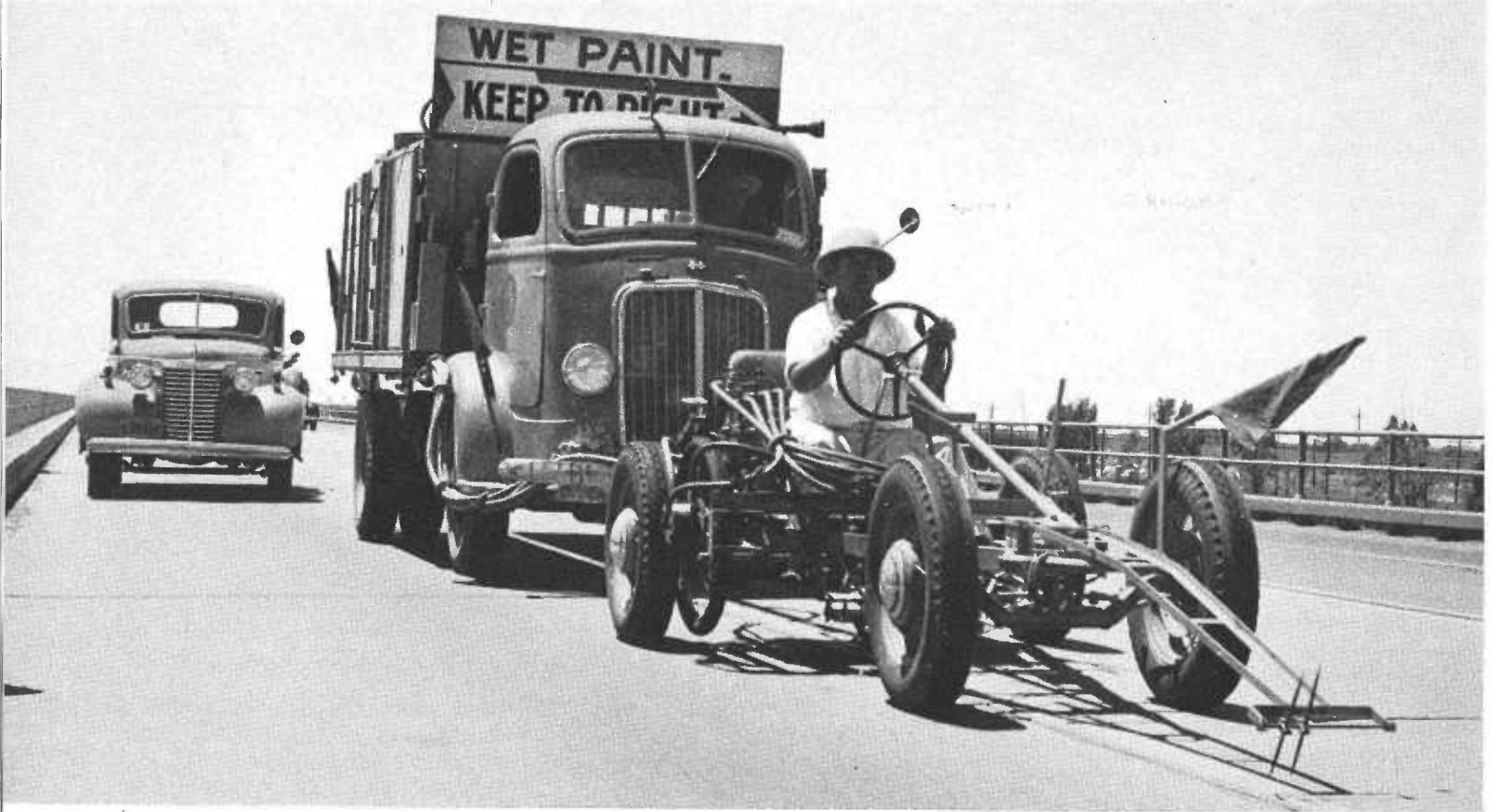
View of broken traffic line striping equipment in operation on State highway
