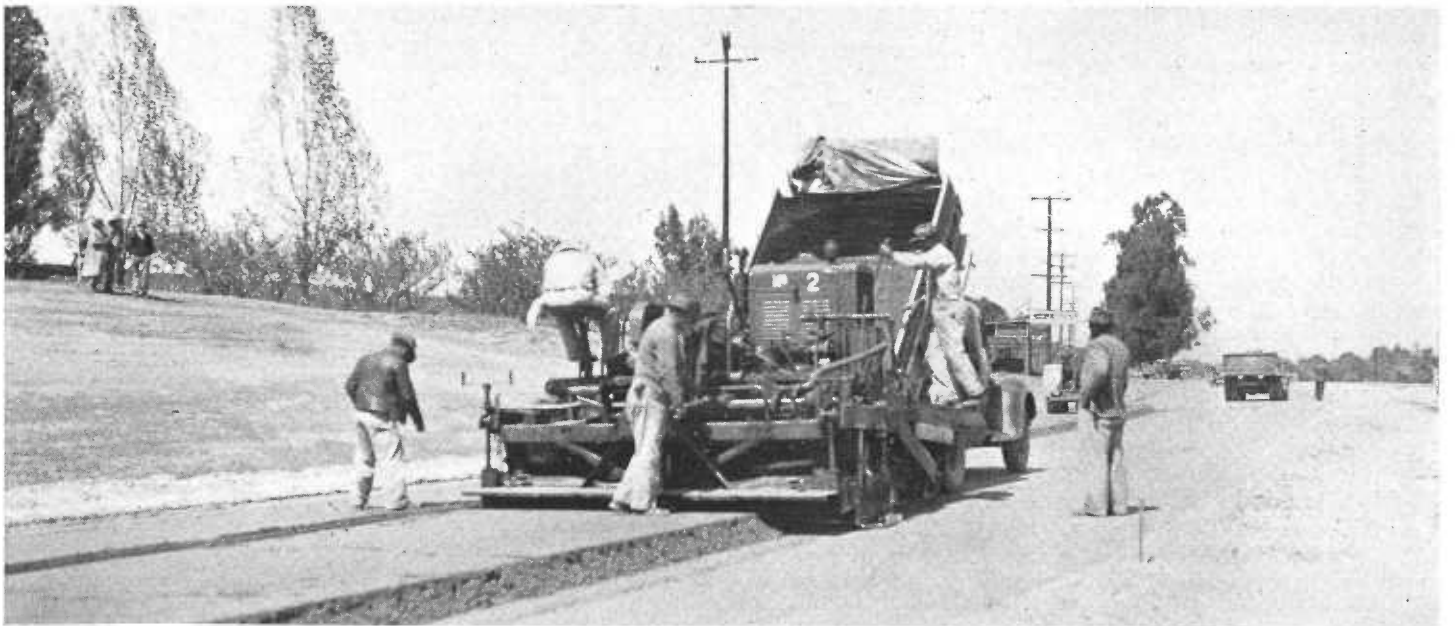
Spreading cement-treated base material with self-propelled mechanical spreading machine which pushes truck discharging material ahead of it
