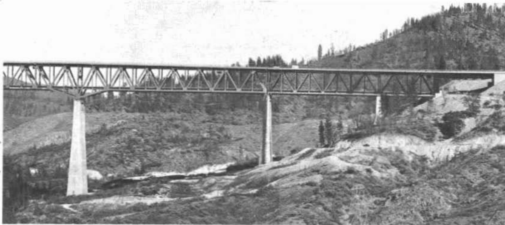
deck. It is 3,587 feet long and 500 feet above river bed. Two of its piers are the highest concrete piers in the world, exceeding bridge is seen in background
