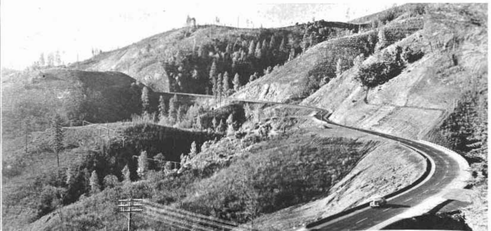
Relocated section of U. S. 99 around Shasta Dam Lake site near O'Brien Summit, photographed before road was opened
