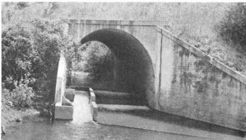
FIG. 36. Rattlesnake Creek, with drop inside the arch culvert. Note fish ladder at left
