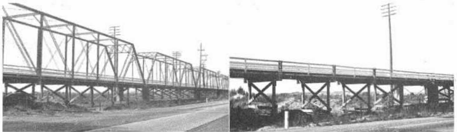
Before and after views of steel truss bridge across old channel of Santa Maria River in Santa Barbara County from which steel above floor was salvaged.
