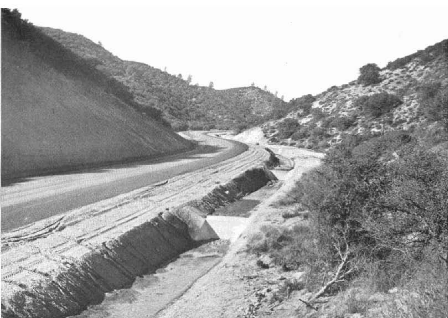
Section of Bradley-King City highway showing concrete check dams along creek channel to prevent excessive erosion in canyon section
