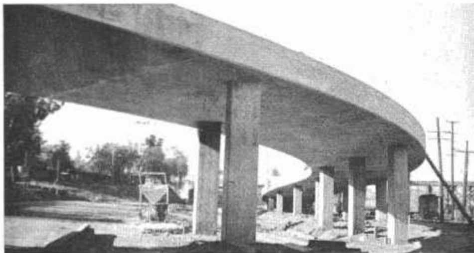
Pomeroy Street overhead, a companion traffic interchange structure to Soto Street, shows a twisting reverse curve alignment
