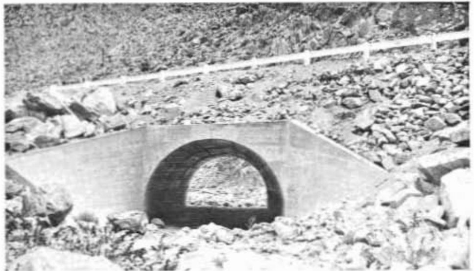
FIG. 54. Myers Creek culvert on State Highway in Imperial County, a flat arch under a low fill
