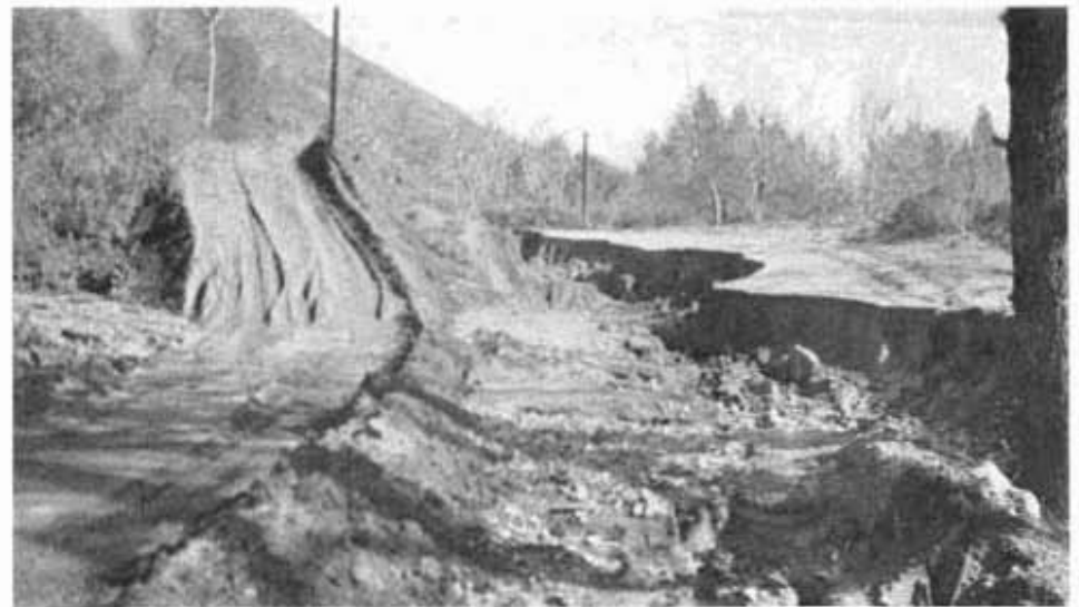
State Highway 188 washed out; temporary detour near Crestline, San Bernardino County
