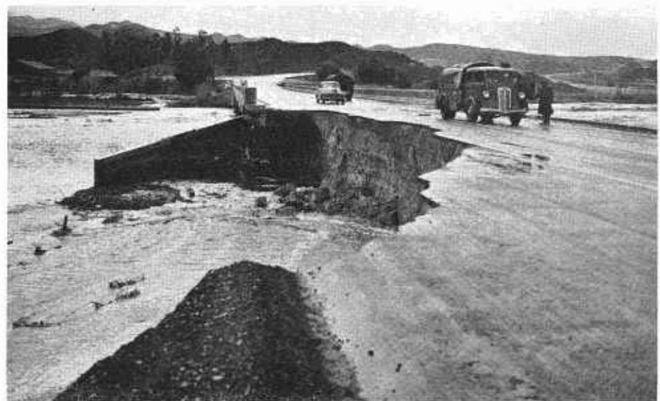
One lane of approach to bridge over Santa Clara River on U. S. 6 damaged
