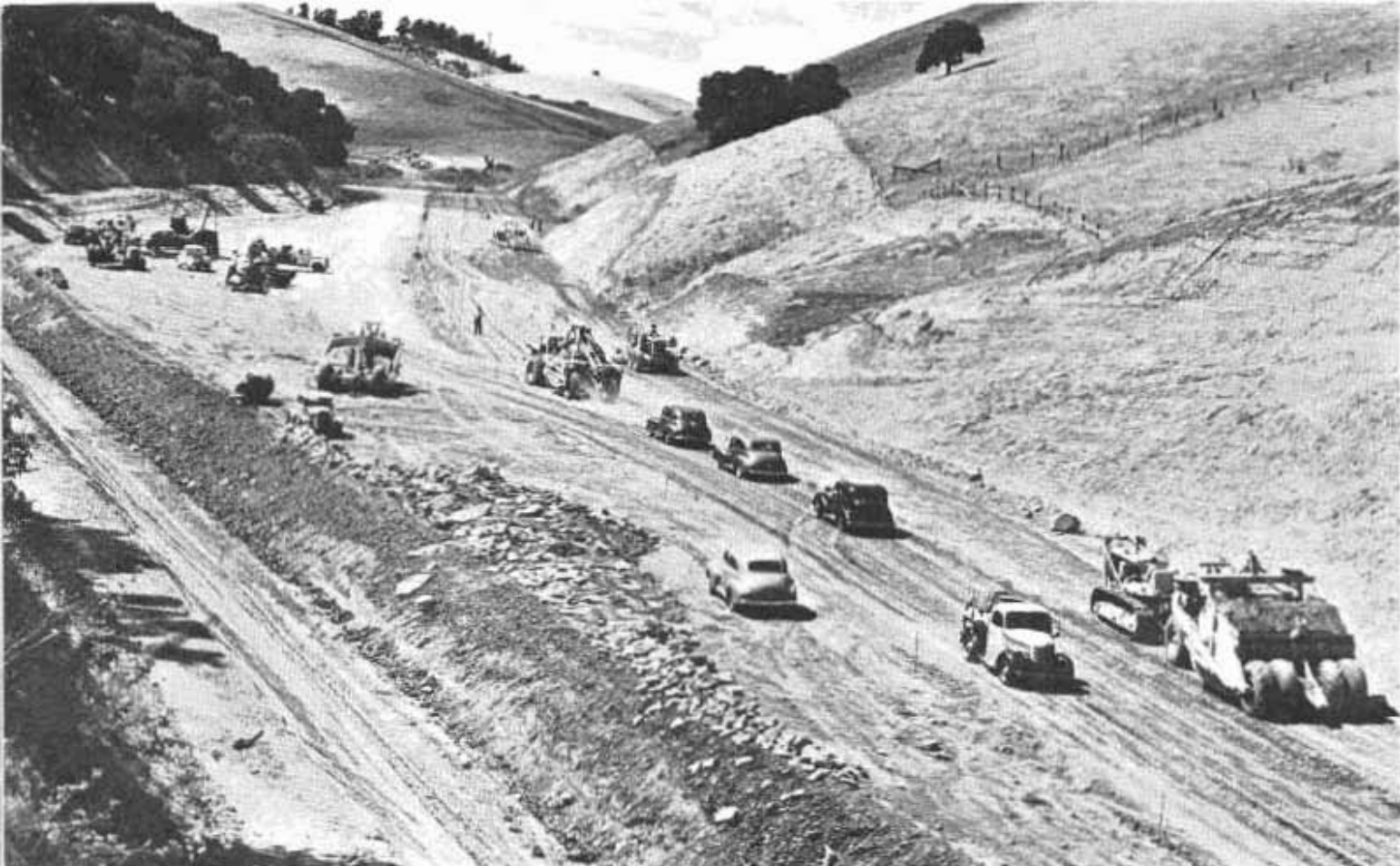
Equipment working on new grade of relocated Franklin Canyon highway. Channel change of Franklin Creek below level of old road shown at left
