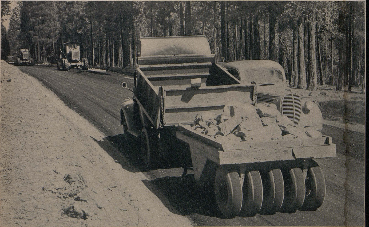
At top—Easy going on 40,000 cubic yard cut. Bottom—Spreading and compacting surface with graders and rubber-tired roller
