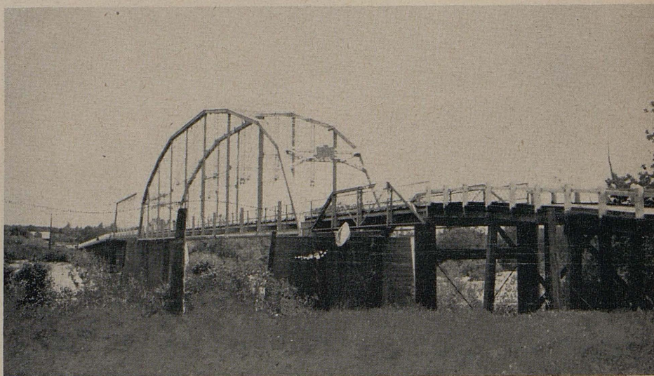
A "must" bridge which is weak and structurally unsound
