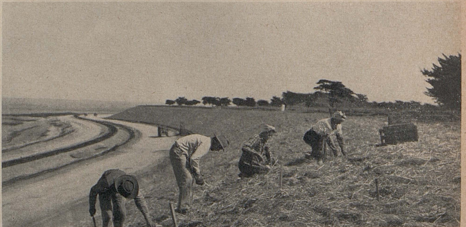
Planting Ice Plant cuttings through straw along top and bottom of slope
