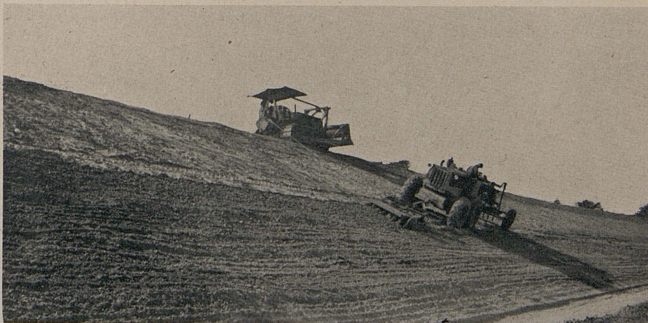
Disking 2:1 cut slope prior to spreading top soil. Grader below is cabled to tractor above
