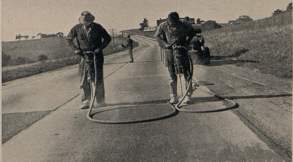
Upper—Mud jacking equipment in operation. Forcing cement treated loam under paving. Lower—Drilling holes preparatory to mud jacking operations
