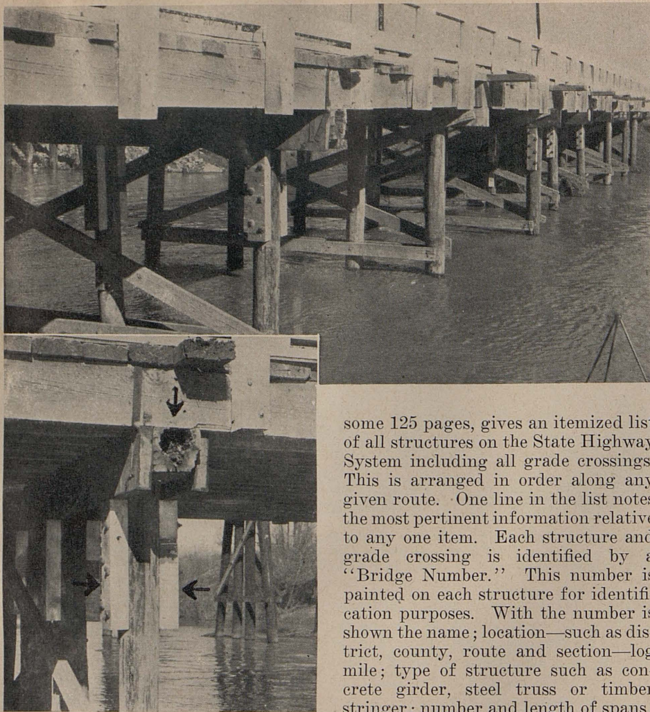
Pictures show typical repairs to a timber trestle scheduled for replacement in fall of 1943. Arrows point to rotted stringer and 6- by 8-inch corbels or supports bolted to the sides of the piles. The corbels support 4- by 16-inch stringers used to reinforce the cap
