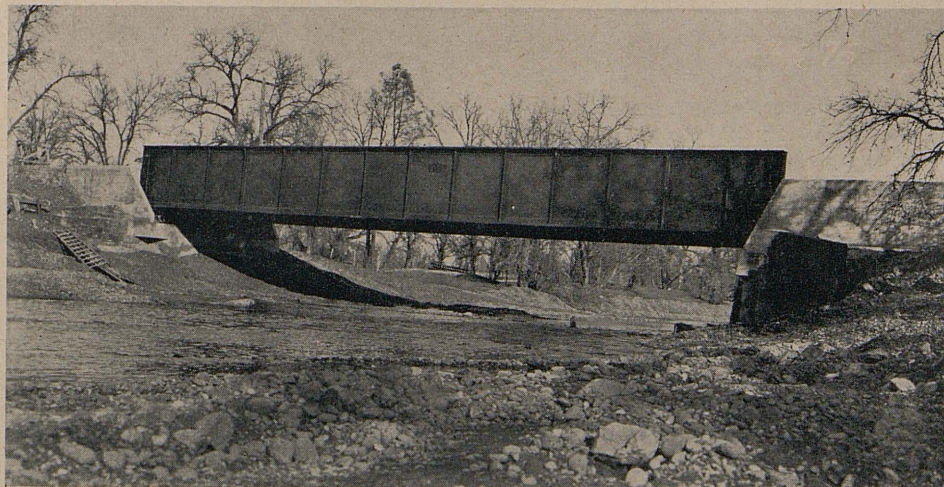
Single span steel railroad bridge State was able to buy for replacement
