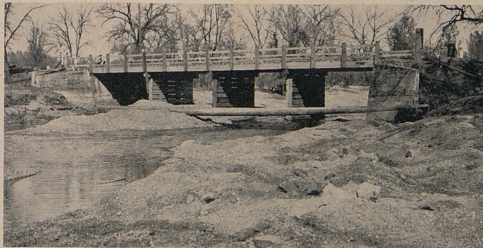
Old four-span timber bridge across Oak Run Creek that had to be replaced
