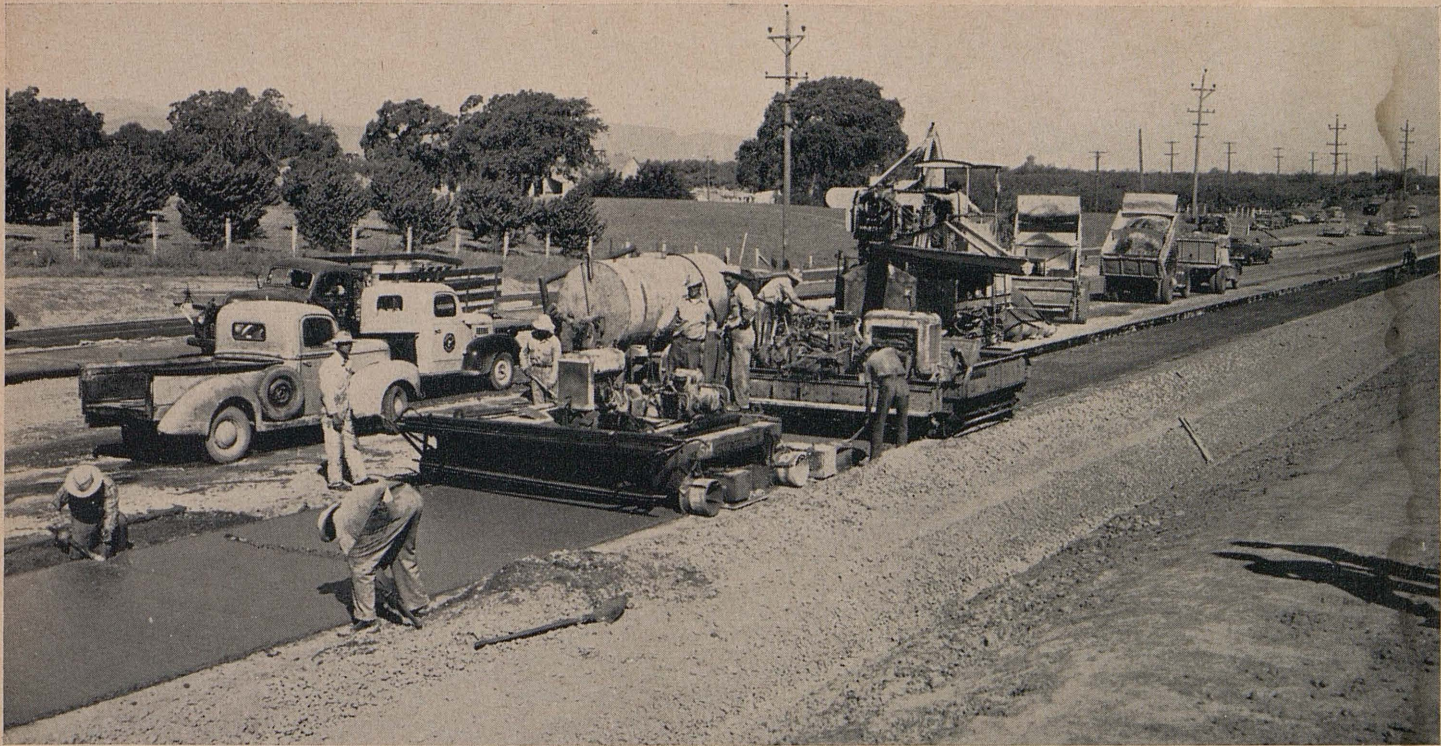
This photograph shows paving operations in progress on Vallejo-Napa highway between Napa Wye and Napa City
