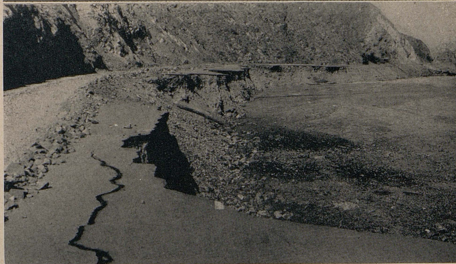
Top—Tractor at work removing deposit from roadway one mile northeast of Homestead, Route 23 in Kern County. Oil truck and trailer in background. Center—Bulldozer working to uncover roadbed on State Route 23 clearing three feet of silt from Pine Tree Dip Bottom—Entire roadway lost. Only portion of center line stripe remaining on this section of State Route 23
