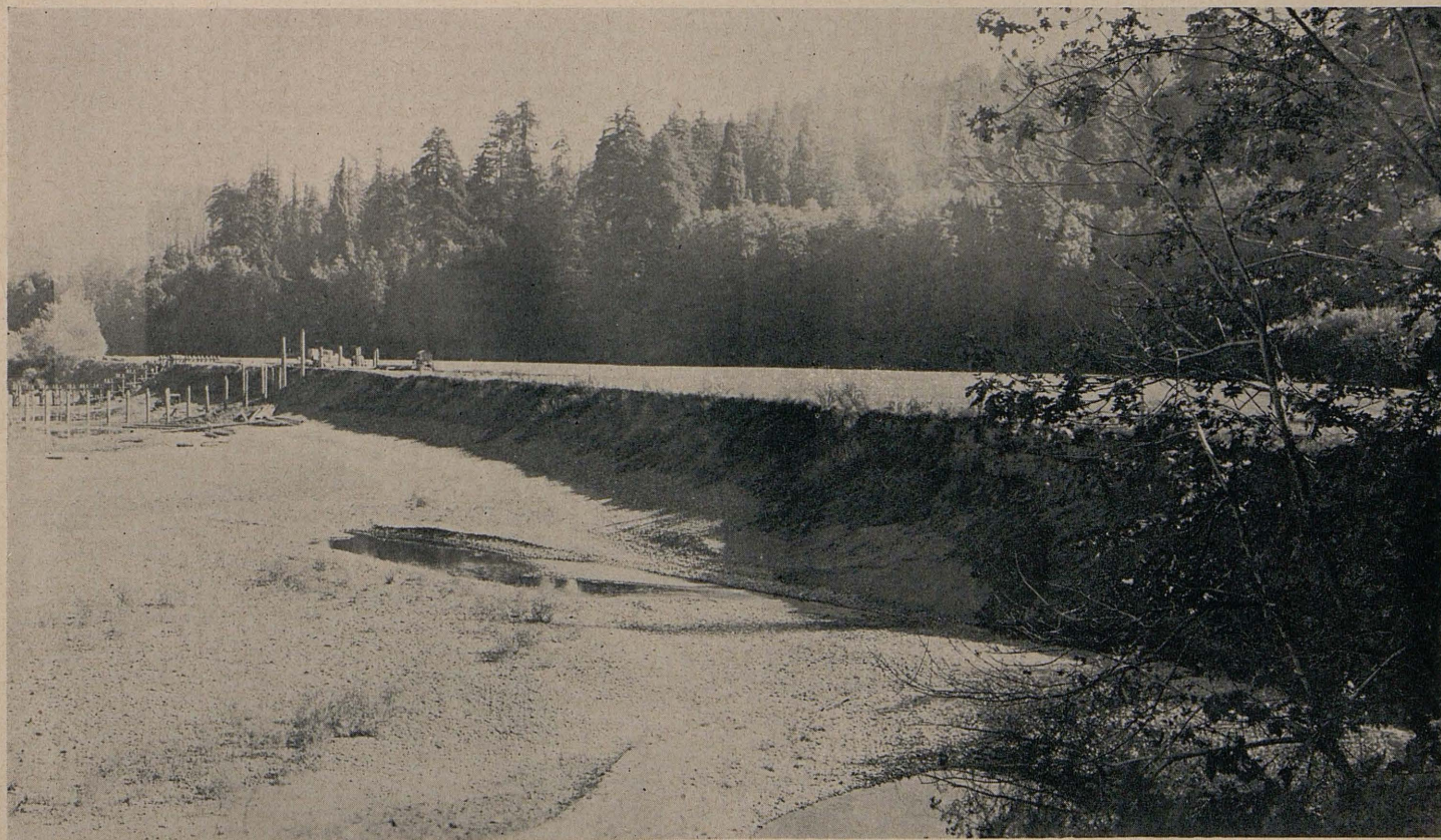
View of site of jetty installation just upstream from Shively Bluff. Piles in the two upstream jetties have been driven. Chad Creek enters the river in the right foreground
