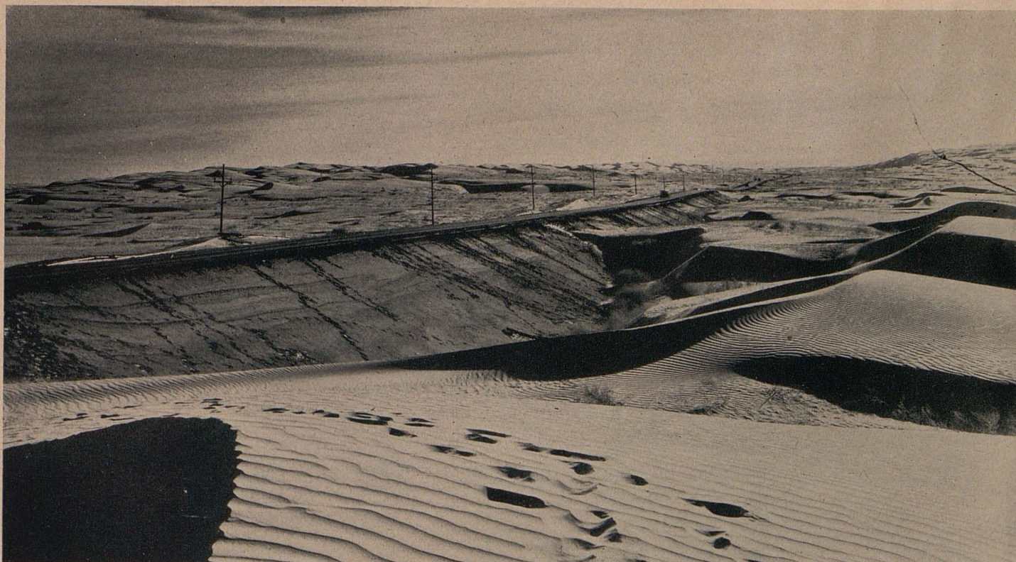
And this is a view of a section of the modern highway which replaced the old plank road. Slopes in right foreground are constructed to prevent sand drifting over the traveled way
