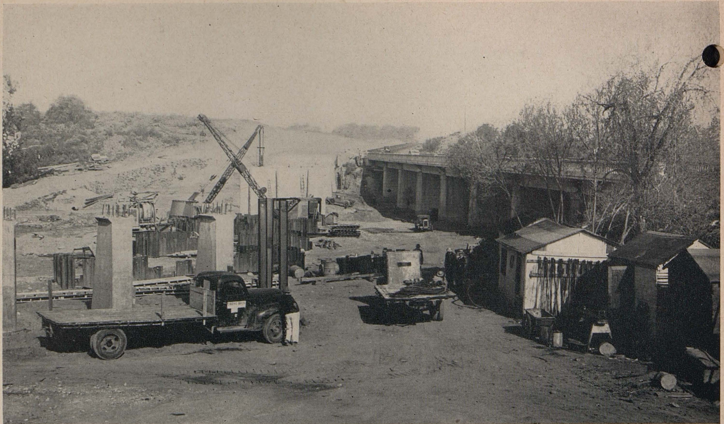
Construction scene at site of new bridge for southbound traffic across San Mateo Creek
