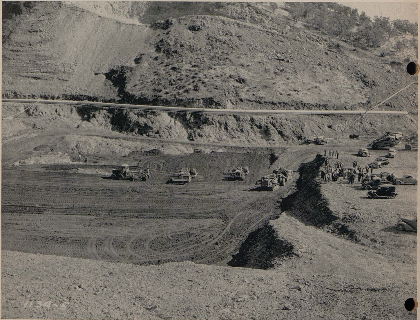
Heavy construction equipment is excavating tons of material on site of Rector Canyon Dam, Napa County
