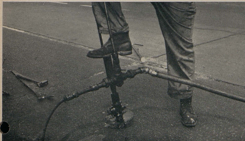
Supplemental or auxiliary nozzle and three-way valve on full circulating system
