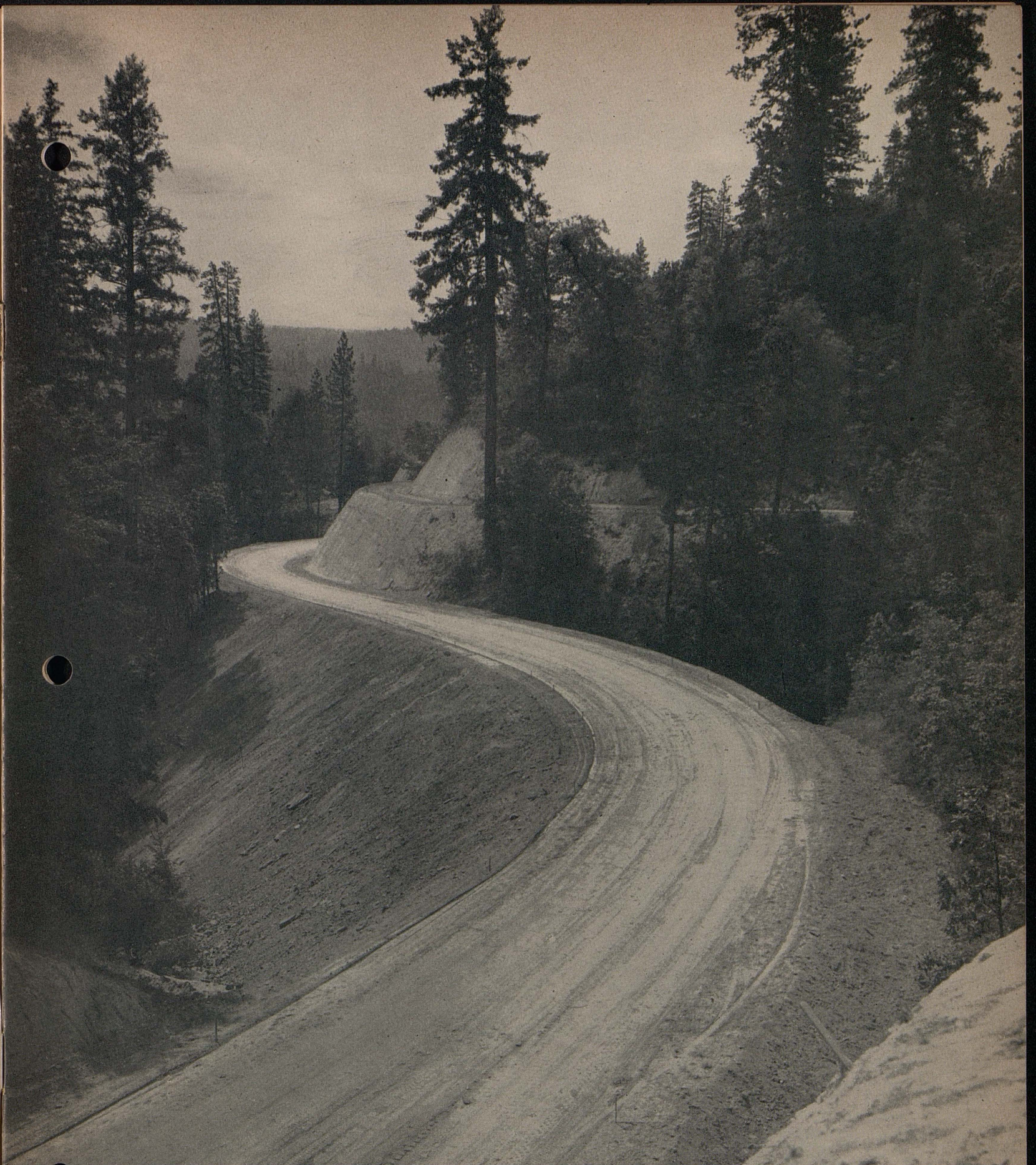
Section of new highway between Nevada City and Downieville—old route follows hazardous curve above new road
