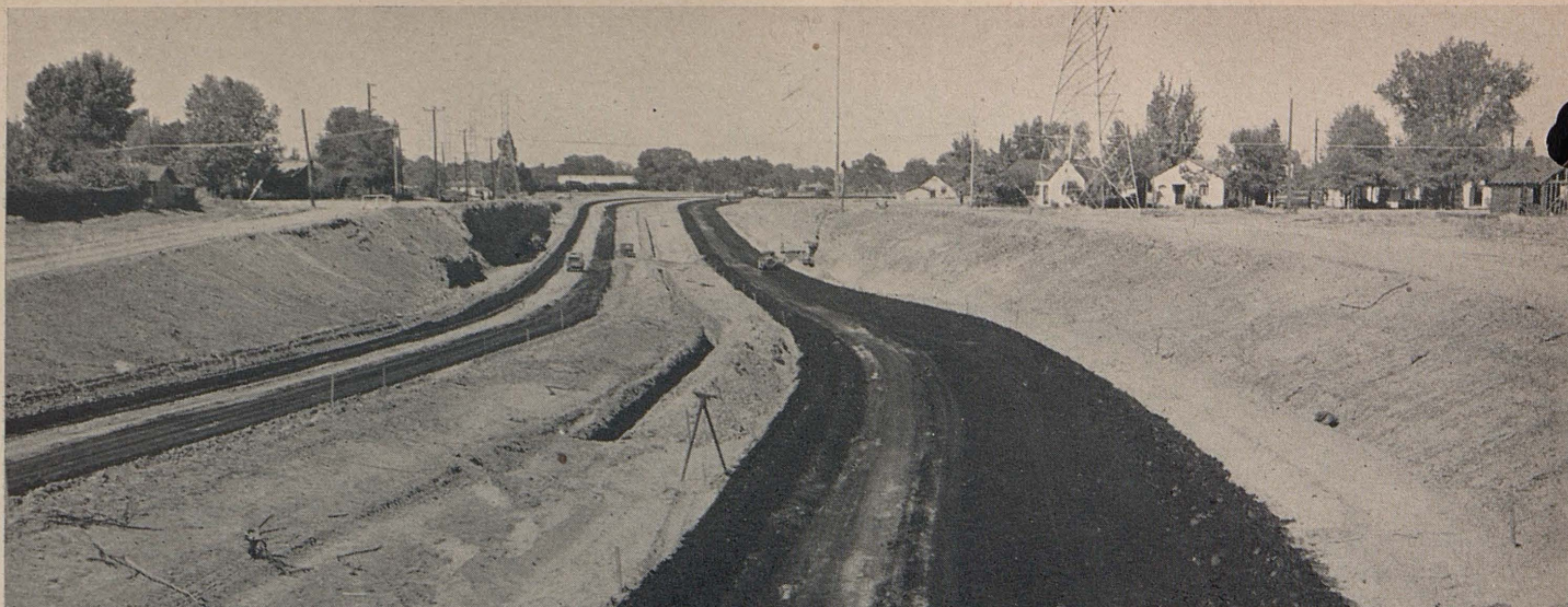
Depressed section under Marconi Avenue structure, which is not yet under construction
