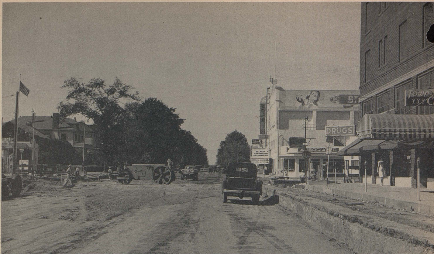
Compacting original ground prior to placing imported borrow on realigned approach to new Feather River Bridge. Scene is at Fifth and E Streets in Marysville
