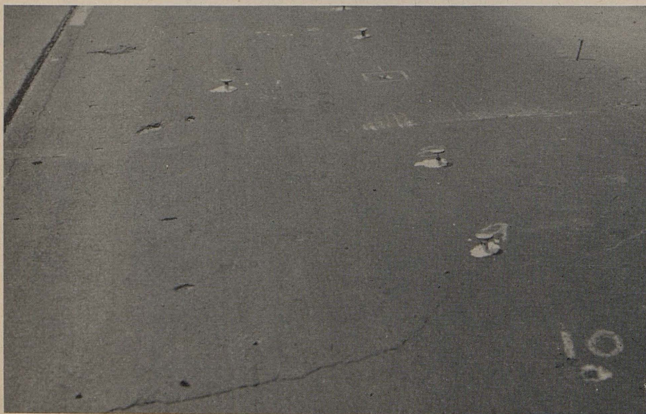
Test holes with thermometer inserted to determine flow of asphalt under pavement
