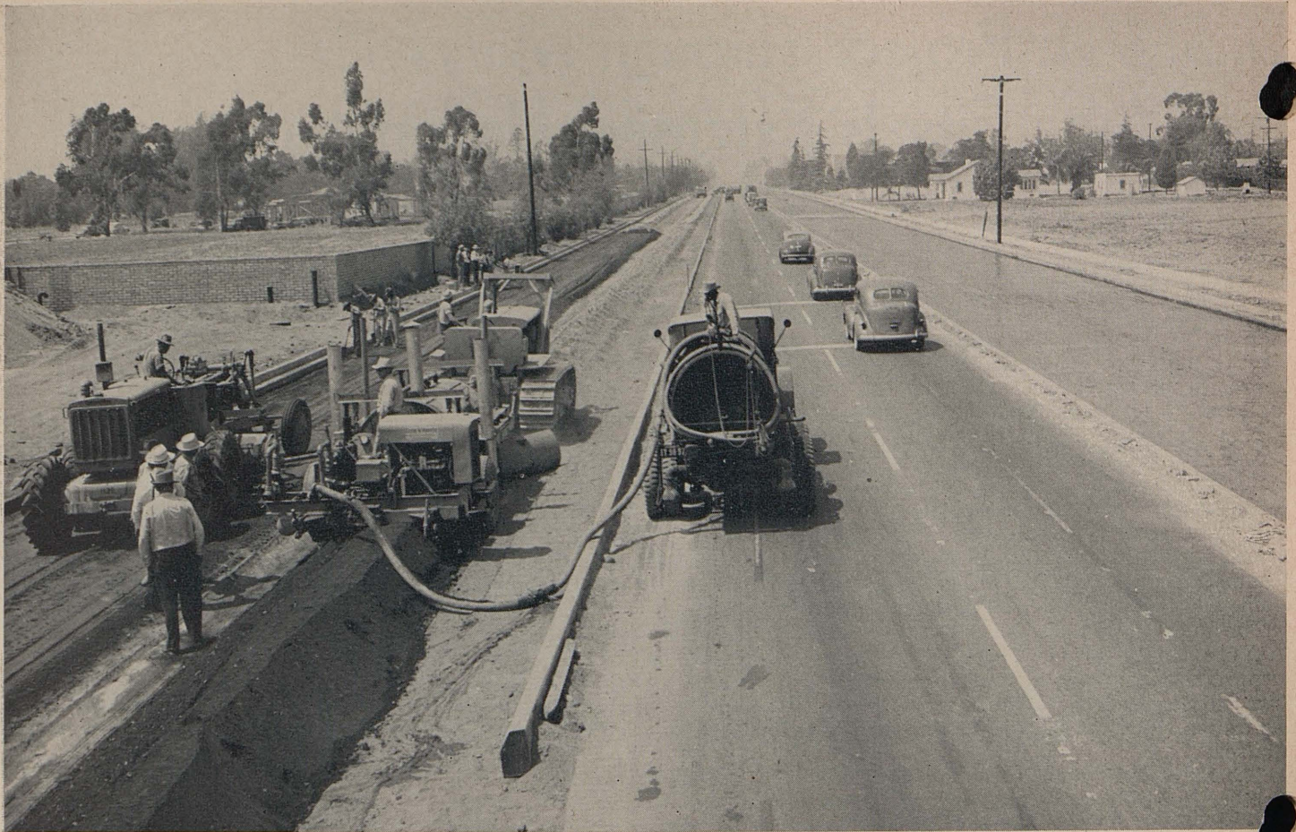
Cement treated base on Rosemead Boulevard had been completed on roadway to the right and seal coat applied when this construction picture was taken
