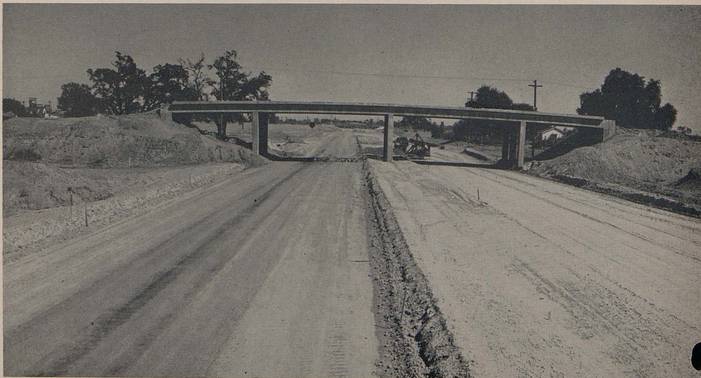
Looking eastward along the freeway with the Canterbury Road overcrossing in foreground and Deadman Slough structure in distance
