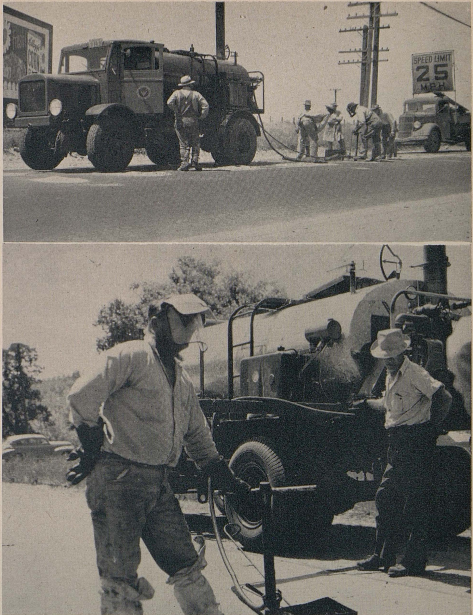
Two views of 900-gallon asphalt tank built by Headquarters Shops for asphalt subsealing
